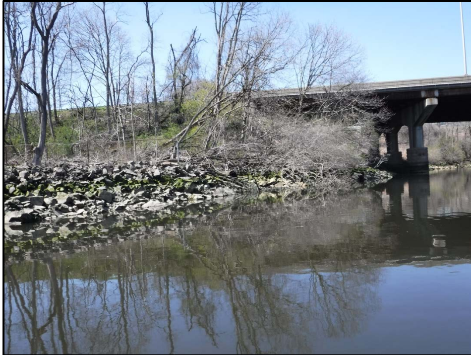
Photo No. 39: Dumped riprap along Interstate 91, looking northwest, photo taken April 14, 2016.
