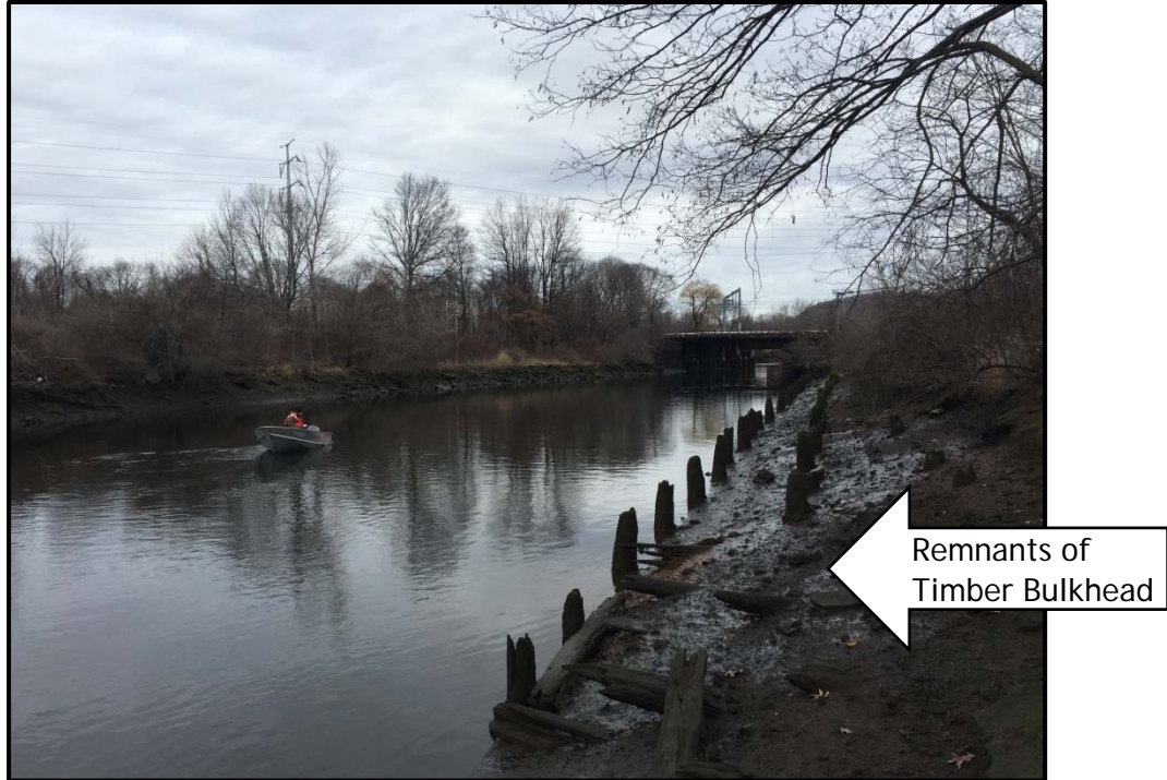
Photo No. 27: Remnants of a timber bulkhead along Radiall, looking north, photo taken February 4, 2016.
