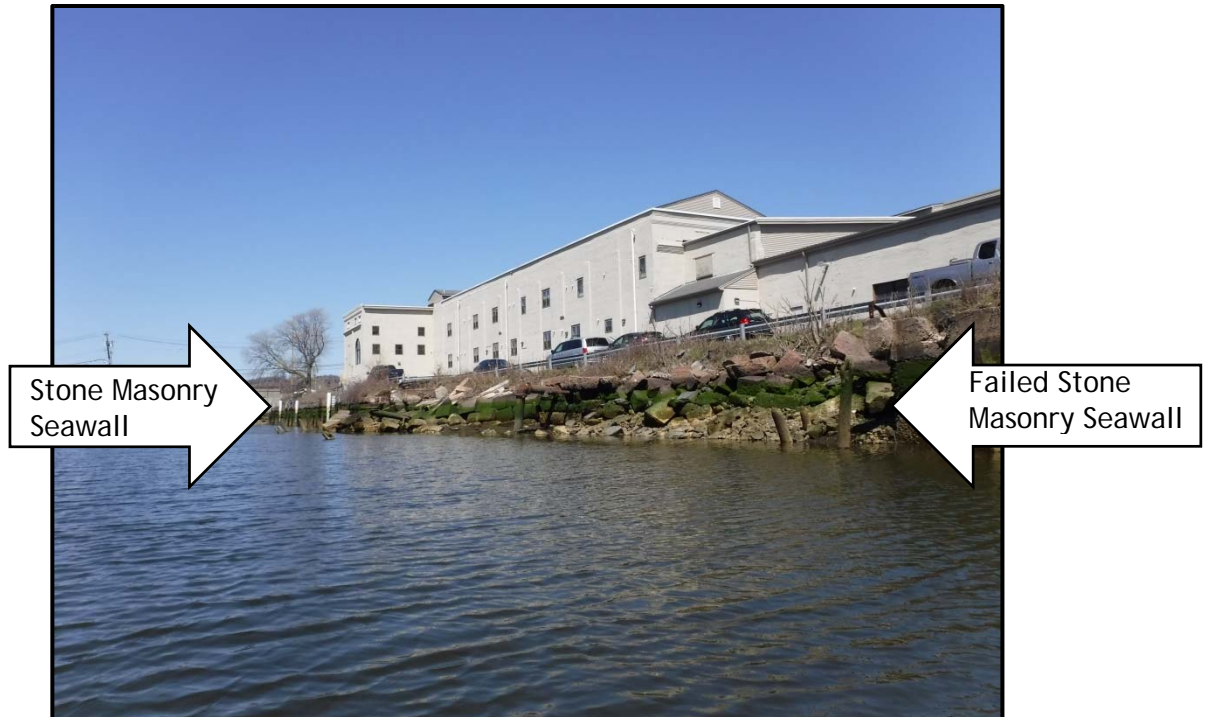
Photo No. 15: Stone masonry seawall along the Powerhouse Building, looking northeast, photo taken April 14, 2016.
