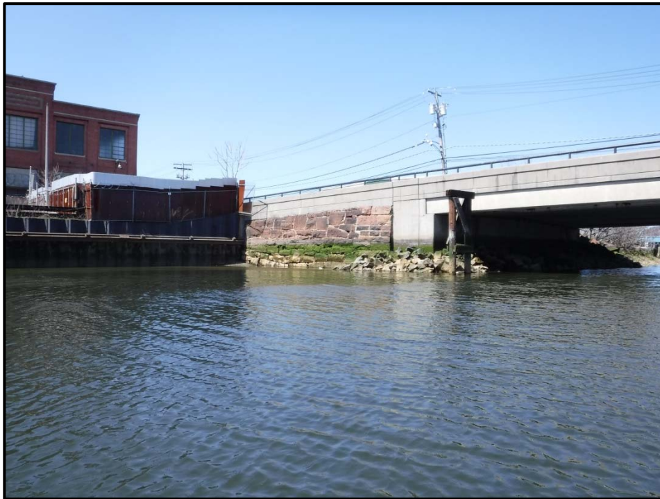
Photo No. 24: Grand Avenue stone masonry seawall, looking northwest, photo taken April 14, 2016.
