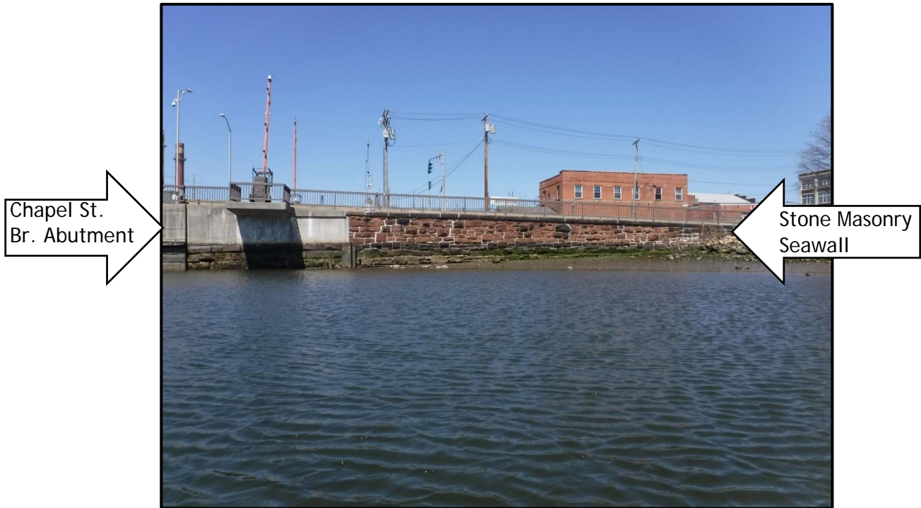
Photo No. 5: Chapel Street stone masonry seawall, looking north, photo taken April 14, 2016.
