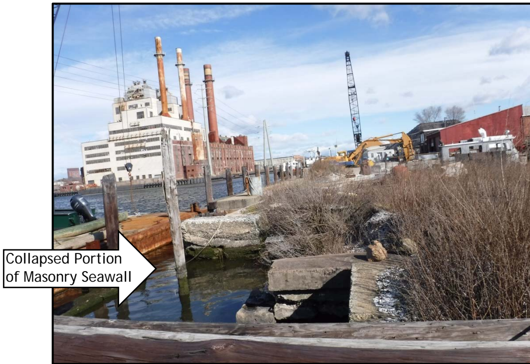
Photo No. 8: Stone masonry seawall along Hillard Bloom Shellfish, Inc., looking north, photo taken March 18, 2016.
