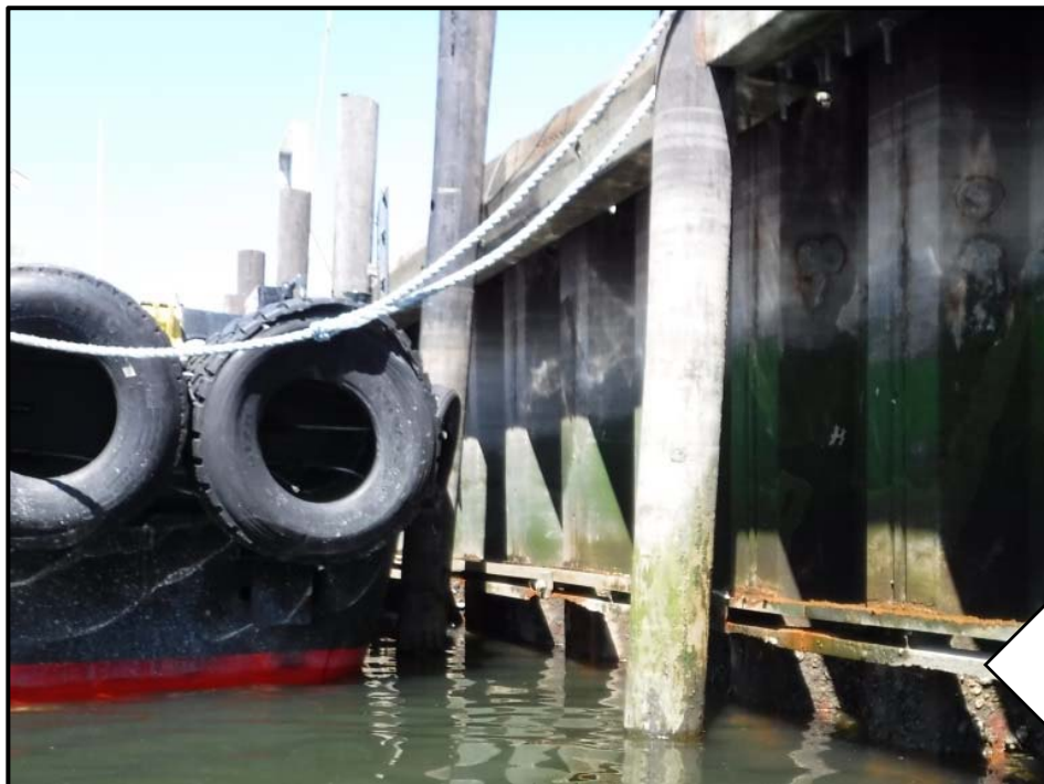
Photo No. 10: Steel sheet pile bulkhead along New NRB #3 Corp., looking northeast, photo taken April 14, 2016.
