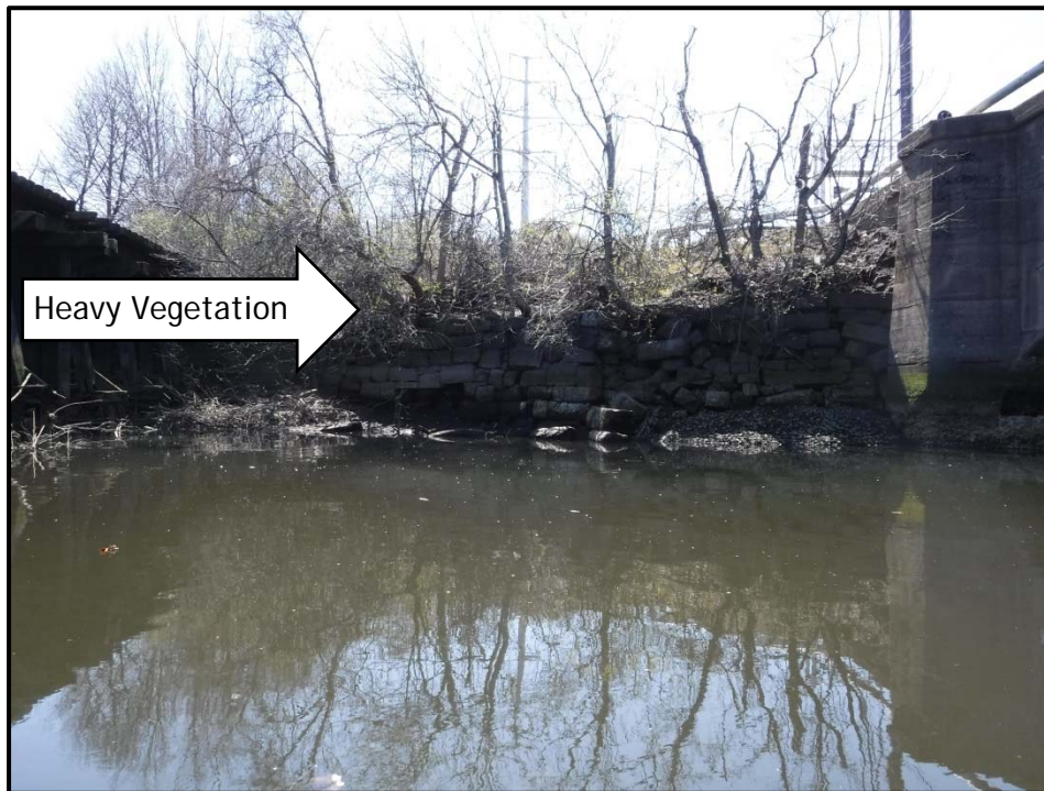
Photo No. 34: Stone masonry seawall between the abandoned and active rail crossings, looking west, photo taken April 14, 2016.
