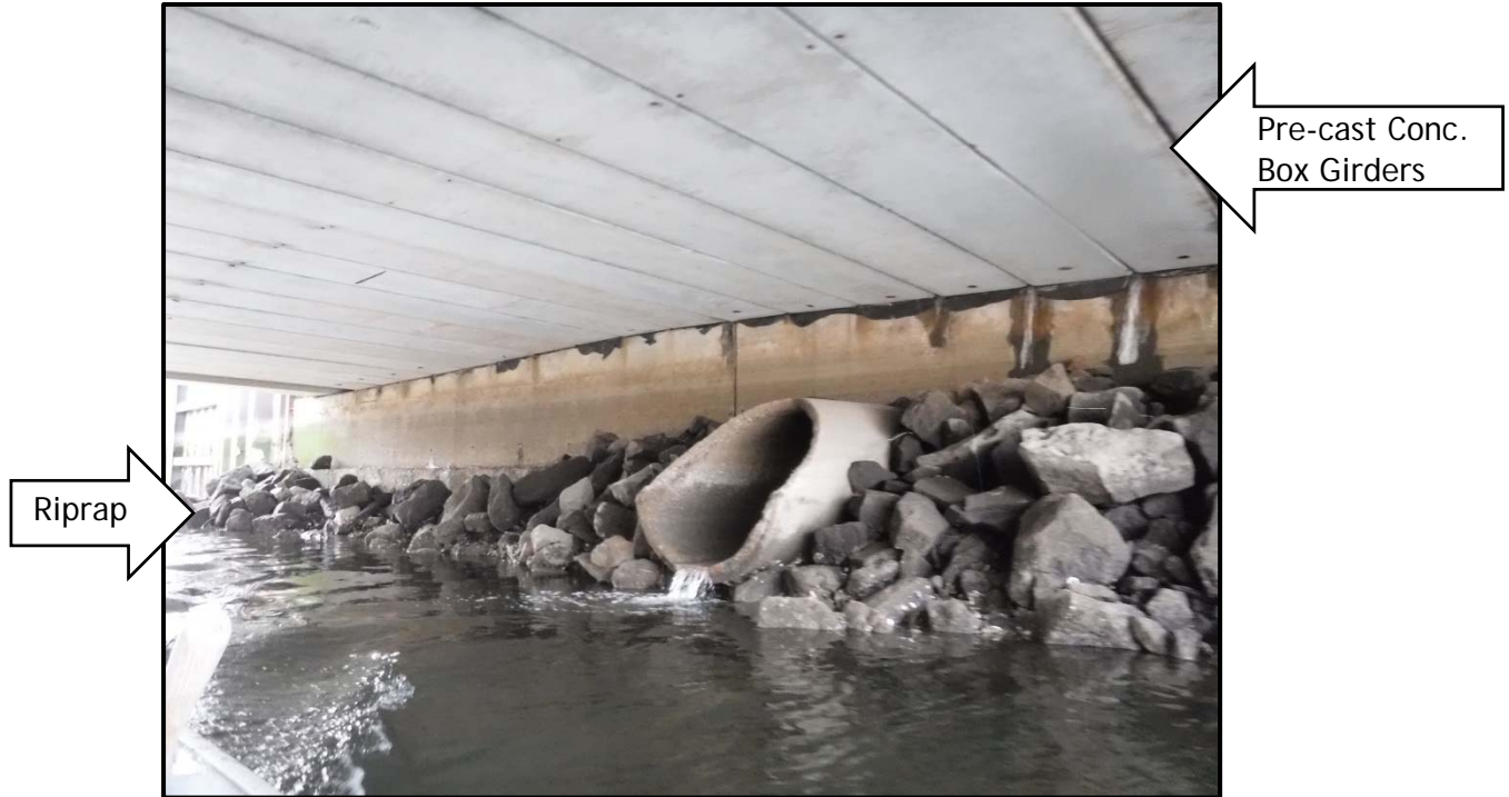
Photo No. 25: Grand Avenue Bridge over the West Branch of the Mill River, looking west, photo taken February 19, 2016.
