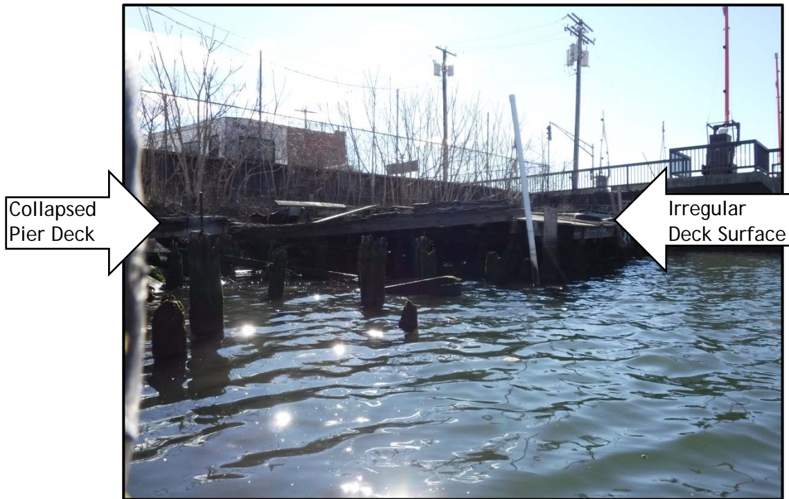
Photo No. 6: Fixed timber pier along 299 Chapel Street, looking southeast, photo taken March 18, 2016.
