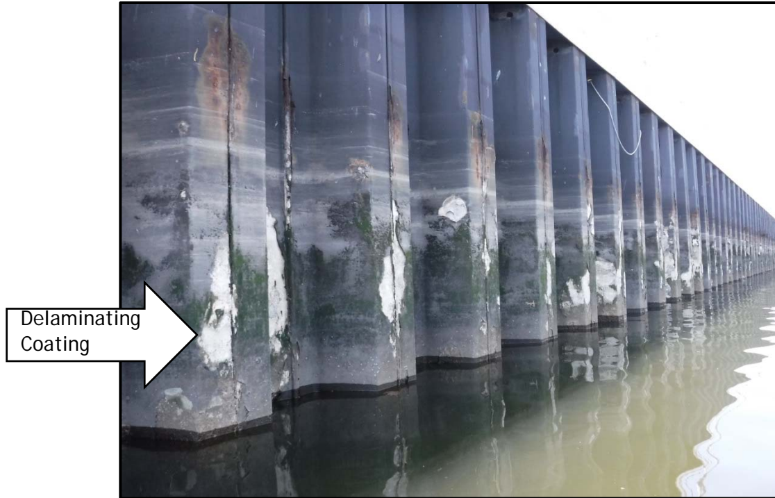
Photo No. 21: Steel sheet pile bulkhead along UL Grand Avenue Substation, looking northwest, photo taken April 14, 2016.
