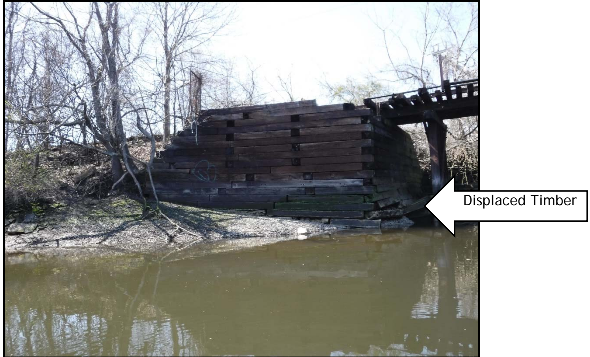
Photo No. 33: West timber abutment of abandoned rail crossing, looking northwest, photo taken February 19, 2016.
