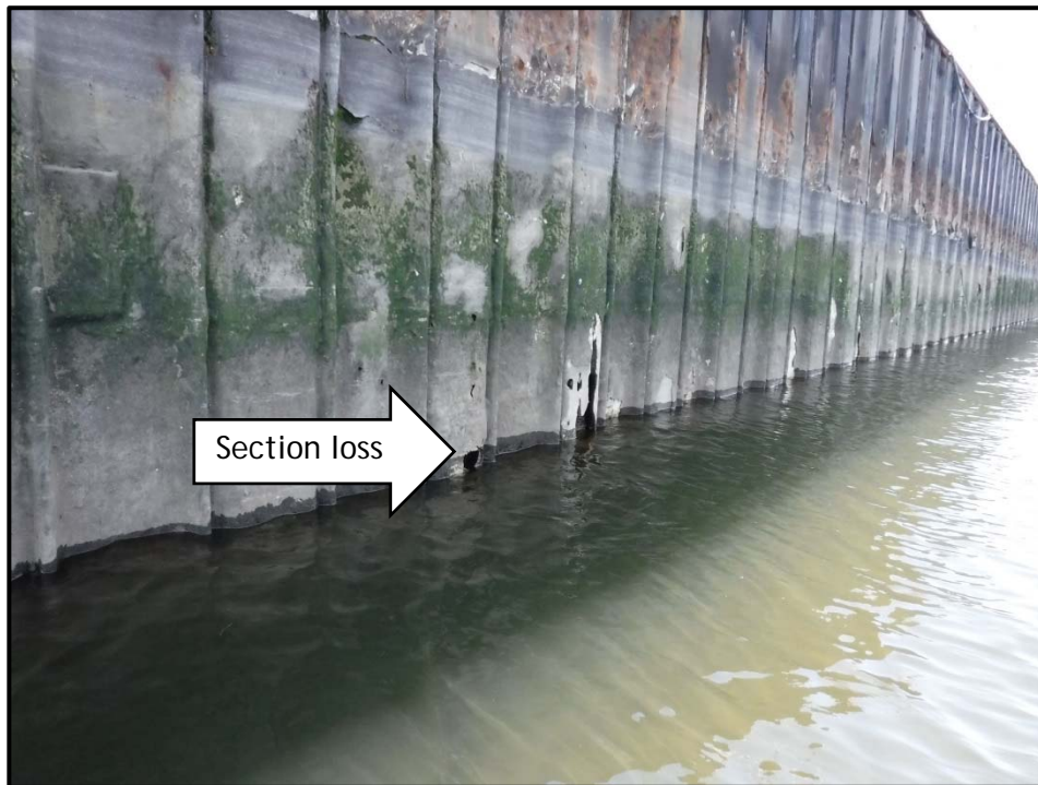
Photo No. 22: Section loss in steel sheet pile bulkhead along UL Grand Avenue Substation, looking northwest, photo taken April 14, 2016.
