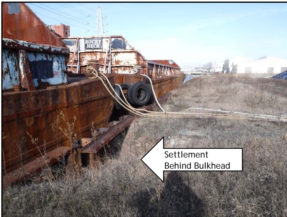
Photo No. 12: Steel sheet pile bulkhead along Gateway Terminal, looking north, photo taken January 8, 2016.
