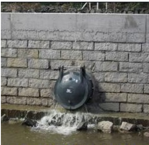
Stormwater Flap Gate
