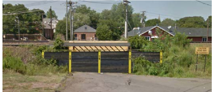
Manually Deployed Floodgate
