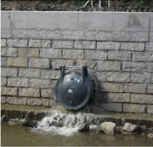
Stormwater Flap Gate
