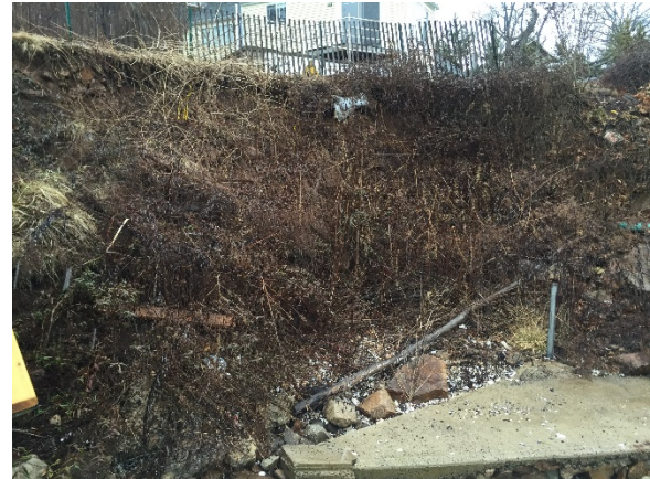
Eroding bank at eastern end of site
