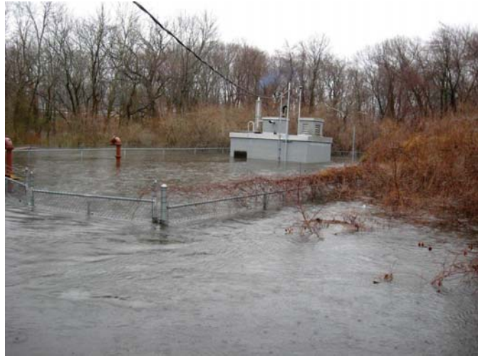
A flooded pump-station in Warwick, RI, 2010 Photo: Janine Burke
