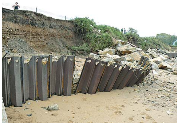
Collapsed seawall below Linden Ave Image: Pam Johnson/The Sound
