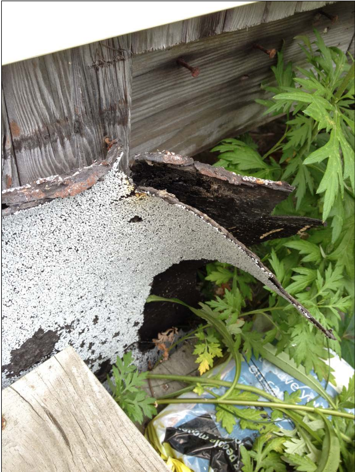
Exterior between stair case and house – rolled roofing used as siding (bottom layer) (All Black Layer)
