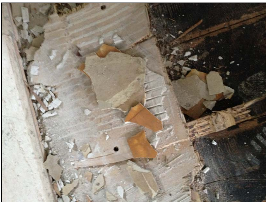
Hall in front of bathroom – scrap floor tile (vinyl)
