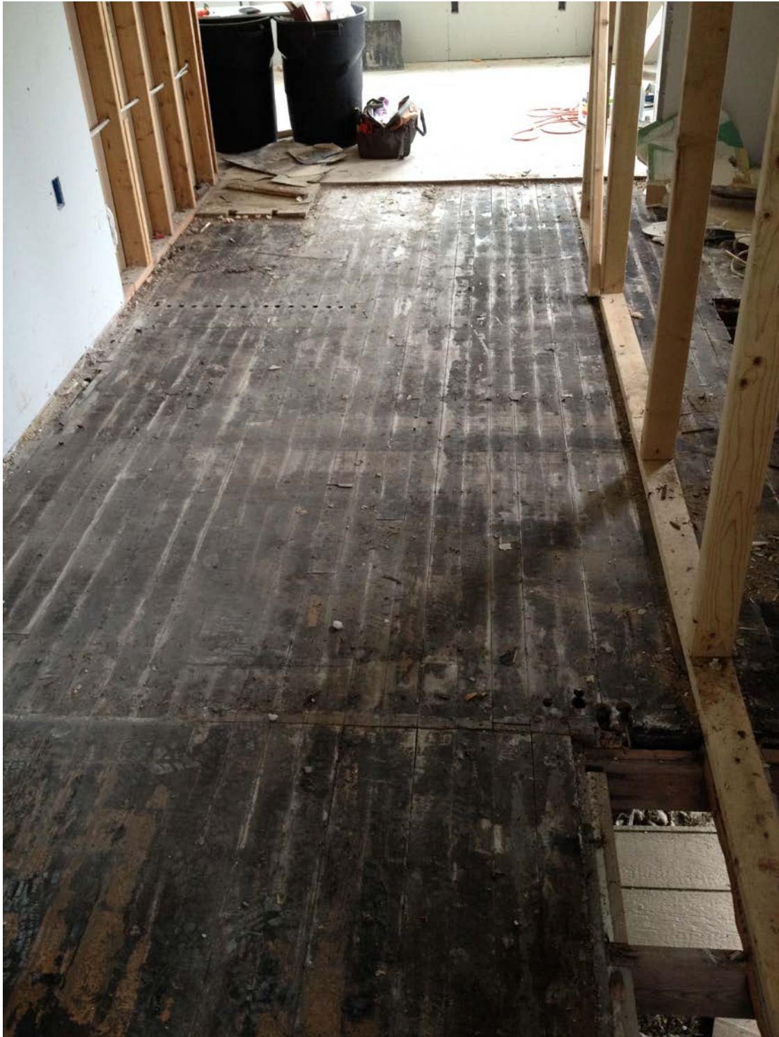
PCB-04 (Tar paper on kitchen floor) Also located on washer/dryer room floor and in hallway in front of the bathroom and bedroom with a closet.
