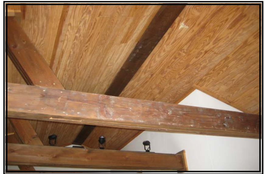
Photograph 8 Possible mold on untreated beams of ground floor
