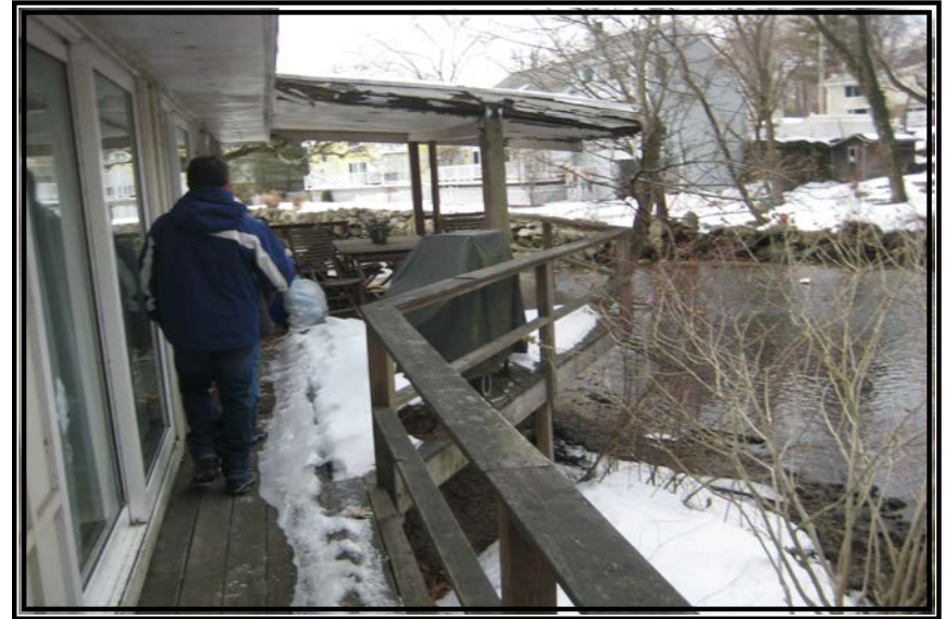
Photograph 2 Deck overhanging watercourse
