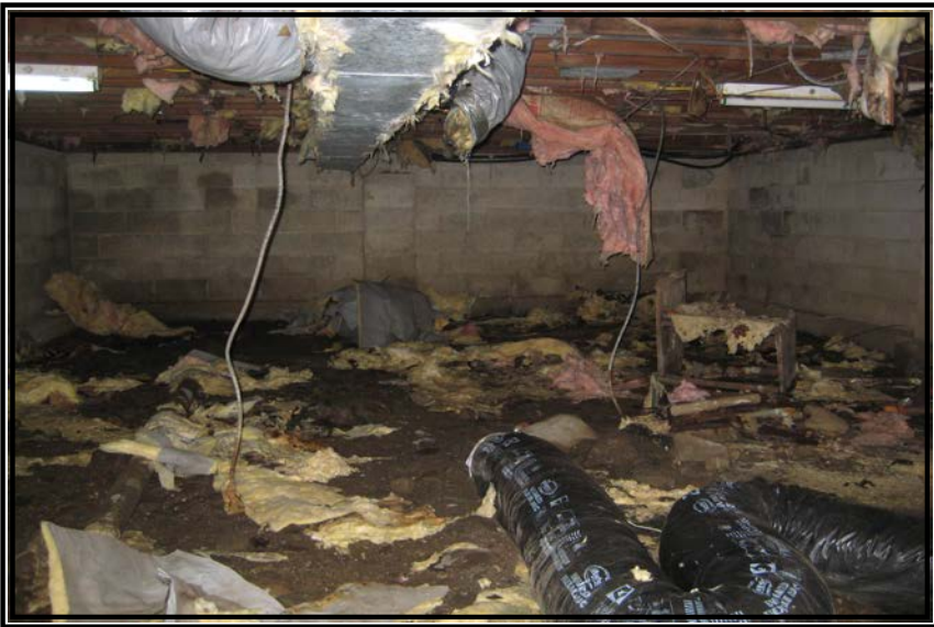
Photograph 7 Basement with mold on ceiling joist
