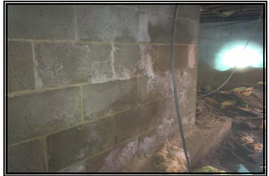
Photograph 6 Mold on concrete foundation wall
