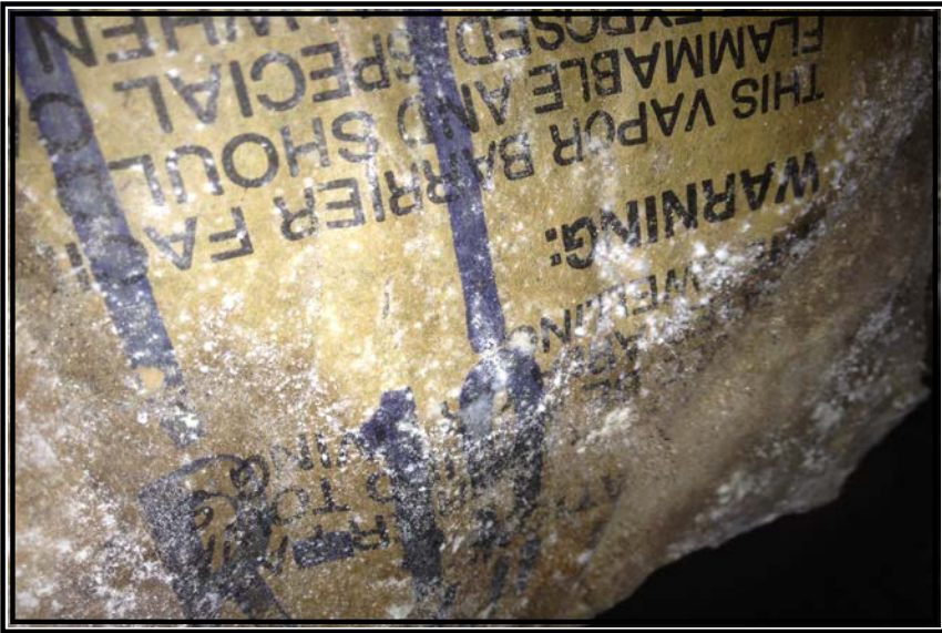
Photograph 5 Mold on insulation in basement
