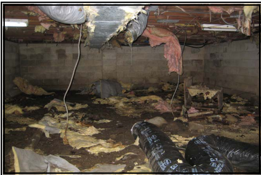
Photograph 7 Basement with mold on ceiling joist
