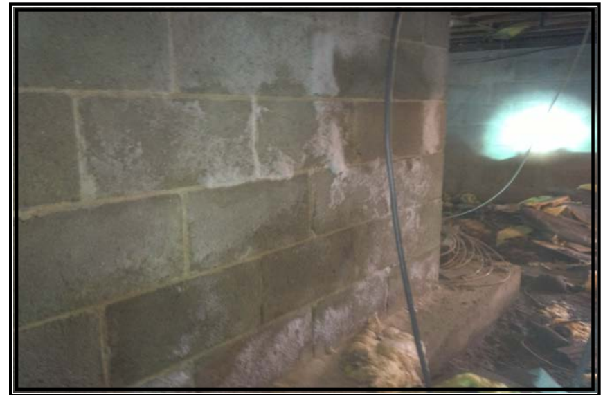
Photograph 6 Mold on concrete foundation wall
