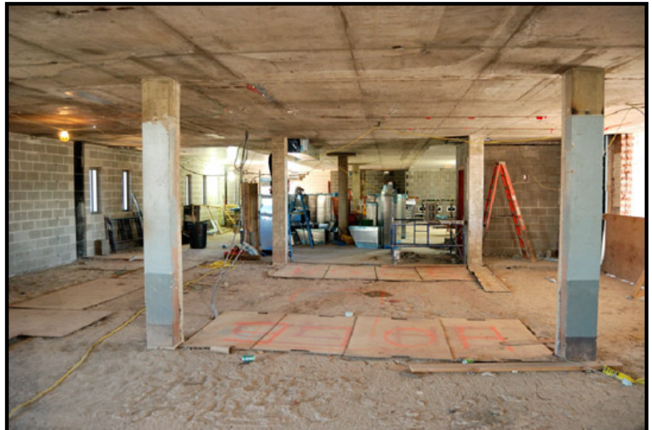
A view from the third floor of the Old North Wing - the central stairway has been removed.
