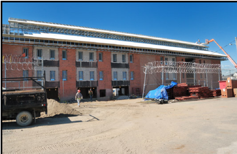
A new pitched roof is being installed on the Old North Wing of the Bridgeport Correctional Center.
