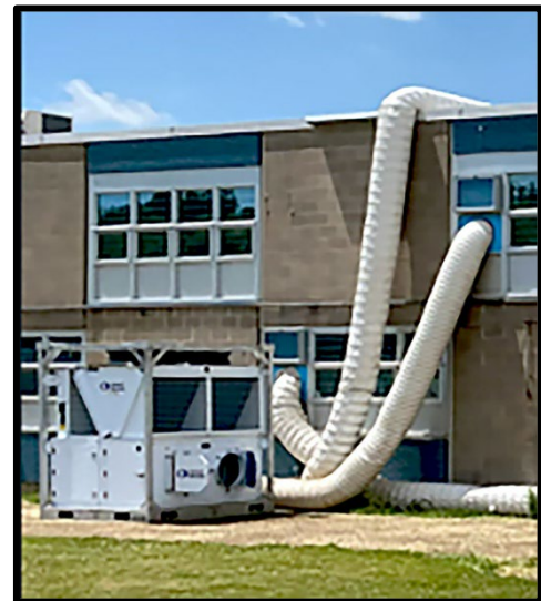
Air Handling Unit Outside the Osborn facility
