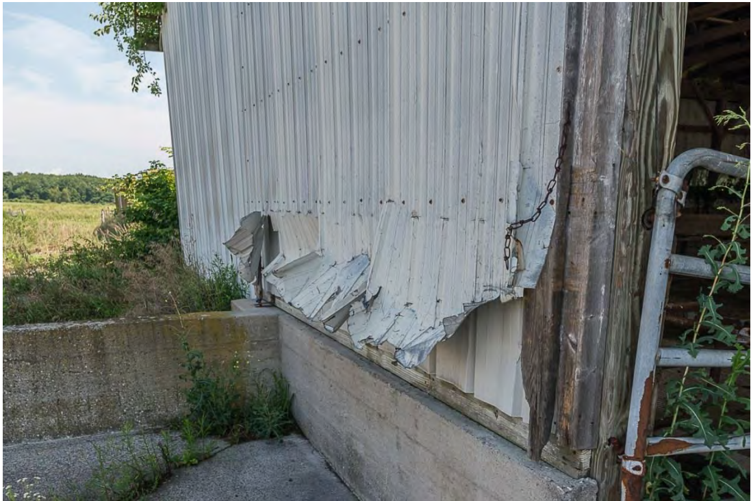
Photo 46. Building 10 view north of west elevation showing damage to siding.
