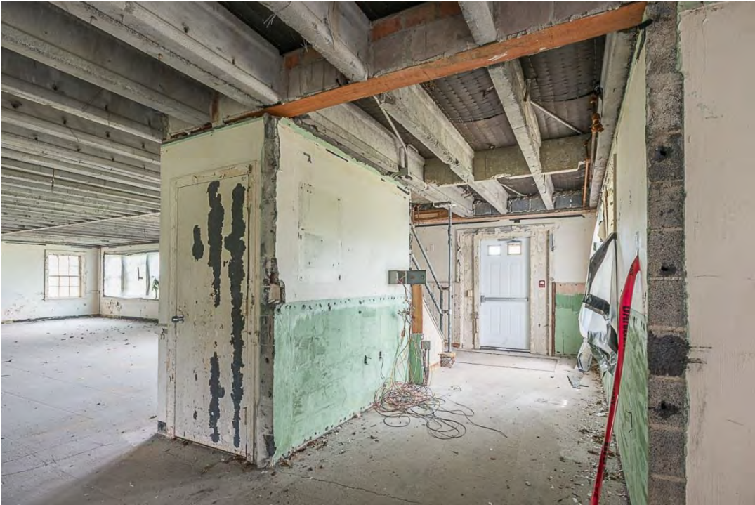
Photo 7. Building 1, first floor interior view north showing exposed floor joists and stair enclosure.
