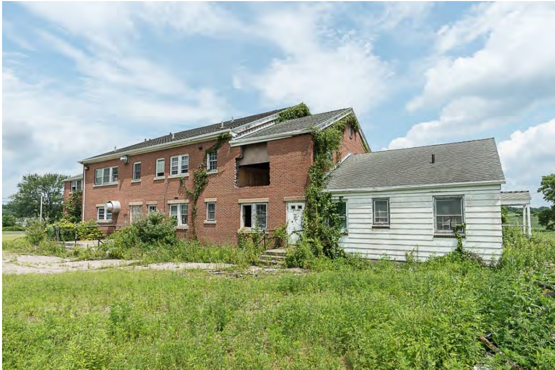
Photo 4. Building 1, view north showing south elevation with hole on second floor.
