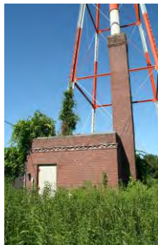
Existing Pump House
