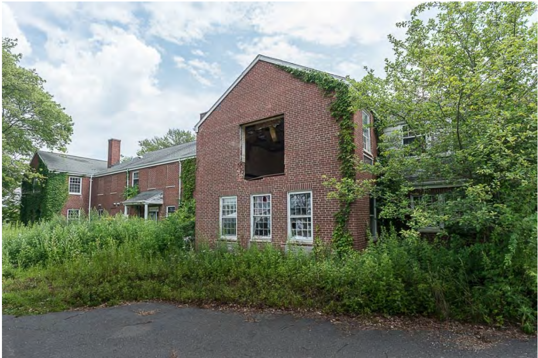
Photo 24. Building 4, view east showing north elevation with hole on second floor.
