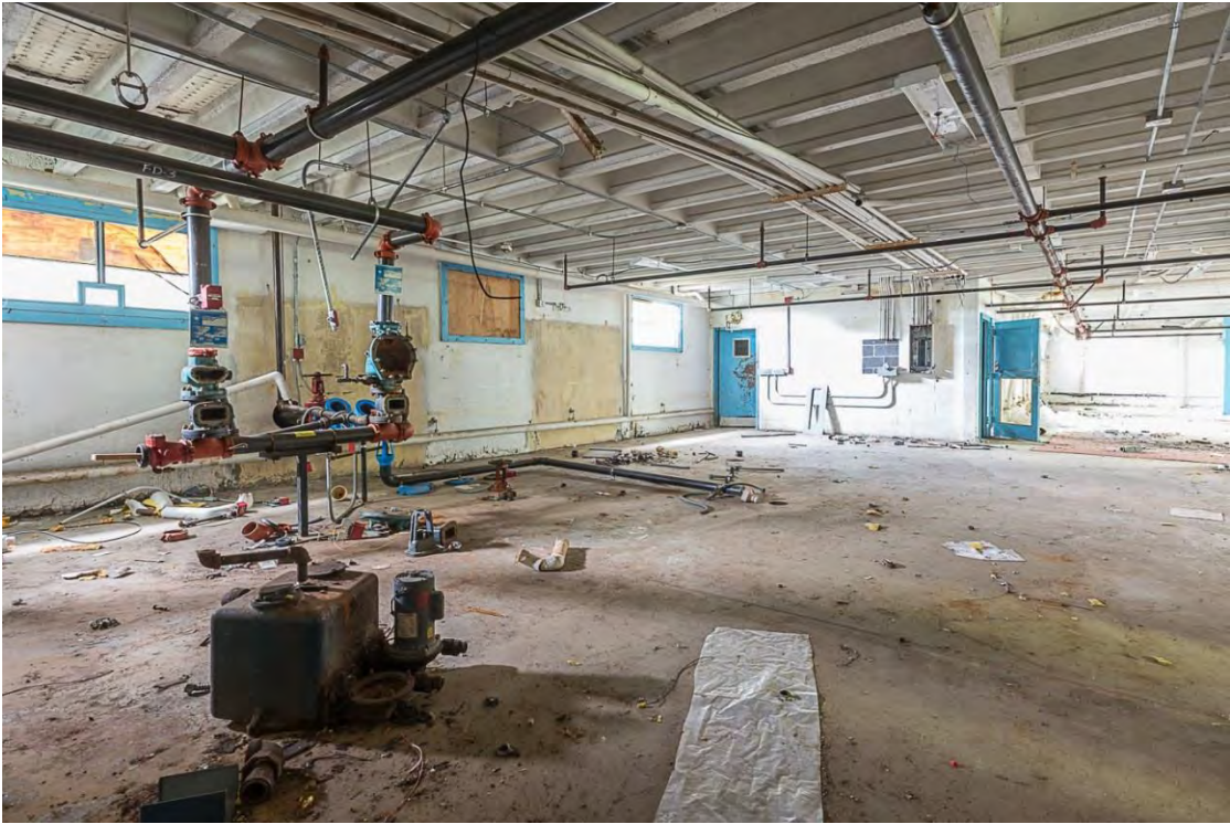
Photo 11. Building 1, basement interior view southeast showing exposed floor joists and heating pipes.
