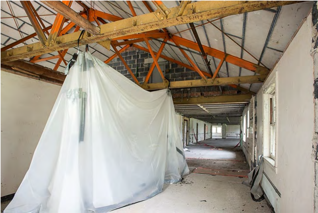
Photo 6. Building 1, first floor interior view northwest showing exposed trusses for east wing.
