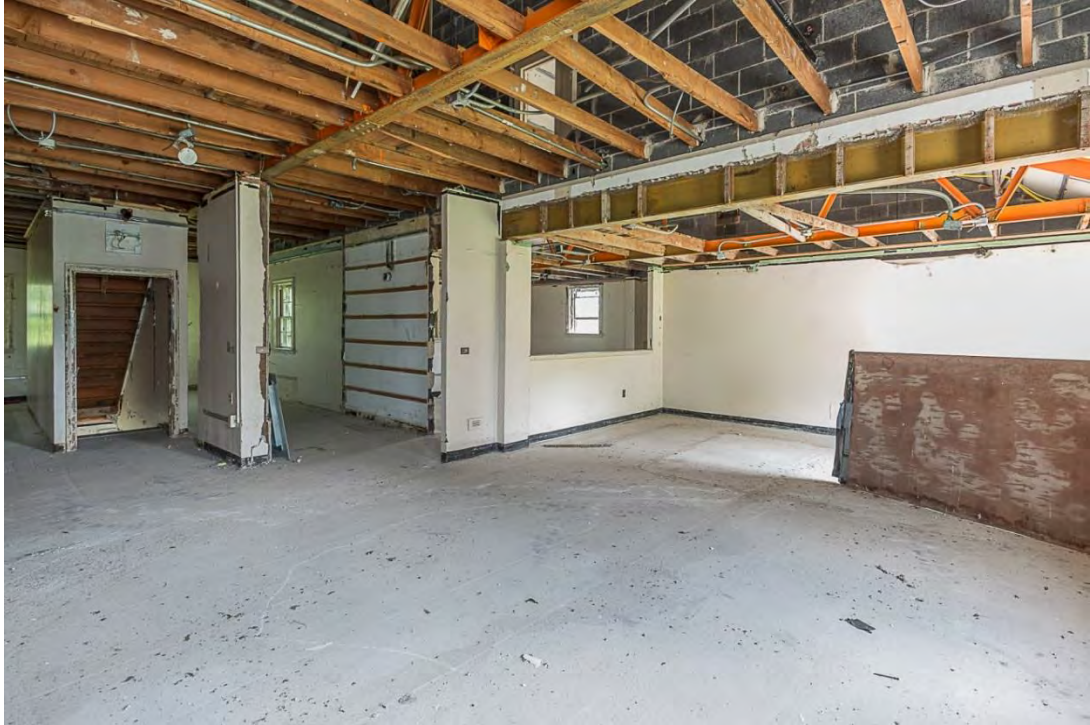
Photo 9. Building 1, first floor interior view southeast showing exposed rafters and remaining walls.
