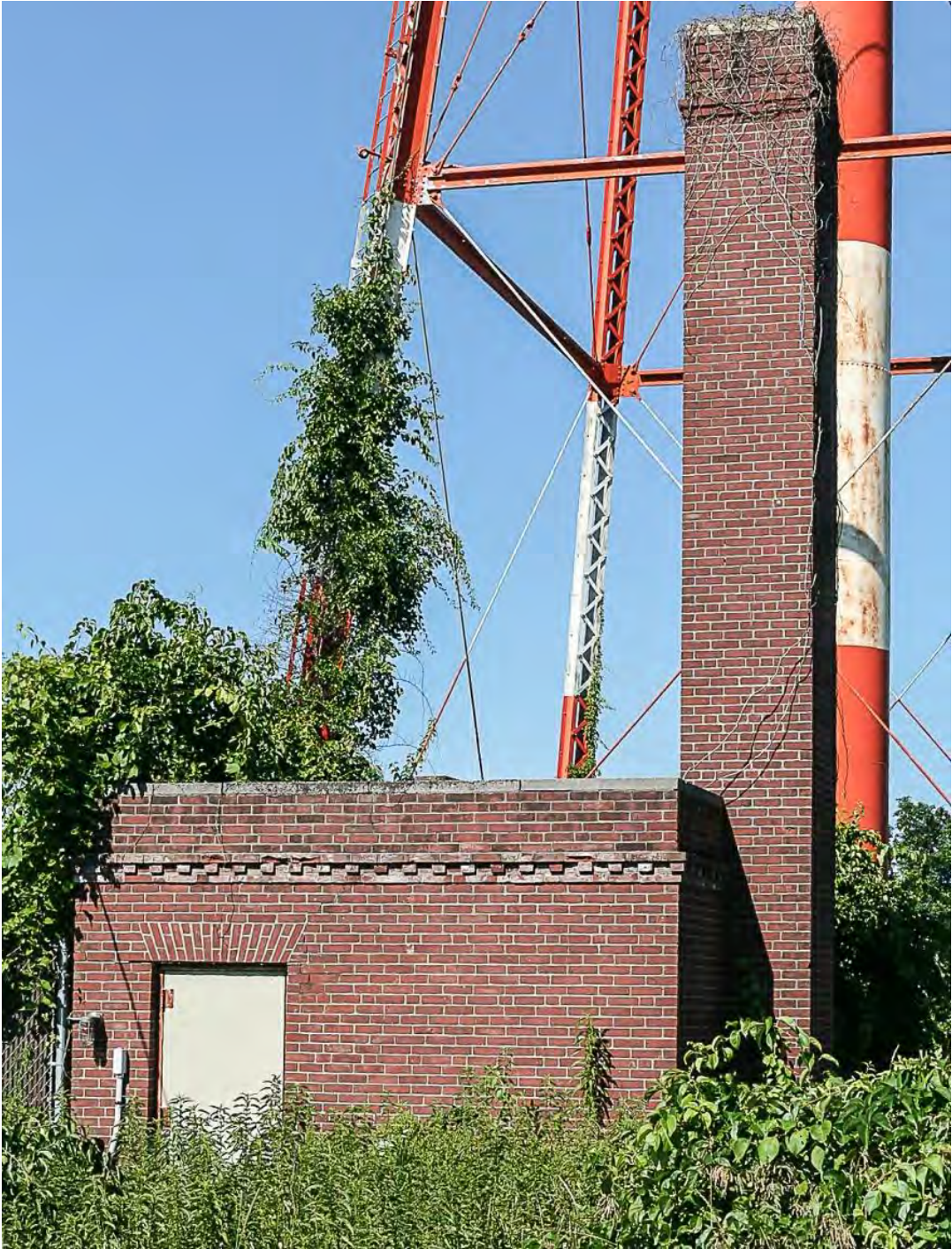
Photo 48. Water tower and pump house, view north showing façade of pump house.
