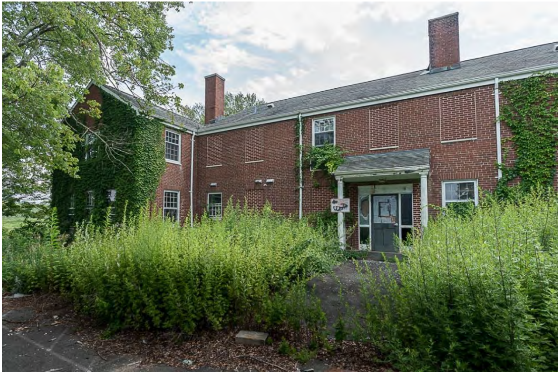
Photo 25. Building 4, view southeast showing north elevation, secondary entrance and bricked-in window openings.
