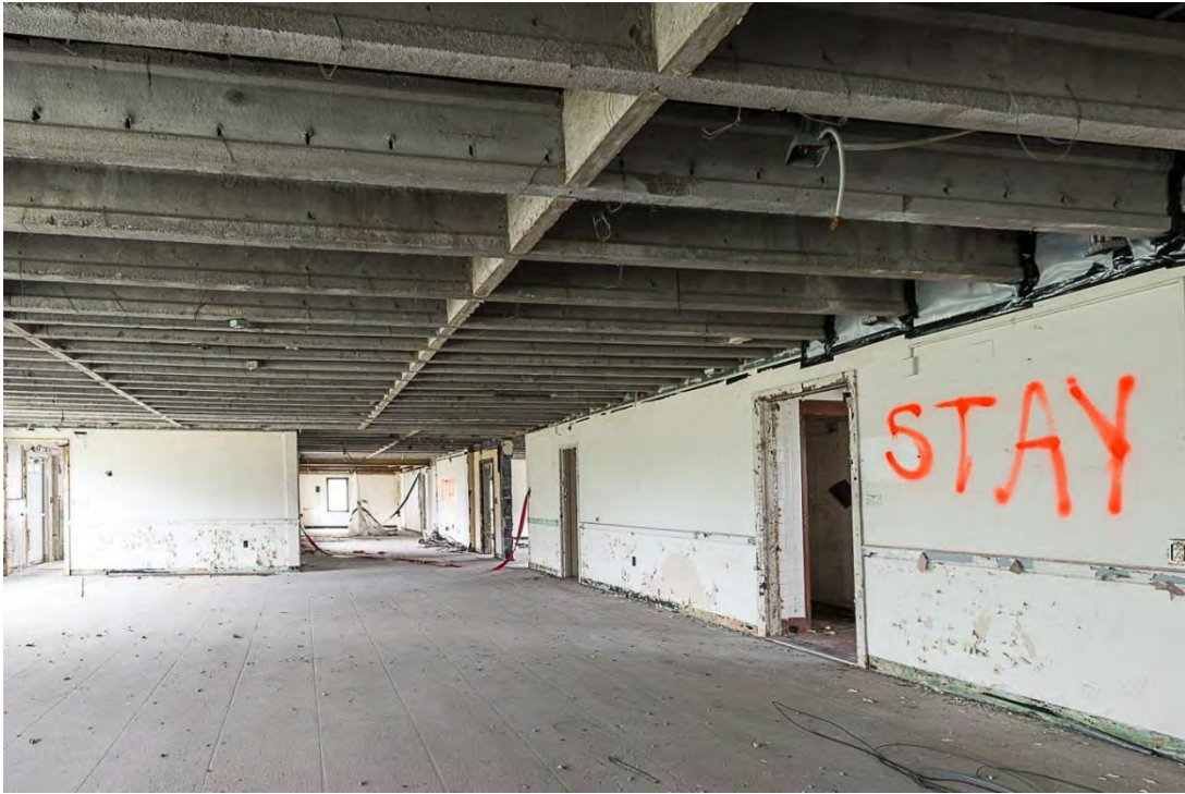
Photo 8. Building 1, first floor interior view north showing exposed floor joists and remaining walls.
