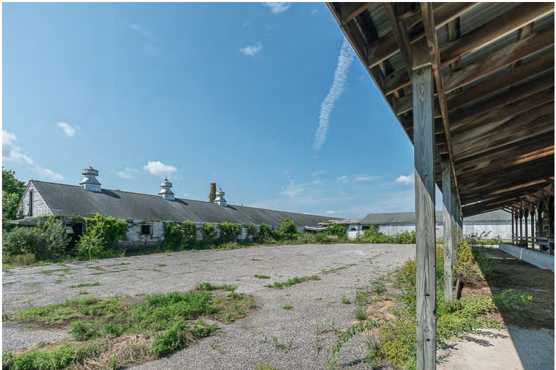
Photo 37. Building 8, view southwest showing east and north elevations of dairy barn, east elevation of hay barn and roof overhang on south elevation of heifer barn.
