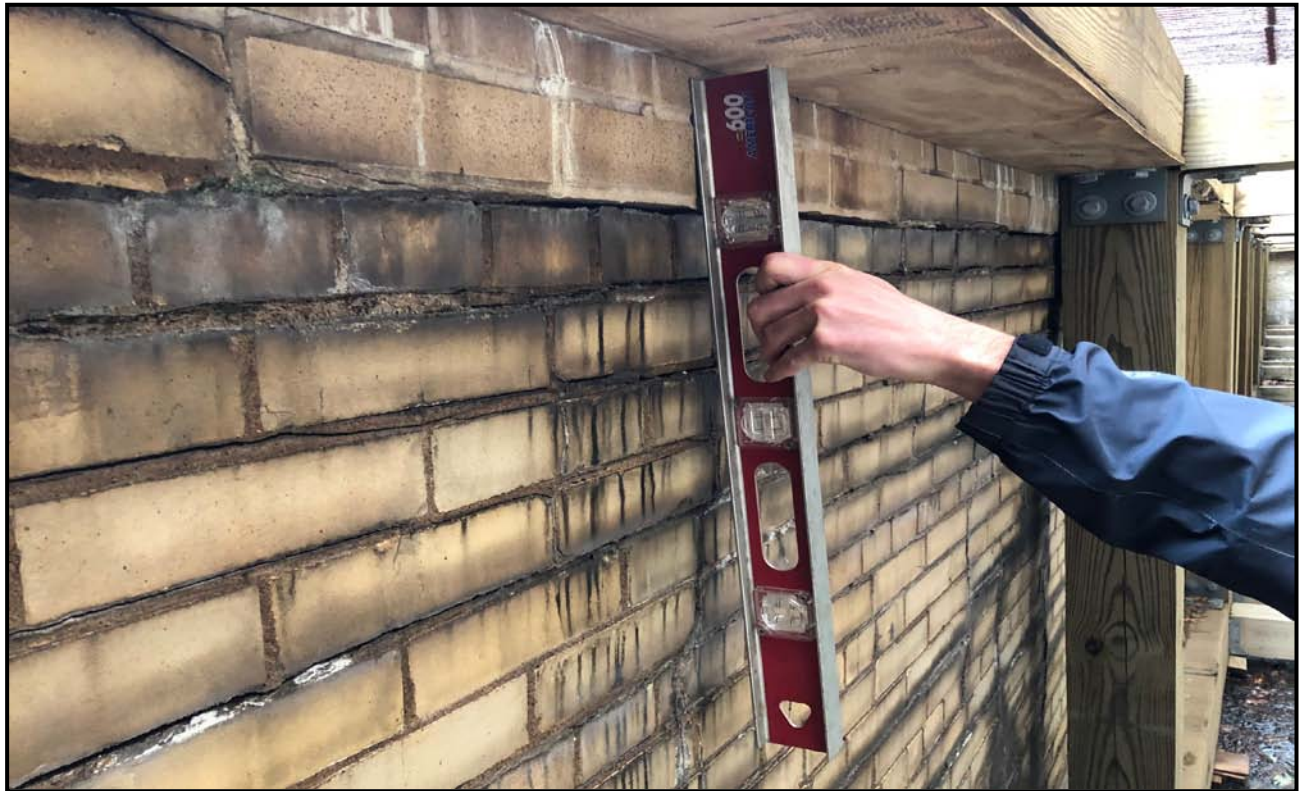
PHOTO 5 – Area way Wall Lateral Displacement
