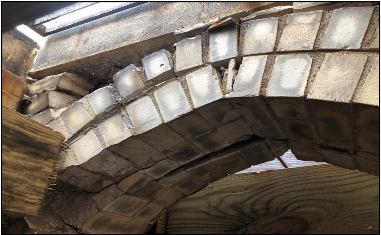
PHOTO 4 – Areaway Lateral Arch Deterioration
