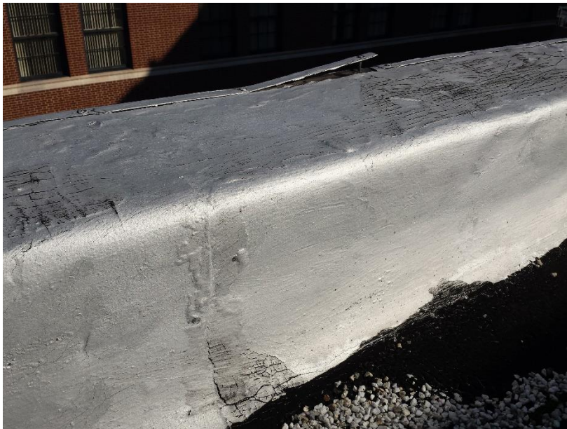
Figure 32. Loose termination bar at coping stone flashing.
