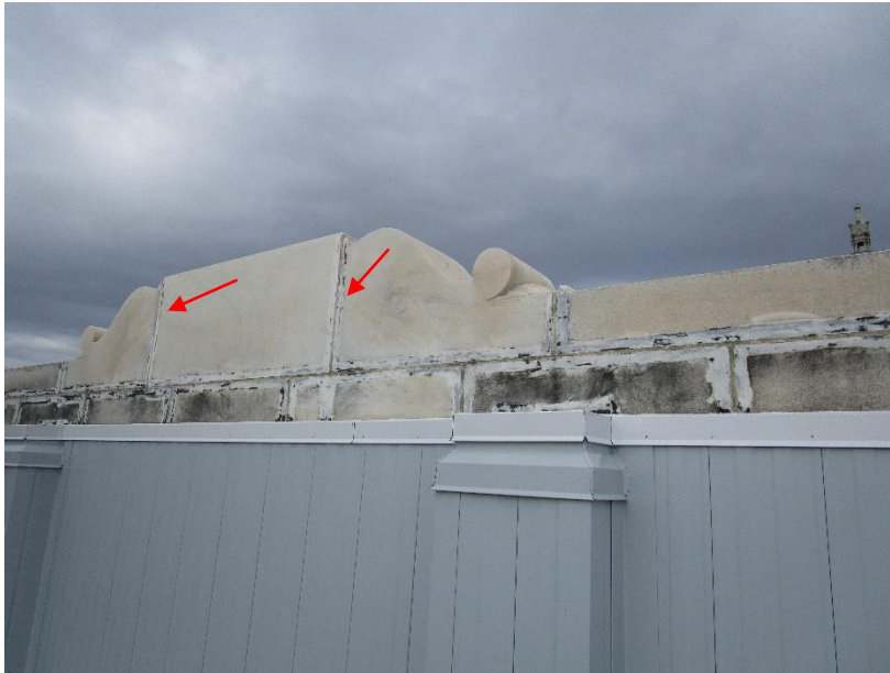
Figure 91. Adhesive sealant failure at joints between coping stones at the roof parapet.
