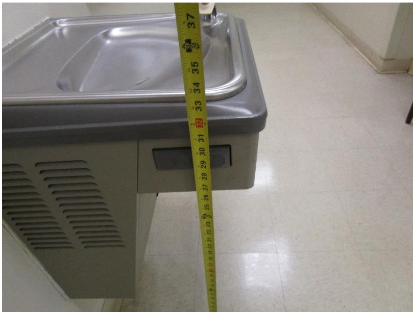
Figure 129. Accessible drinking fountain at 30 Trinity Street.
