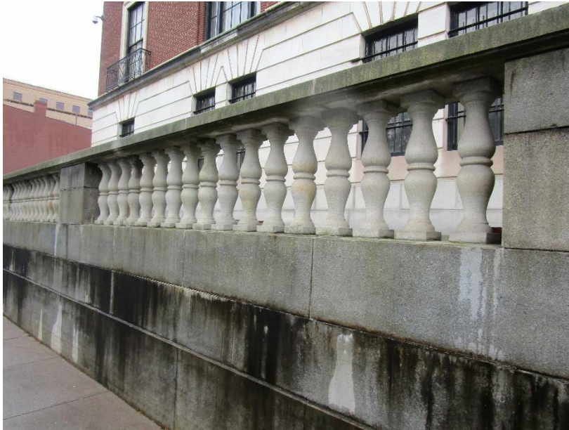
Figure 93. Organic soiling and mortar deterioration at north retaining wall.
