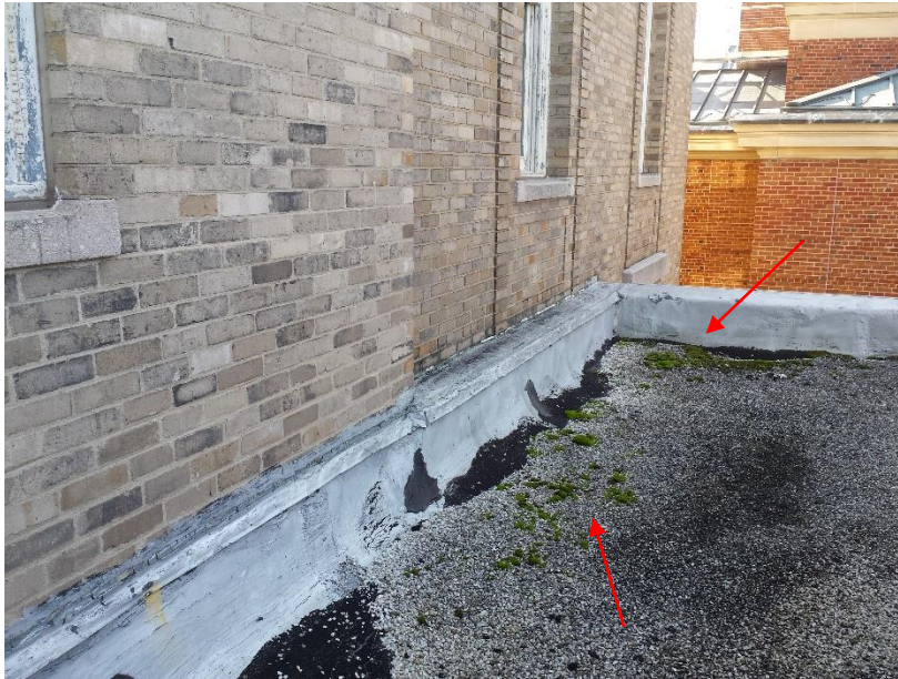
Figure 33. Organic growth on roof surface.
