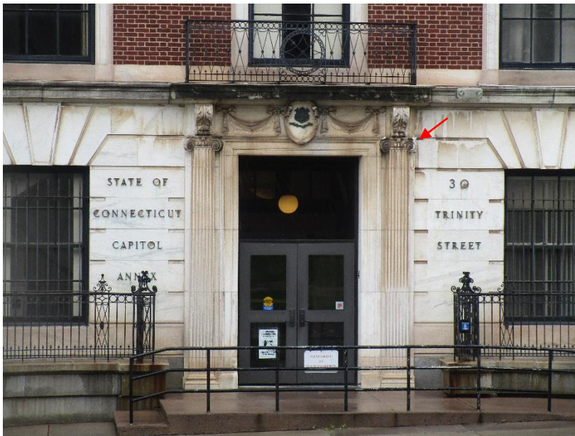
Figure 78. Soiling on marble at east elevation. Also note spall at column capital.
