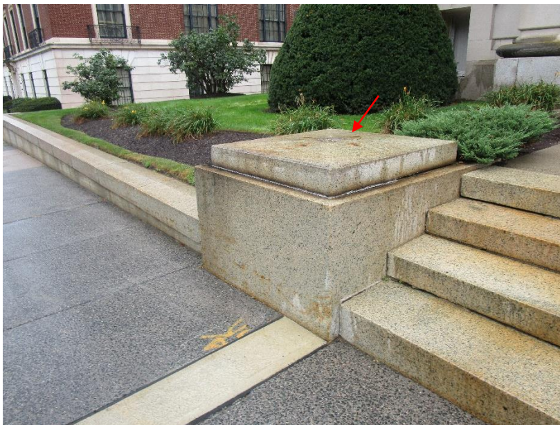
Figure 10. Anchors for missing light fixture. Staining on granite at stair and retaining wall.
