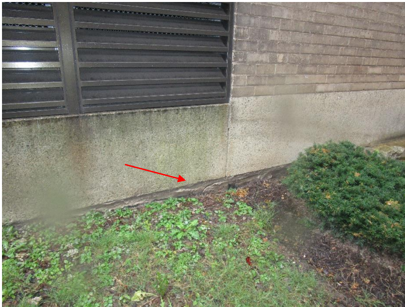
Figure 20. Spalls at concrete foundation.
