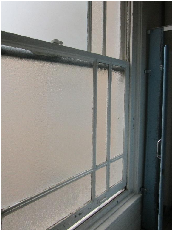
Figure 59. Peeling paint at interior window.
