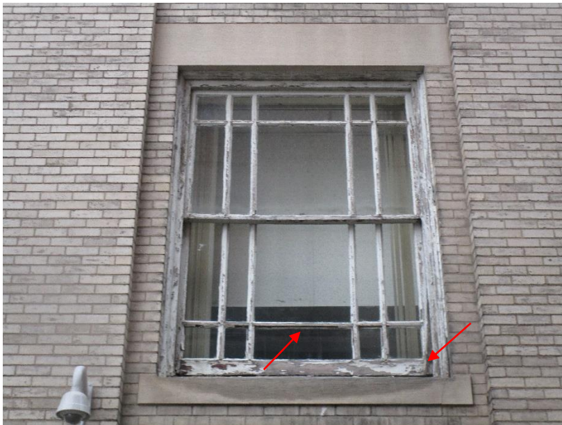
Figure 22. Double hung wood window at south elevation of 20 Trinity Street. Arrows point to damage and decay at wood sash and muntin.
