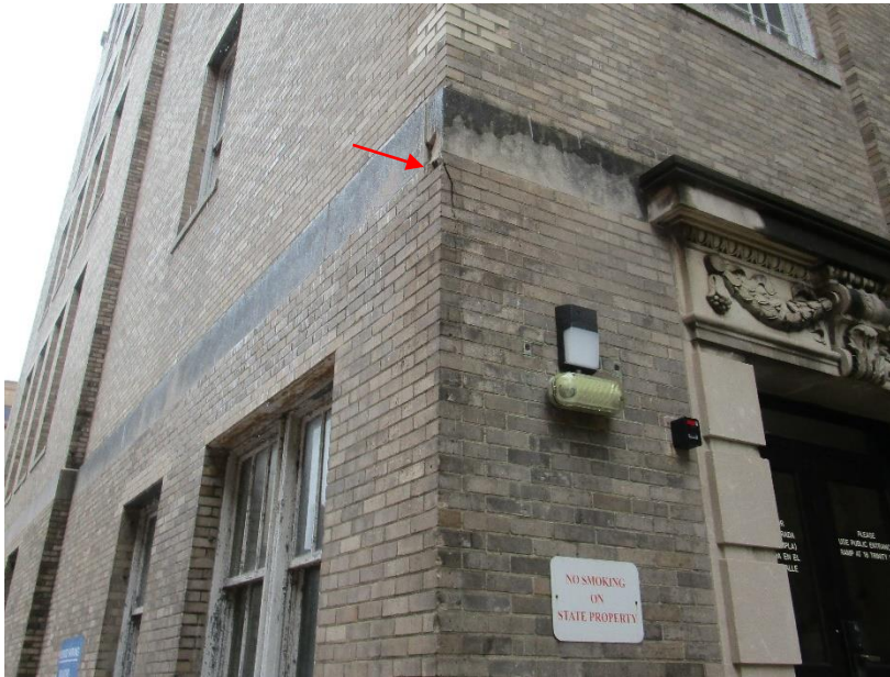
Figure 47. Spall at band stone and cracked bricks at the southwest corner of 18 Trinity Street.
