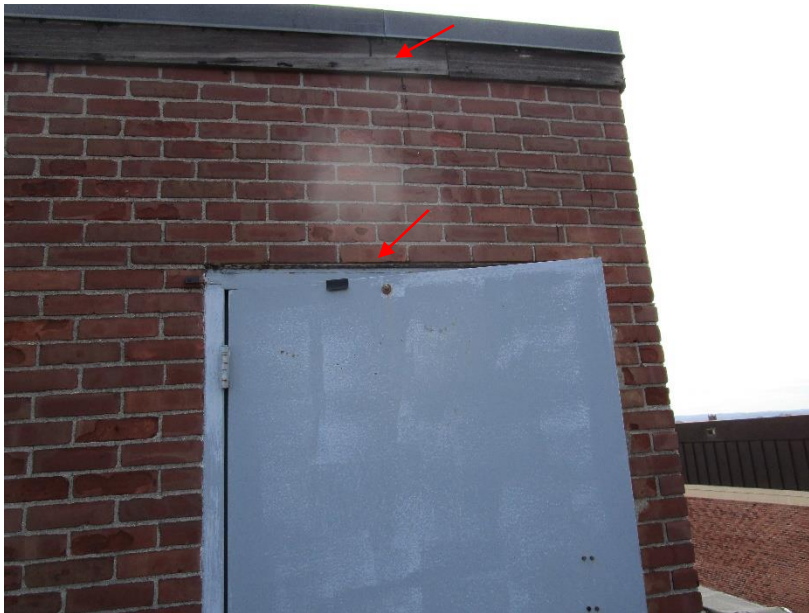
Figure 70. Corrosion at steel lintel at top of door opening and exposed wood nailer below roof edge.
