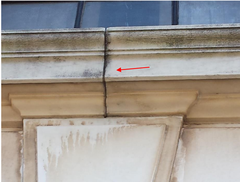
Figure 89. Loose mortar in marble cornice joint.
