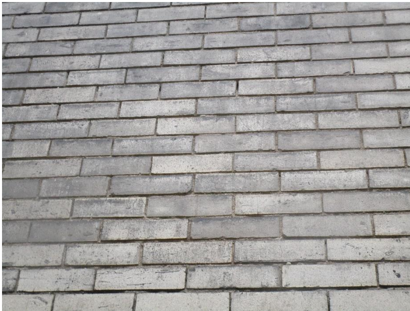
Figure 18. Mortar in brick joints at north elevation.
