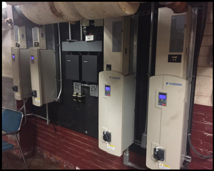
Exhibit "E8" Mechanical Equipment VFD's
