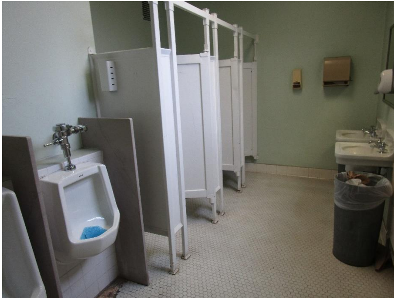
Figure 120. Non-accessible toilet room at third floor of 18 Trinity Street.
