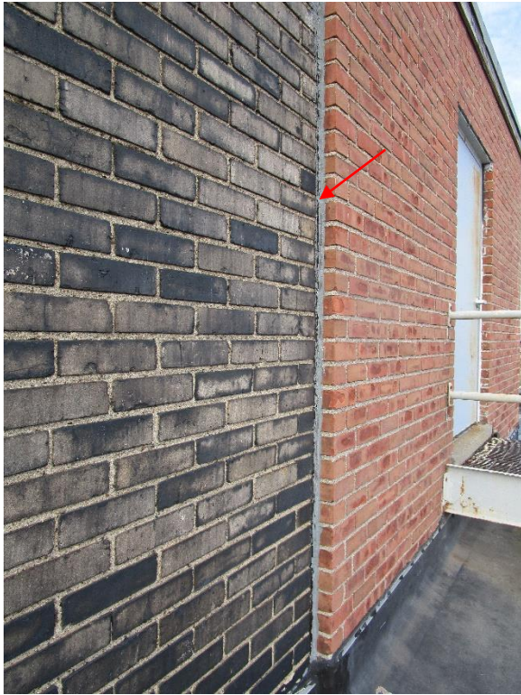
Figure 69. Adhesive sealant failure at vertical joint between chimney and penthouse. Also note faded paint and surface rust on stair and door to penthouse.
