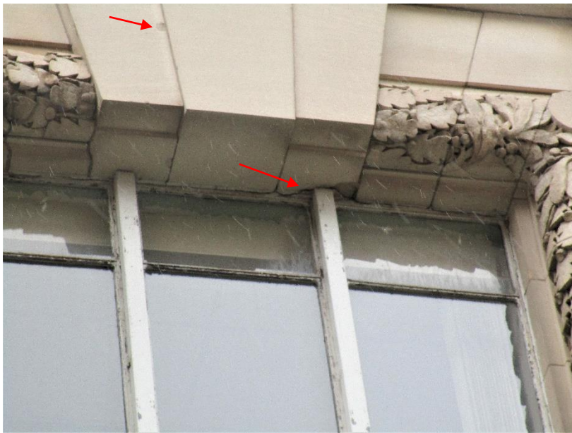
Figure 4. Spalled stone at intersection with window mullion at north elevation of 20 Trinity Street. Also note small spall at keystone.
