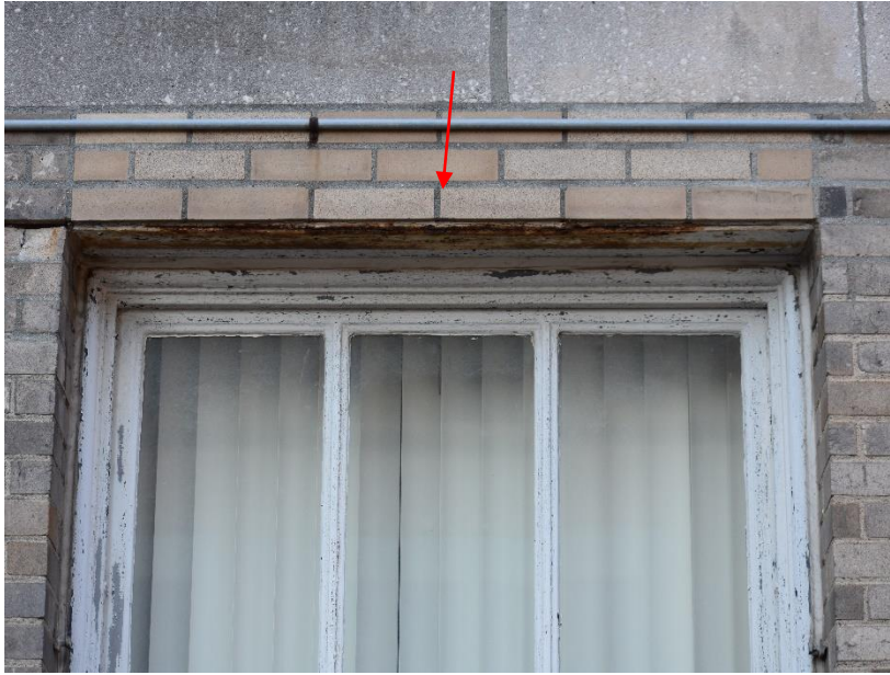
Figure 51. Corrosion and deflection at steel lintel.
