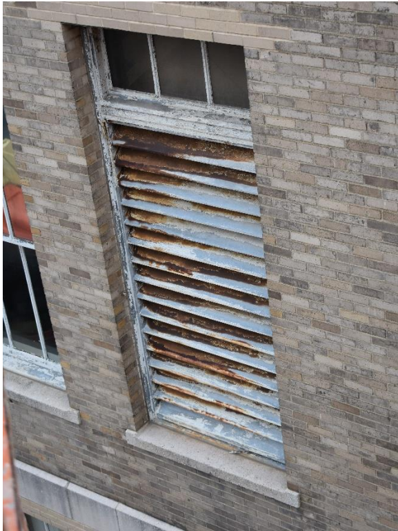
Figure 61. Corrosion at steel louver.
