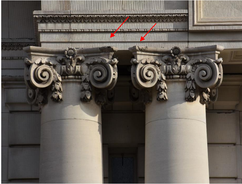
Figure 5. Erosion of limestone at column capitals.
