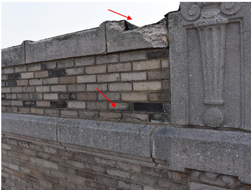
Figure 46. Delamination of cast stone coping. Also note cracks at face bricks.
