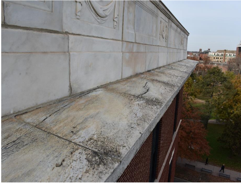
Figure 85. Cracks at upward facing surface of the parapet cornice.
