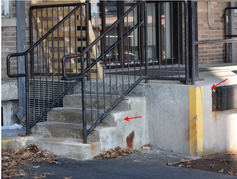
Figure 57. Concrete spalls at treads and cracks in concrete at loading dock.
