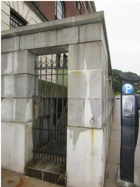
Figure 94. Mortar deterioration and rust stains at east retaining wall.
