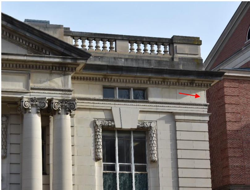
Figure 6. Crack in limestone at southwest corner of 20 Trinity Street. Also note soiling at cornice, balustrade and pediment.
