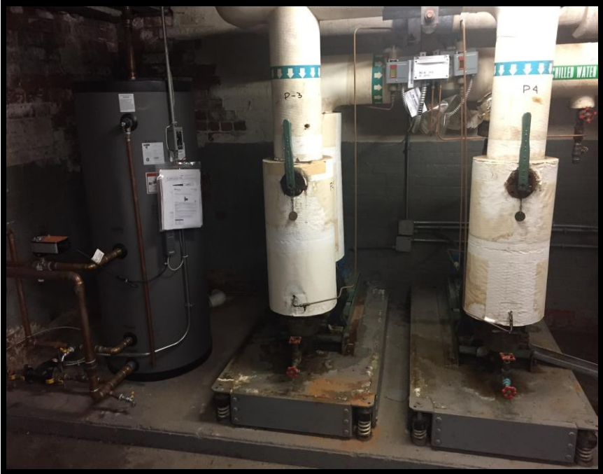
Exhibit "M1" Recently Replaced Water Heater
