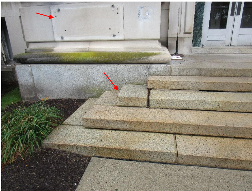
Figure 8. Granite displacement at west entrance stair and anchors in stone left after signage removal.
