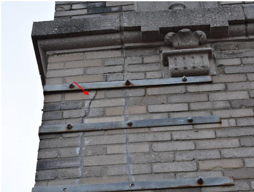
Figure 44. Cohesive sealant failure at crack repair.
