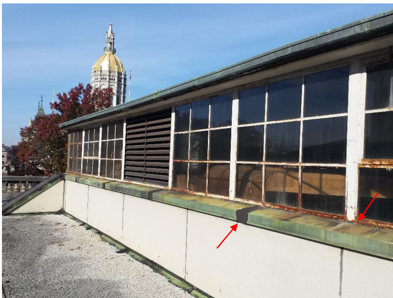
Figure 34. Corrosion at steel windows and repairs at copper sill joints at 20 Trinity Street mechanical penthouse.
