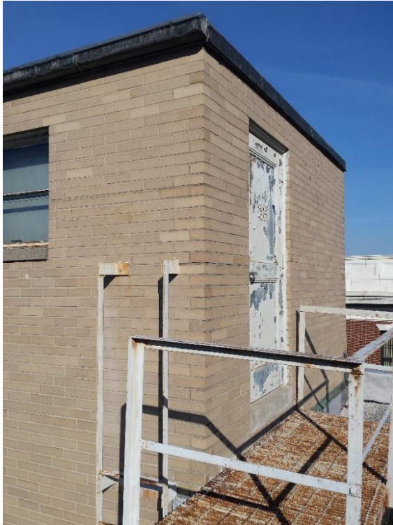
Figure 35. Elevator penthouse at 20 Trinity Street.
