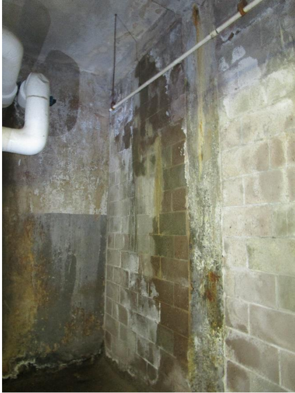
Figure 73. Leak into basement vault at 18 Trinity Street.
