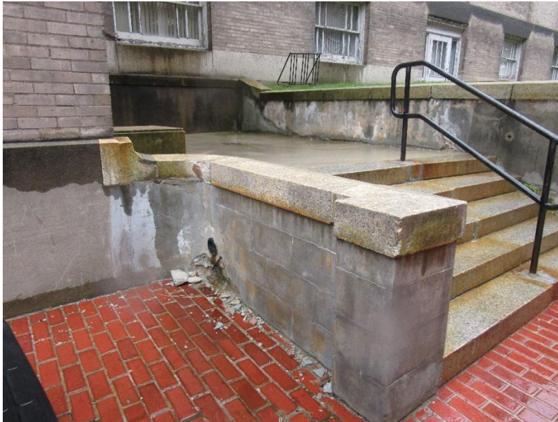
Figure 55. Concrete deterioration at stair and retaining wall at the northwest corner of 18 Trinity Street.
