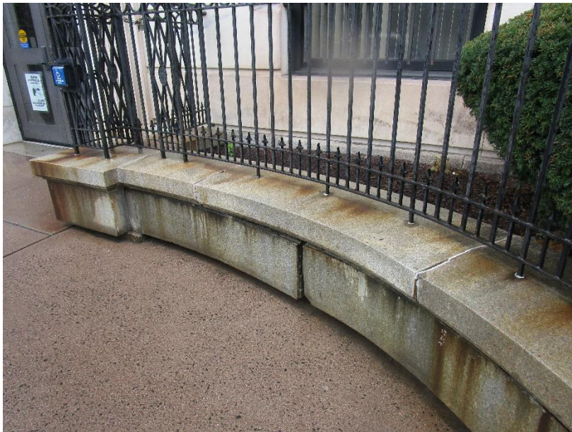
Figure 92. Stone displacement, spalls, mortar deterioration, rust staining, and joint sealant deterioration at retaining wall.
