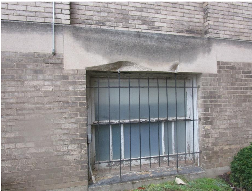
Figure 16. Spalls at stone lintel.
