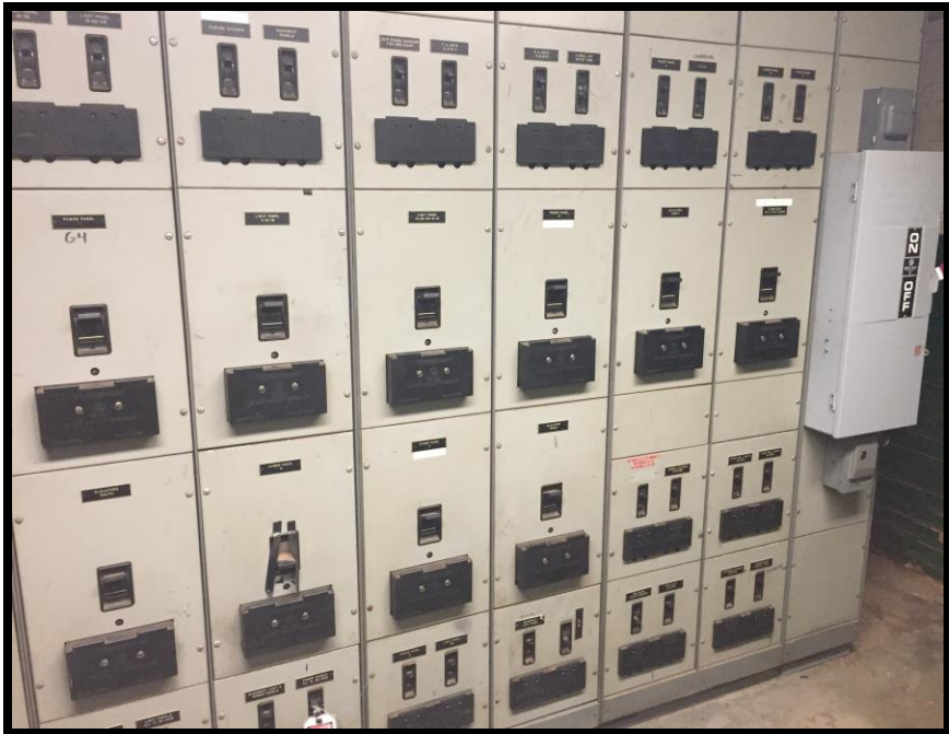
Exhibit "E2" 18-20 Trinity Street Electrical Distribution
