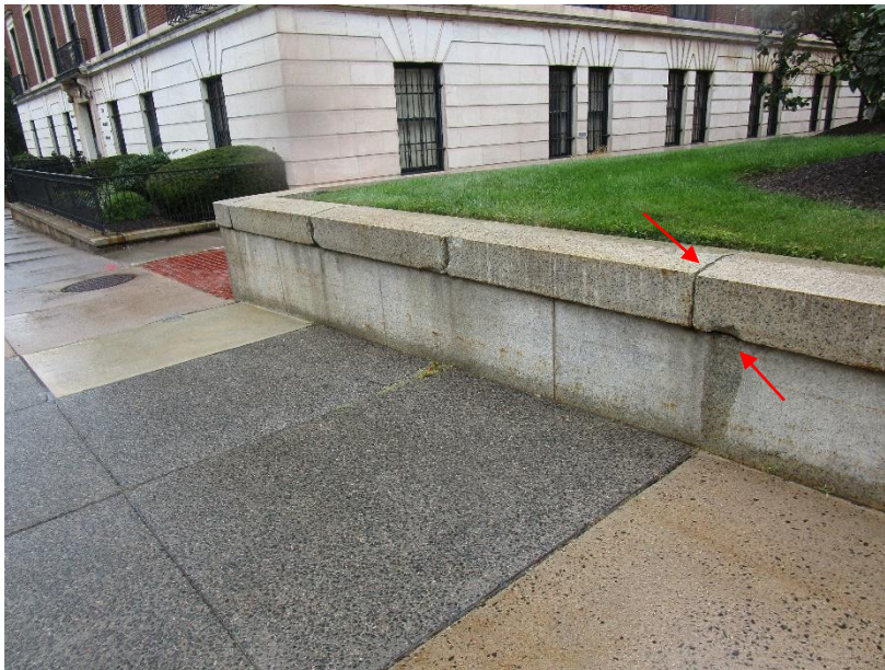
Figure 12. Spalls and mortar deterioration at granite retaining wall.
