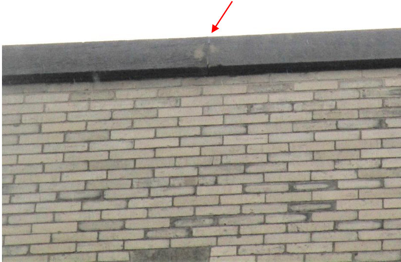
Figure 19. Mortar deterioration at coping joint.
