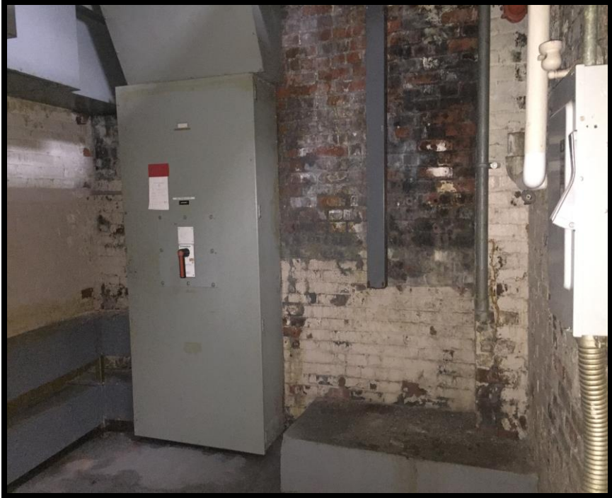
Exhibit "E5" 30 Trinity Street Main Switch
