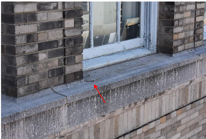
Figure 48. Spall at cast stone window sill at 18 Trinity Street.
