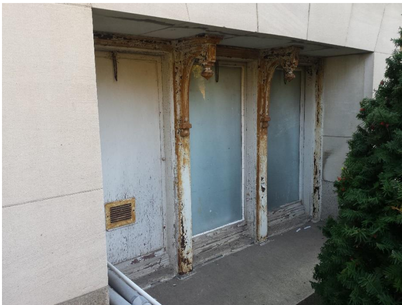
Figure 24. Peeling paint at wood and iron surfaces as well as surface rust on iron at ground level window.
