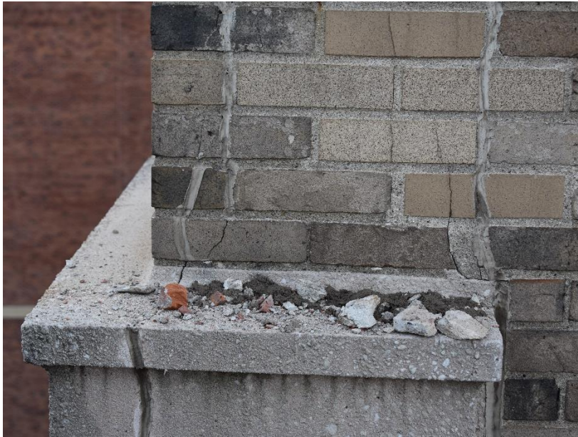
Figure 45. Cracks adjacent to and below sealant crack repairs.
