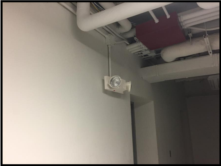
Exhibit "E4" Emergency Egress Lighting
