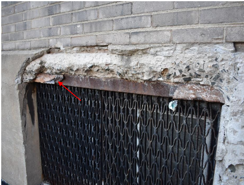
Figure 56. Concrete deterioration at ground floor of north elevation. Note the volume of the corrosion at the steel frame at the left hand side of the figure.
