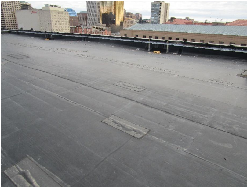
Figure 65. Blisters under roof patches at 18 Trinity Street.
