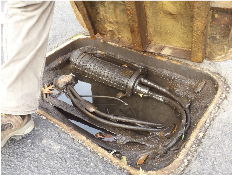
Figure 75. Apparent pump above vault at 18 Trinity Street.
