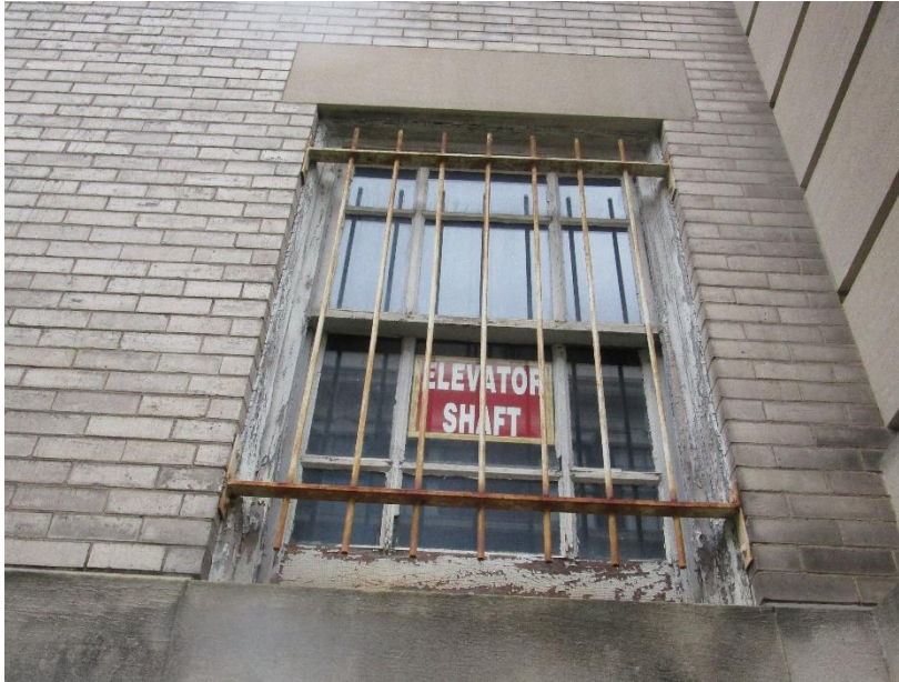
Figure 17. Paint failure and surface rust at window security grille.
