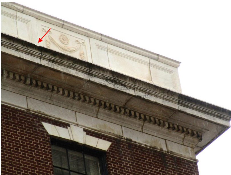
Figure 84. Spall at cornice.
