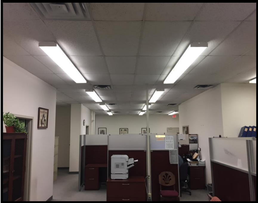
Exhibit "E3" Office Area Lighting
