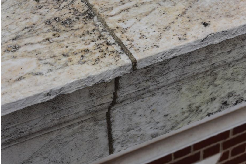
Figure 87. Stone crumbling at edge of cornice.
