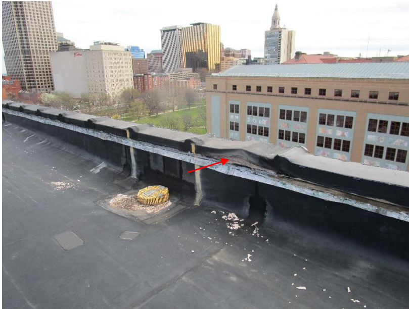
Figure 67. Membrane adhered to cast stone copings. Delaminated cast stone below membrane.
