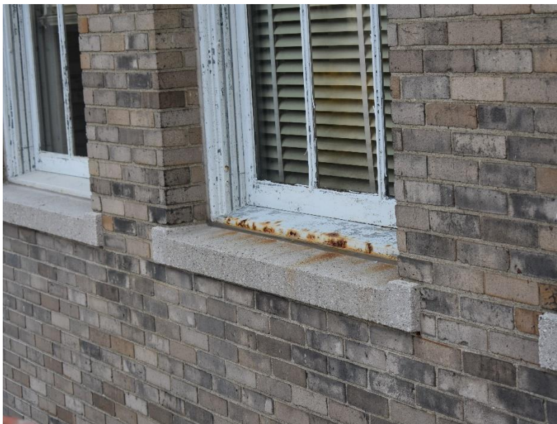
Figure 60. Corrosion through a steel window sill.
