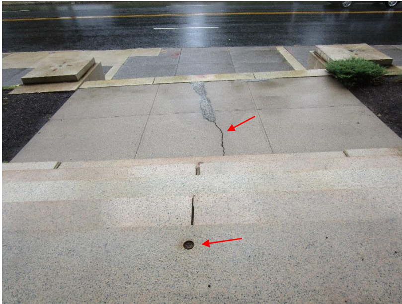
Figure 9. Crack and surface loss in concrete landing at stair to west entrance. Also note sleeve for missing handrail post.
