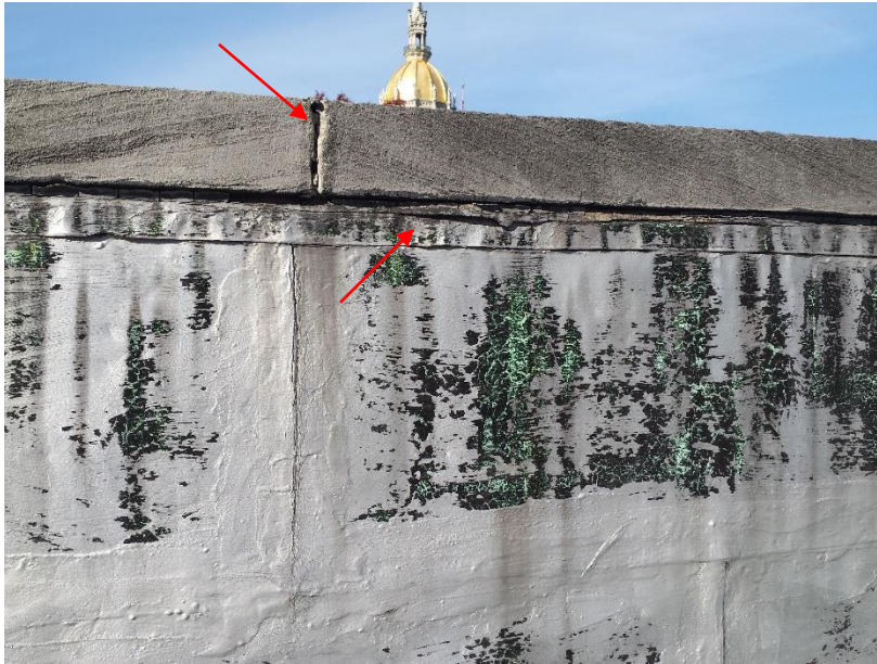
Figure 31. Aluminized coating failure at copper panels at roof parapet as well as mortar and sealant failure at coping stones.
