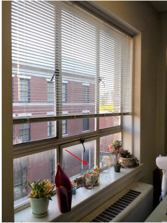
Figure 25. Cracked glass at window.
