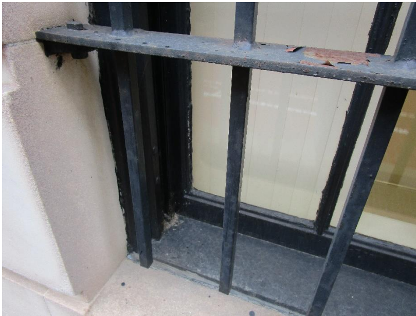
Figure 80. Peeling paint and surface rust at window security grille.
