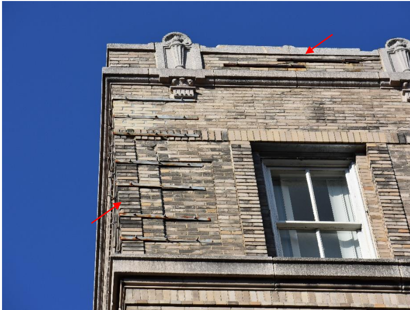
Figure 41. Strap repairs at east roof parapet at 18 Trinity Street. Also note soiling and staining on the brick and cast stone surfaces.
