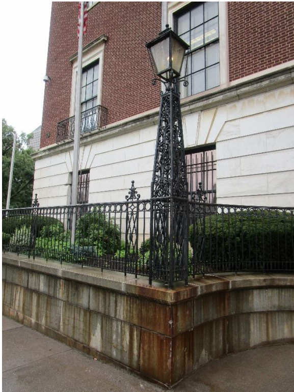
Figure 95. Peeling paint and surface rust on iron railing and light fixture causing rust stains on the stone retaining wall.
