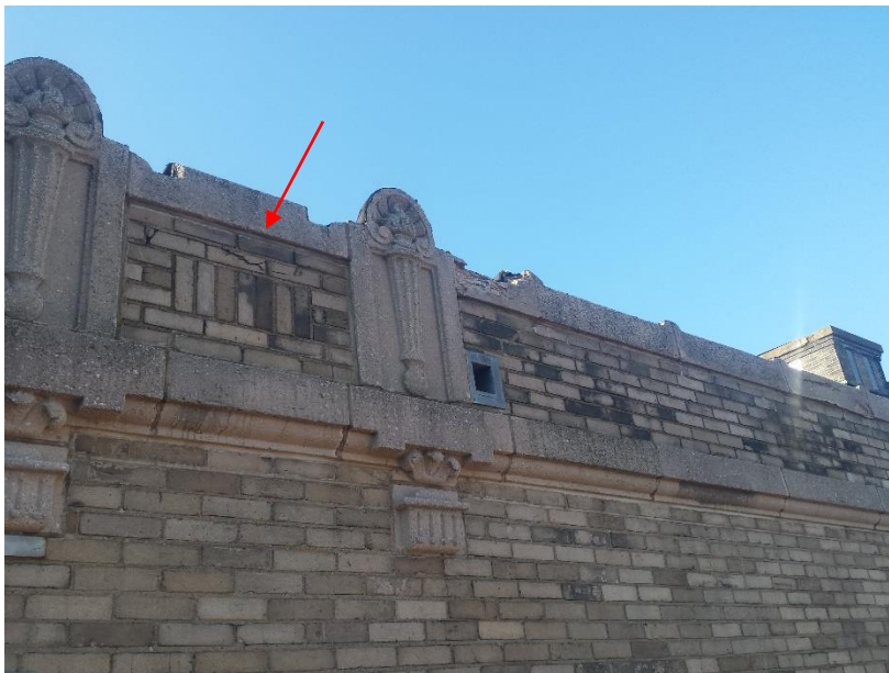
Figure 50. Spalled face brick at roof parapet.
