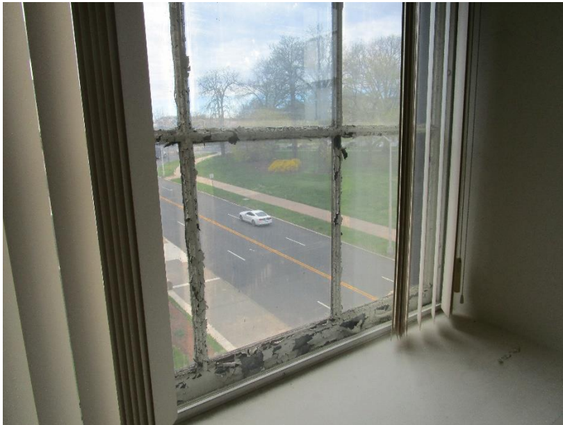
Figure 97. Peeling paint at interior surface of window.
