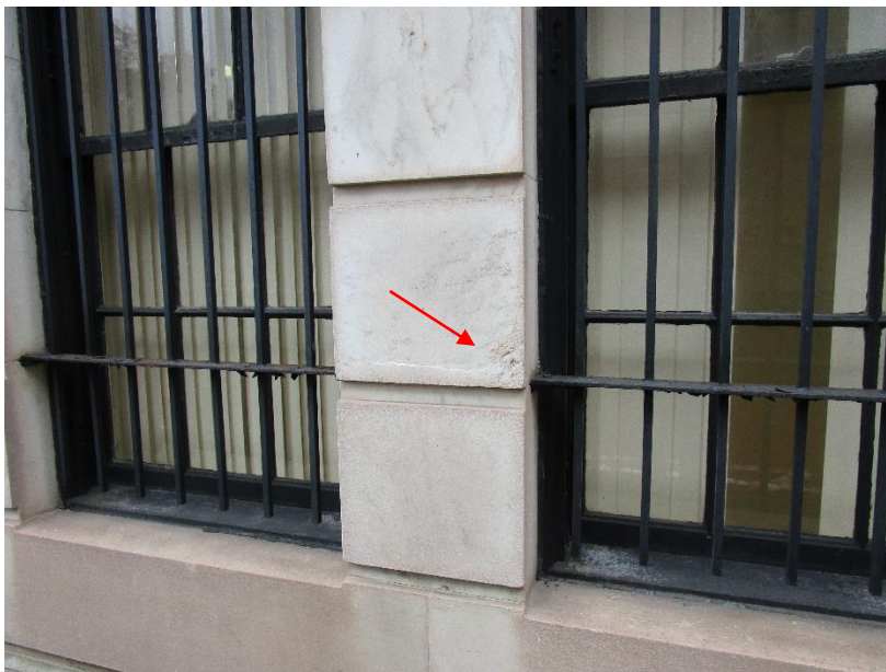
Figure 82. Surface erosion at marble unit.
