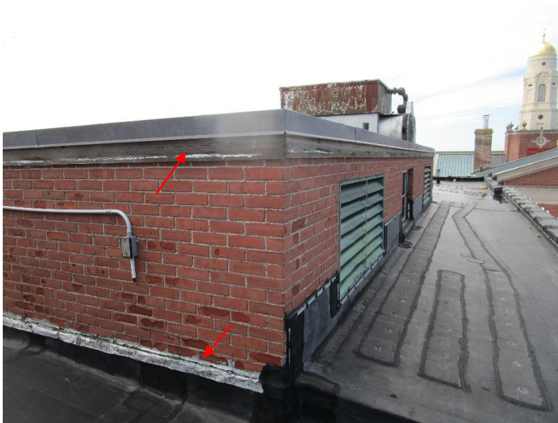
Figure 64. Patches at roof membrane. Also note deteriorated sealant in the joint above the counter flashing and exposed wood nailer below the roof edge.
