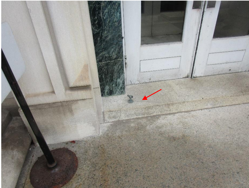
Figure 7. Crack at granite door sill.
