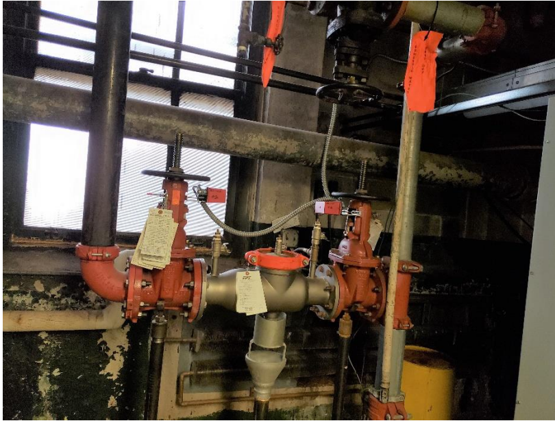
Figure 111. Standpipe Incoming Water Supply.
