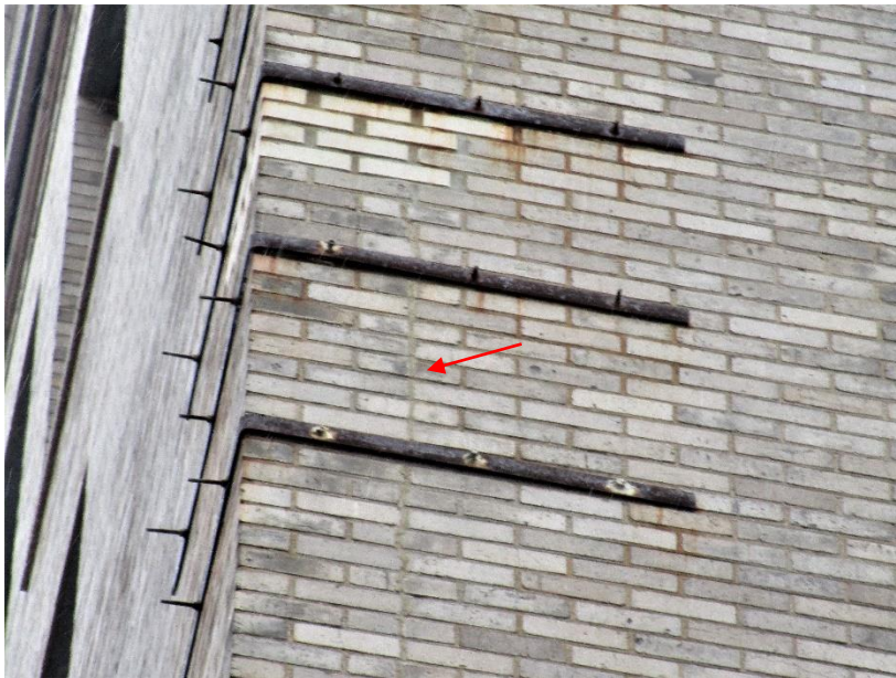
Figure 40. Corrosion at steel reinforcement straps and fasteners. Also note crack filled with elastomeric sealant.
