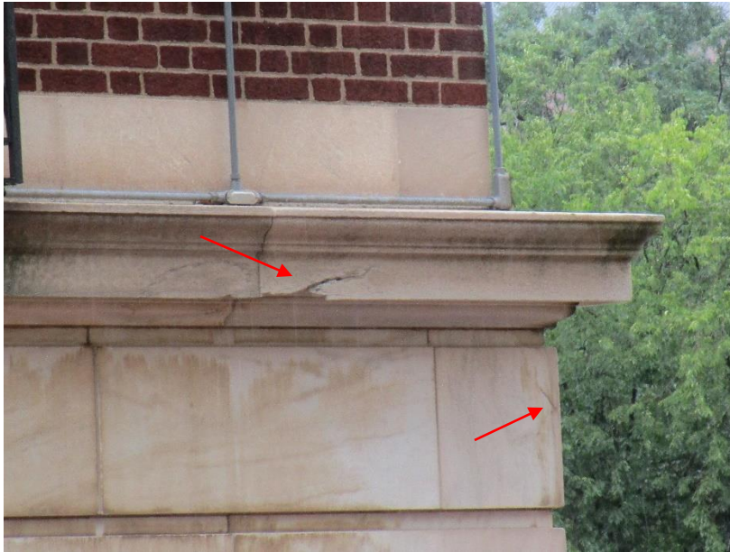
Figure 81. Spall at first floor cornice and cracked stone below cornice at the southeast corner of 30 Trinity Street.
