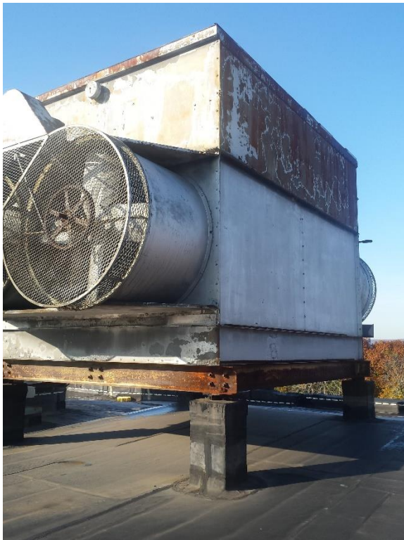
Figure 68. Cooling tower reported to be abandoned at 18 Trinity Street.
