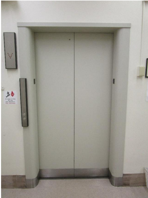
Figure 118. North elevator at 18 Trinity Street.
