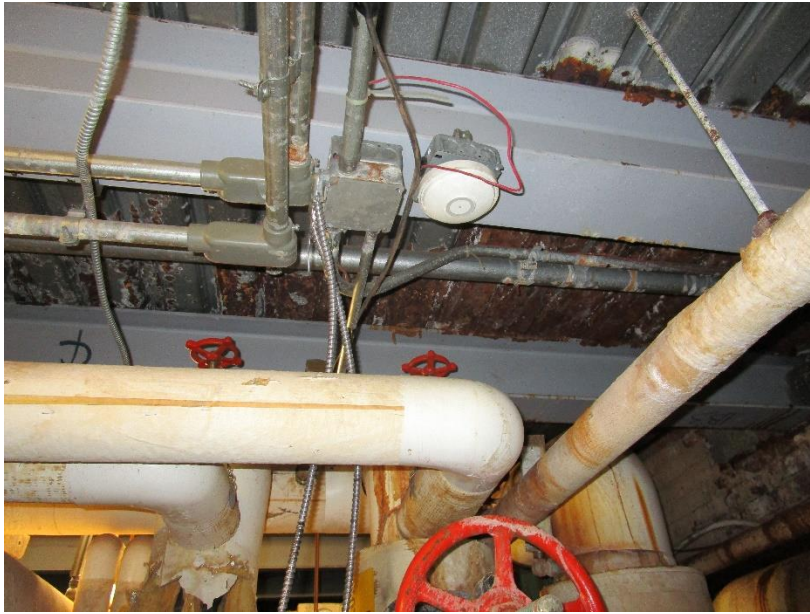
Figure 105. Corrosion at roof deck at vault at 30 Trinity Street.
