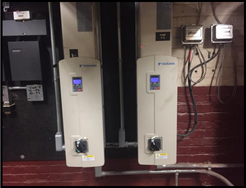
Exhibit "M4" Mechanical Equipment VFD's
