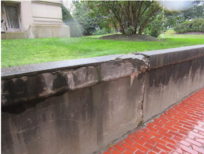
Figure 13. Concrete deterioration at retaining wall at the north side of 20 Trinity Street.
