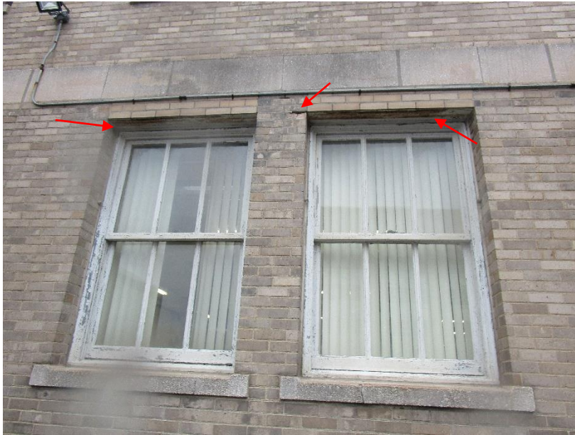
Figure 53. Surface rust on steel lintels at window openings. Also note spalled brick where the lintel bears on the masonry.
