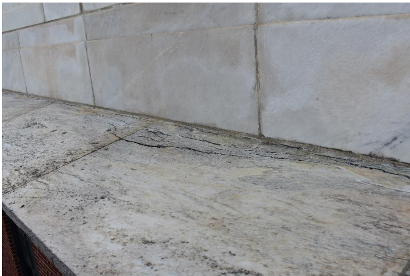
Figure 86. Cracks at upward facing surface of the parapet cornice.
