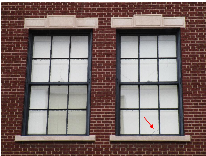
Figure 96. Faded paint finish at steel window and cracked glass at window panes.
