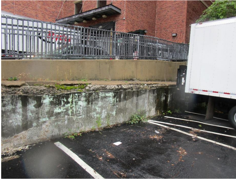
Figure 109. Concrete deterioration at parking lot retaining wall.
