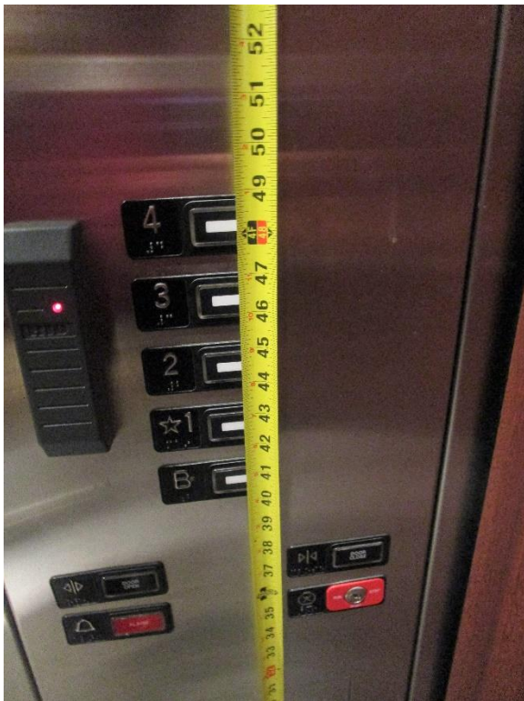
Figure 127. Controls at east elevator at 30 Trinity Street.
