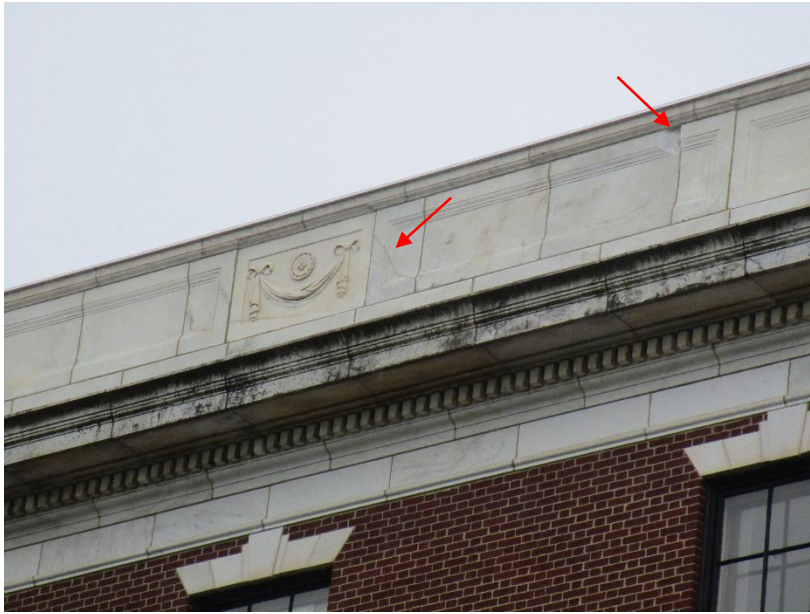
Figure 83. 30 Trinity - Spall and crack at north elevation roof parapet.
