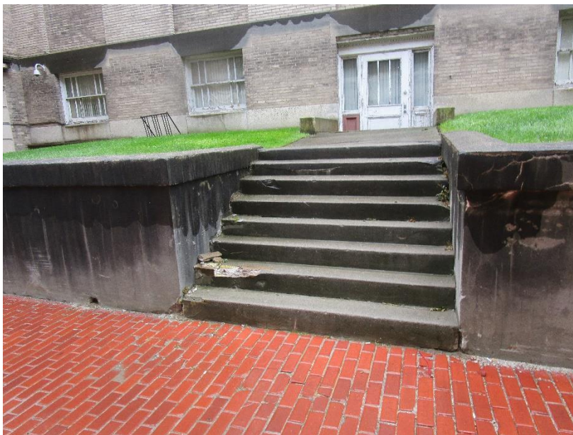
Figure 14. Concrete deterioration at stair and retaining wall at 20 Trinity Street.
