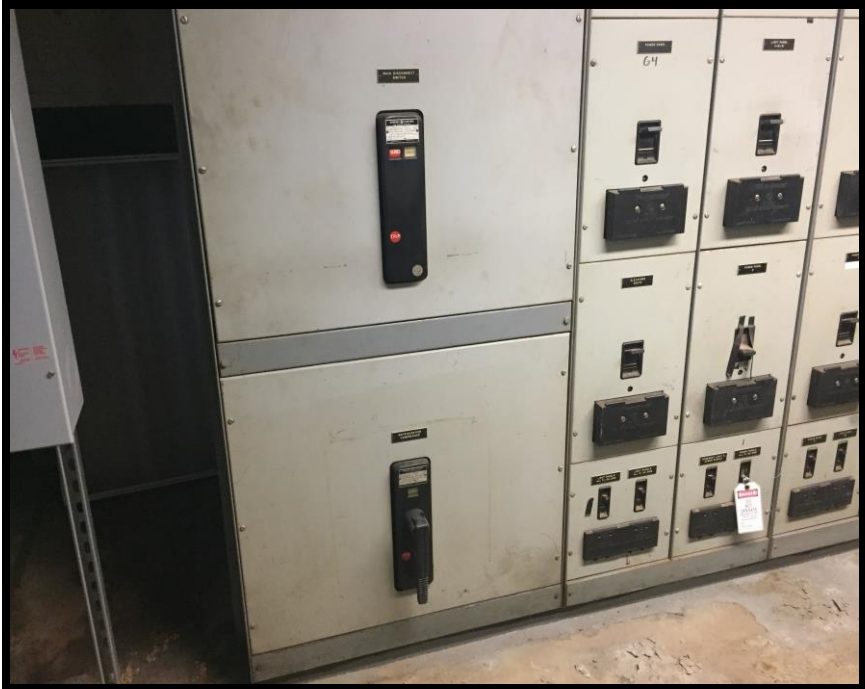
Exhibit "E1" 18-20 Trinity Street Main Switch
