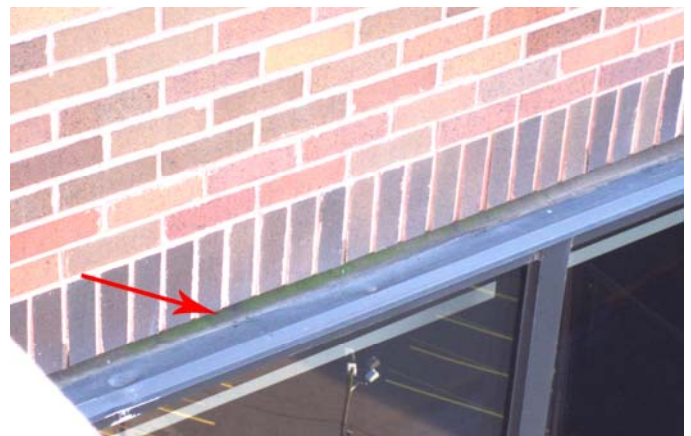
3. Moss Growing on Flashing above Window Sign of Water Pooling and Possible Infiltration (18 th floor "zipper")
