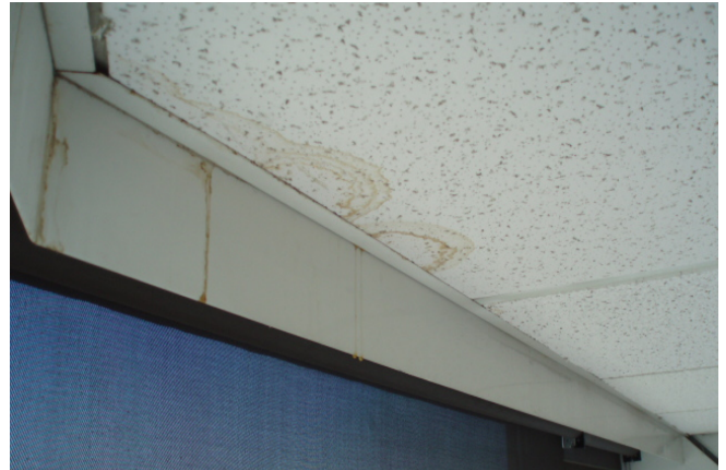
4. Visible Stains on Ceiling Tile & Fascia (18 th floor)
