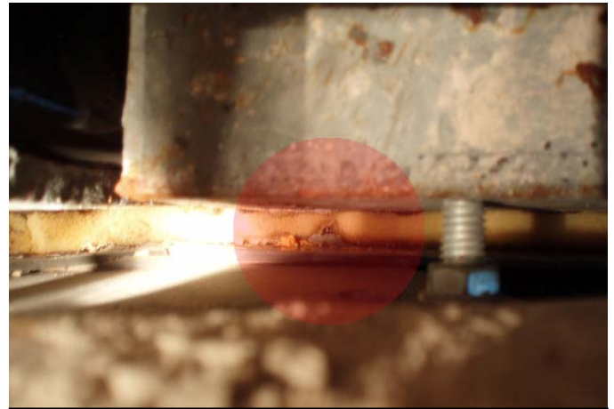
7. Water Leaking Thru Sealant and Backer Rod (19 th Floor North West Corner Office)
