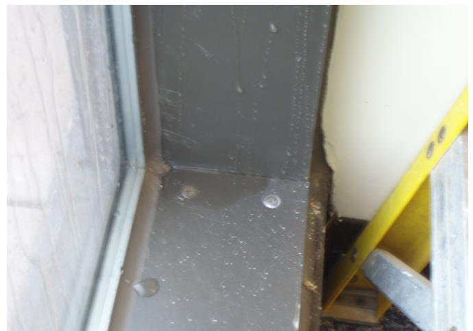
8. Water Pooling at Window Sill (19 th Floor North West Corner Office)
