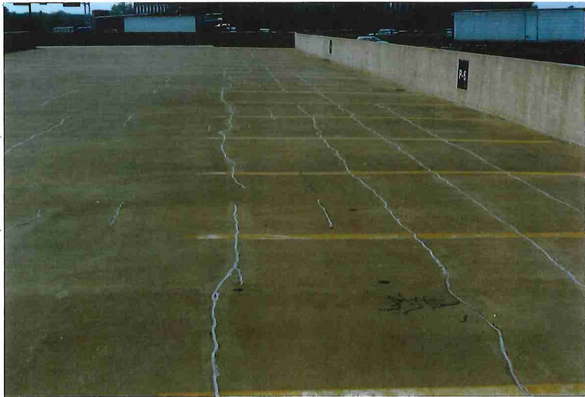
#8 Network of cracks parallel to long axis in garage slab (Level 6).
