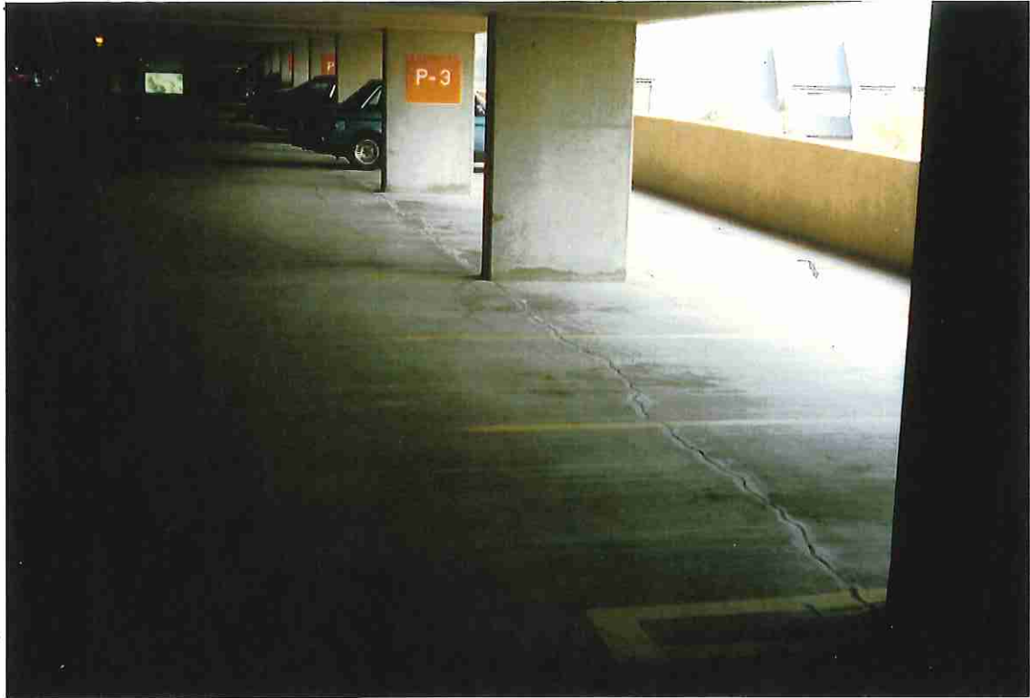
#7 Typical crack running along column line in garage floor slab.
