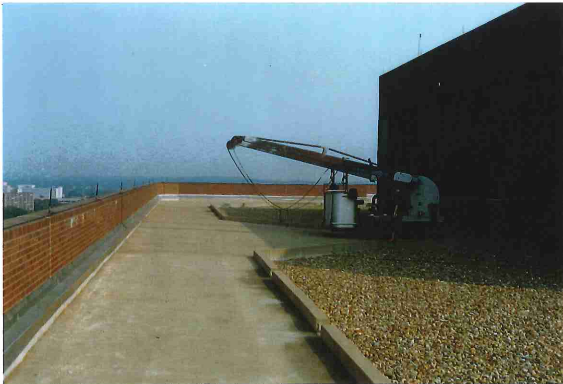
#10 Main roof, looking north from southwest corner, showing concrete runway and window washer rig "garage".
