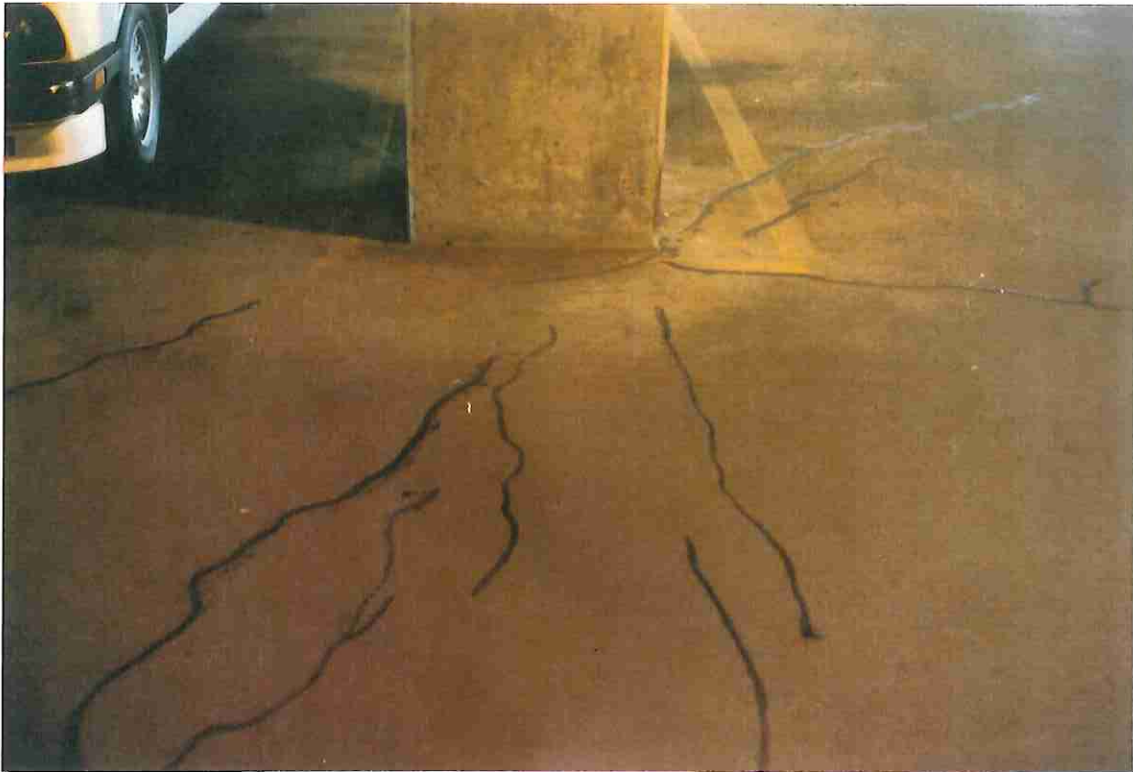
#6 Cracks radiating from column in garage area.
