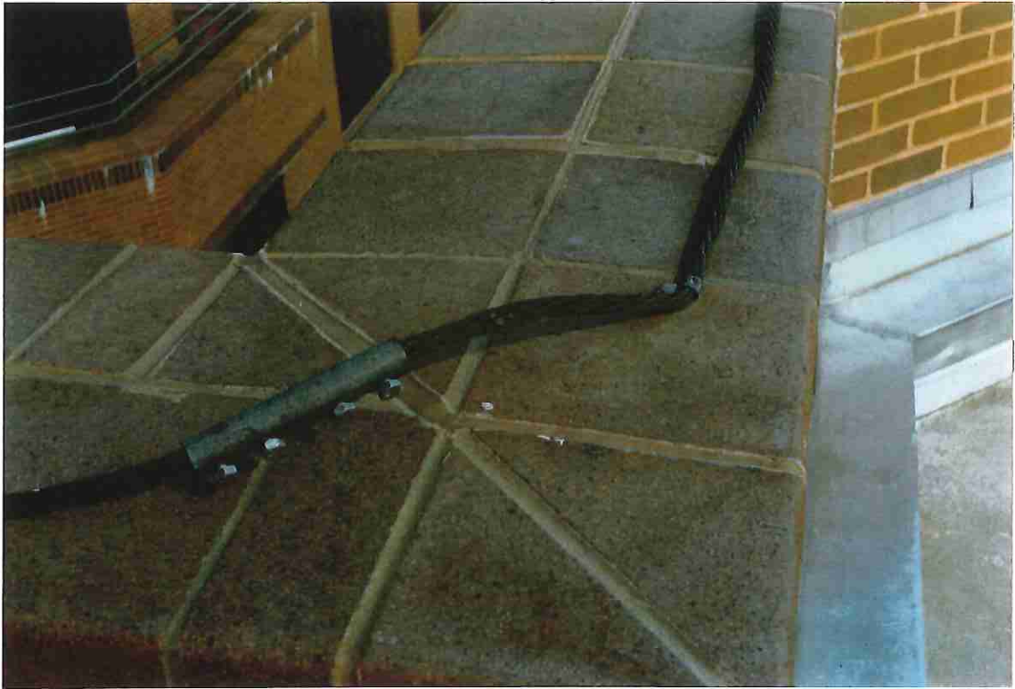
#9 Exposed and spot-repaired mortar joints in typical parapet coping.
