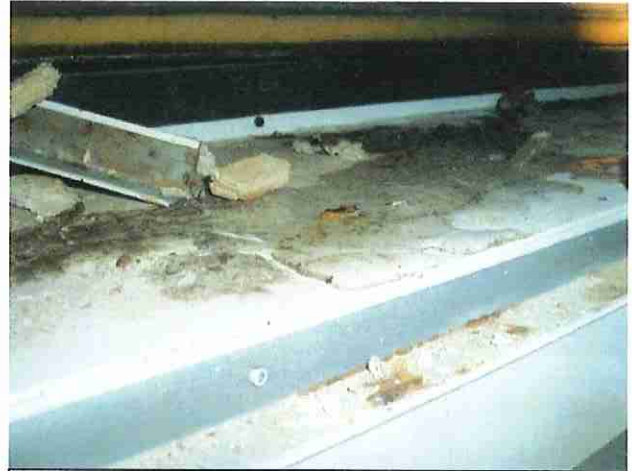
Water Soaking through Backer Rod and Pooling above Window
