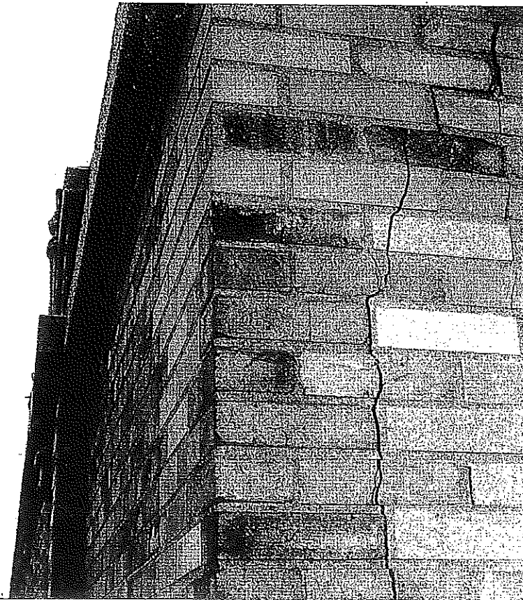
PHOTO #13 MOVEMENT AT TOP OF NORTHEAST CORNER.
