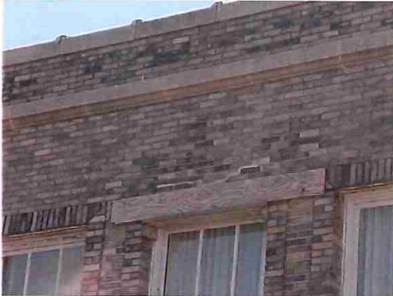
Photo #25: Damaged masonry wall over window
