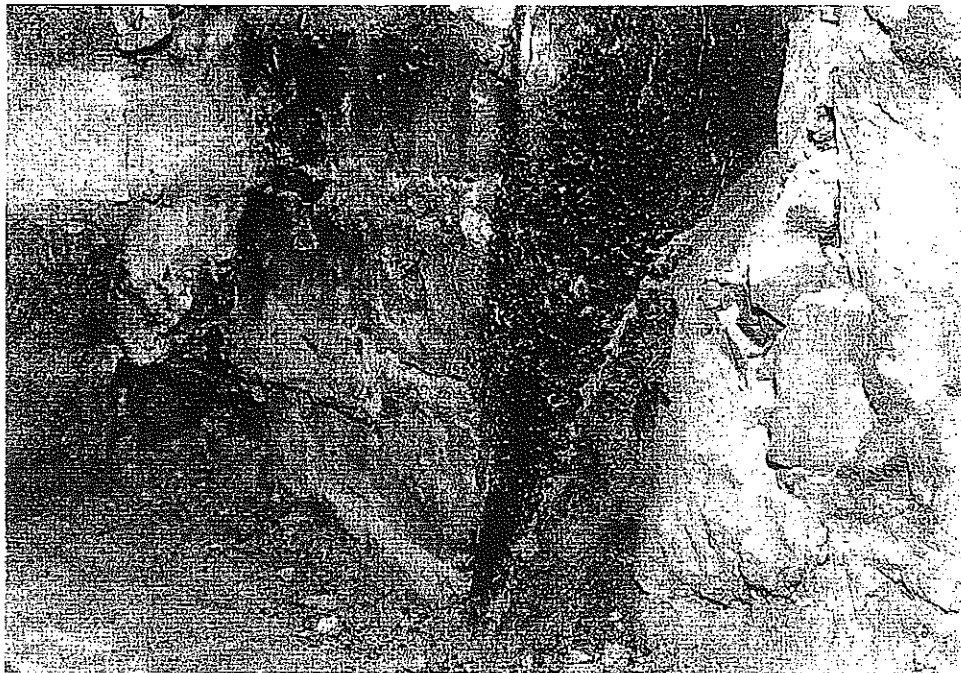
PHOTO#8 PHOTO #7 CLOSE UP SHOWING CORRODED FLANGE
