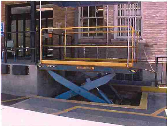
Photo #57: Hydraulic lift at loading dock
