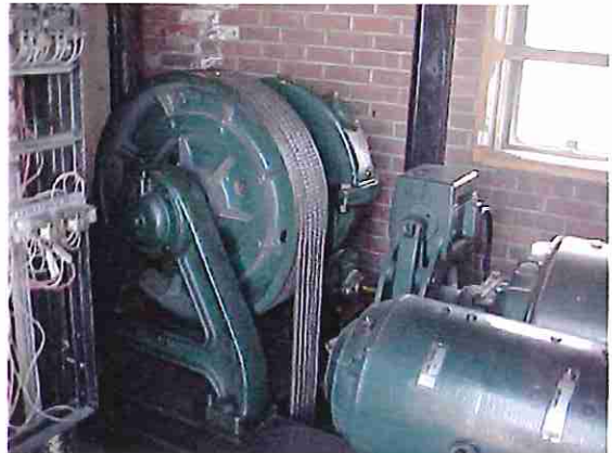
Photo #58: Elevator equipment
