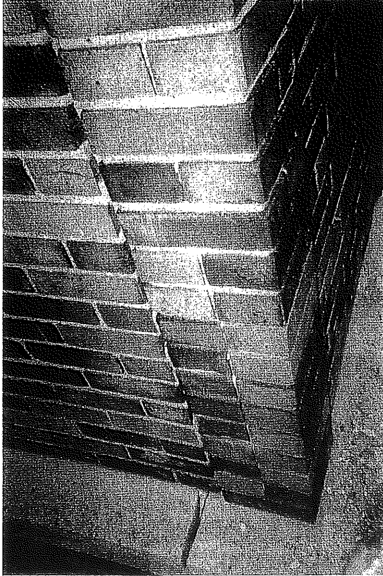
PHOTO #23 SOUTHEAST CORNER OF THE SIXTH FLOOR SHOWS WALL MOVEMENT. GAP IS ABOUT 1". NOTE PRECAST CONCRETE CORNICE LOSING CEMENTING PROPERTIES AND POROUSITY.
