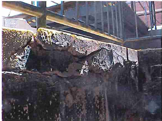
Photo #10: Damaged concrete at exterior concrete stair
