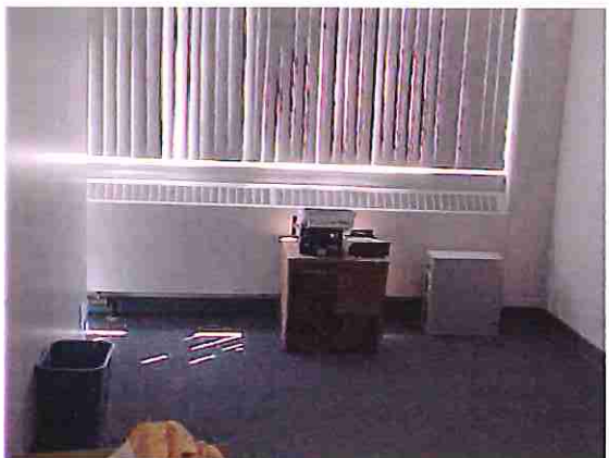
Photo #48: Perimeter heater
