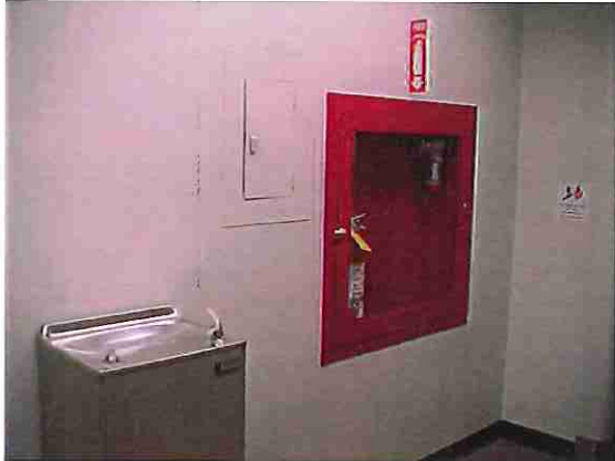
Photo #61: Typical abandoned fire hose station with standpipe in wall
