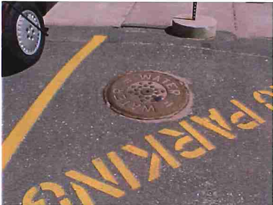
Photo #45: Water meter vault
