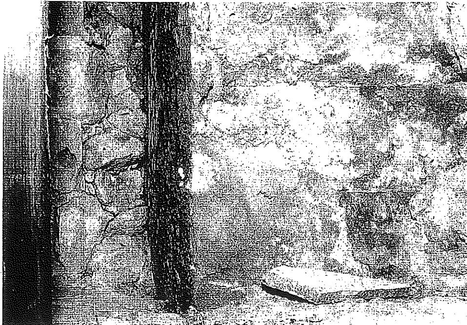
PHOTO# 10 PHOTO#9 CLOSE UP SHOWING CORRODED FLANGE
