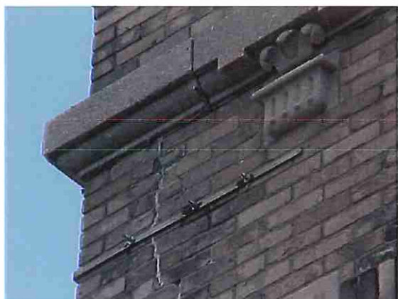
Photo #24: Masonry wall cracking
