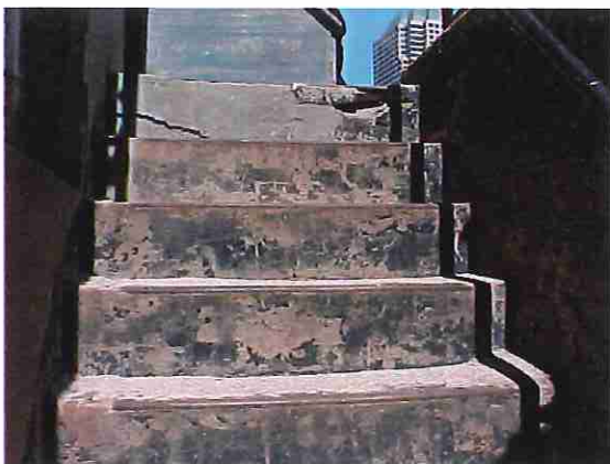
Photo #11: Exterior stair and spalling concrete
