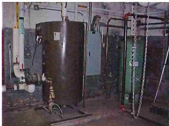
Photo #52: Domestic water heater
