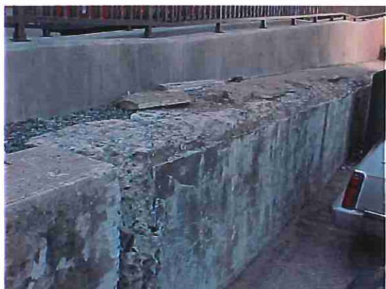
Photo #12: Damaged concrete retaining wall along southern property line
