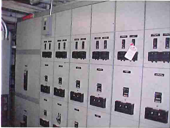
Photo #55: Main electrical switchboard
