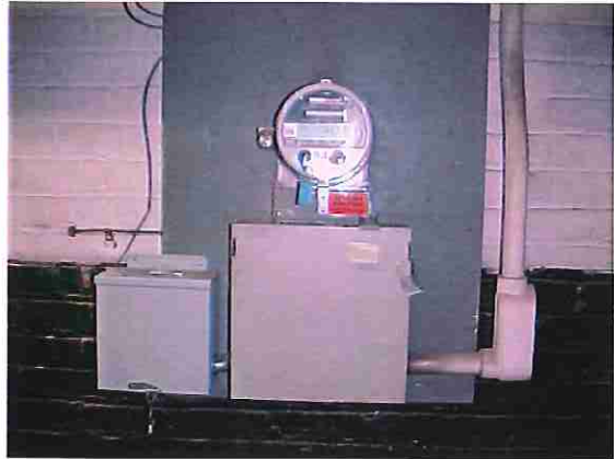
Photo #56: Main electrical meter
