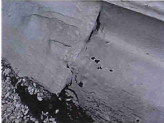
Photo #19: Damaged built-up roof flashing
