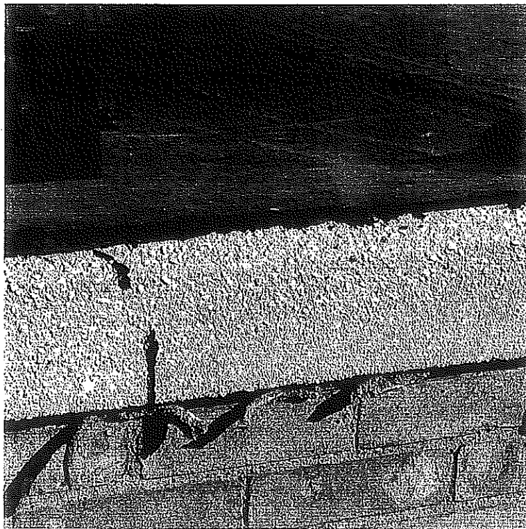
PHOTO -H PRECAST CONCRETE COPING. NOTE: CAULKING IS MISSING
