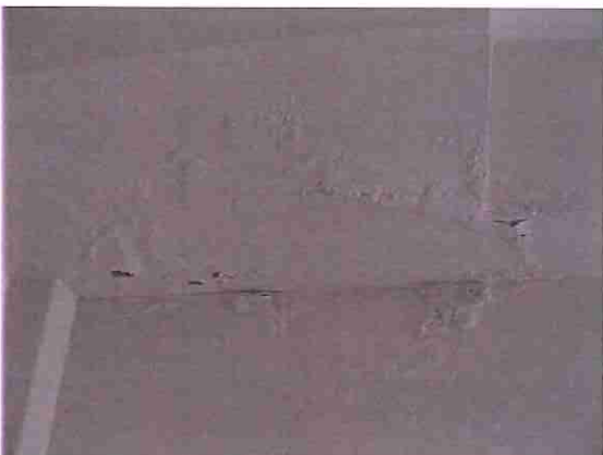
Photo #29: Water infiltration at interior wall
