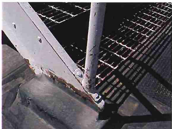
Photo #34: Rusted rooftop stair
