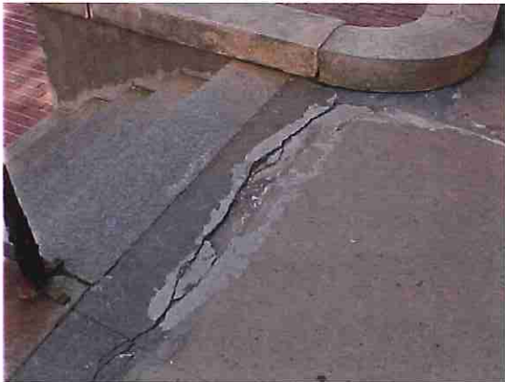
Photo #9: Cracking concrete at exterior steps
