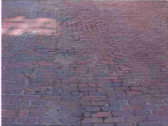
Photo #7: Damaged brick pavers
