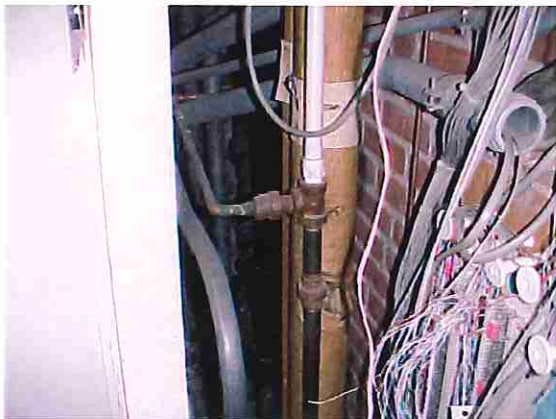
Photo #51: Typical heating and plumbing piping
