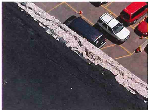
Photo #22: Spalling stone veneer at parapet wall
