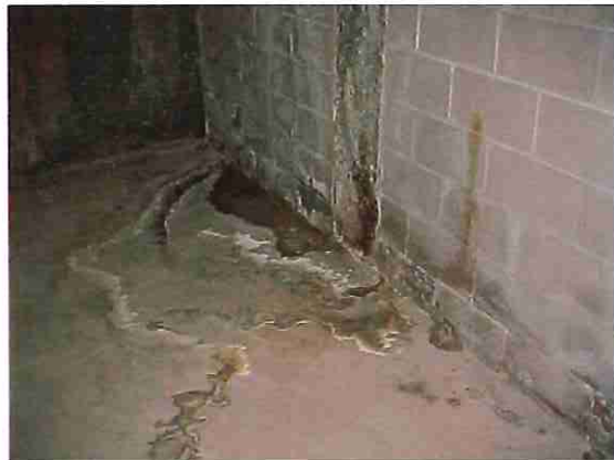
Photo #15: Water staining in basement at rear wall
