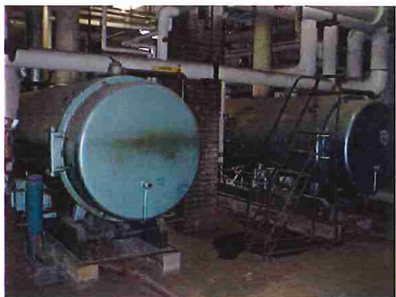
Photo #54: Abandoned boilers
