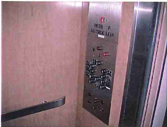
Photo #59: Elevator control panel
