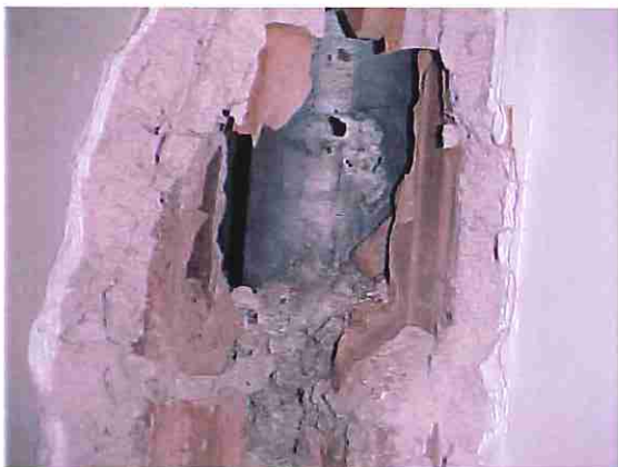
Photo #53: Rusted through galvanized drain lines
