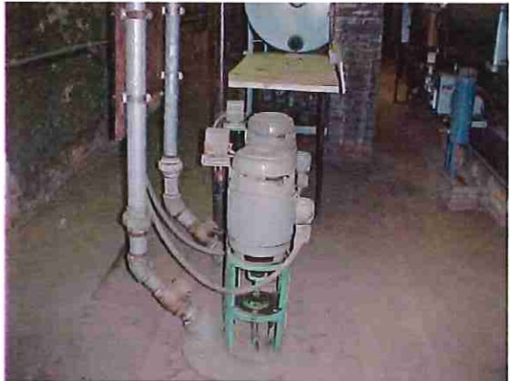
Photo #46: Sump pumps
