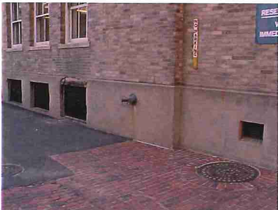
Photo #63: Siamese connections for fire standpipes
