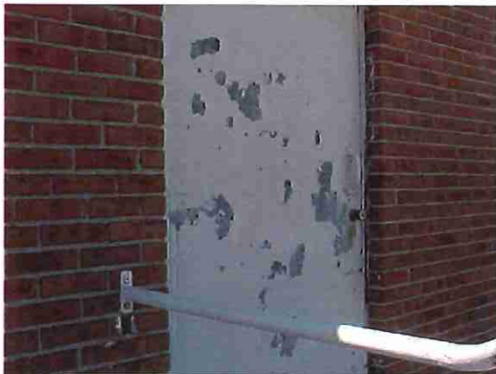
Photo #33: Peeling paint at rooftop door
