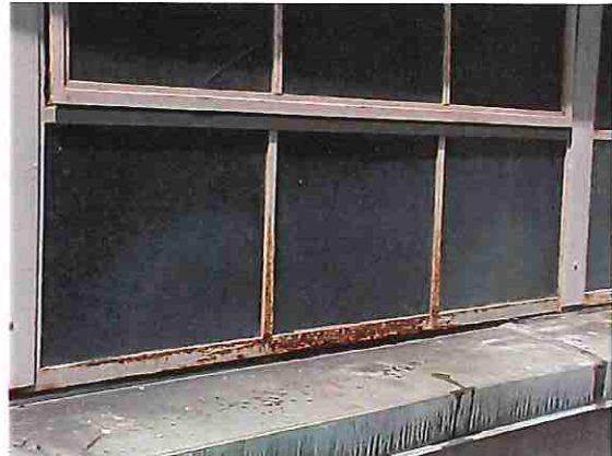
Photo #32: Rusting window frame
