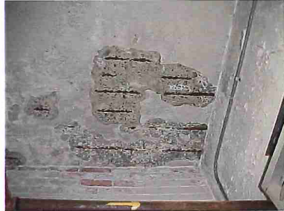
Photo #14: Spalling concrete basement ceiling
