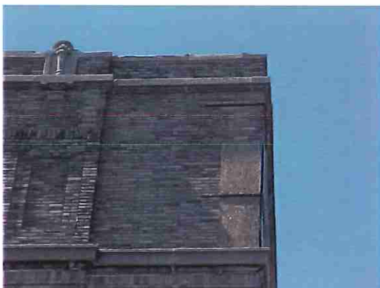
Photo #23: Exterior masonry wall damage and temporary wood bracing
