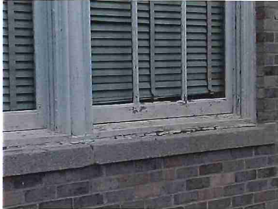
Photo #31: Deteriorating window finish and sealant
