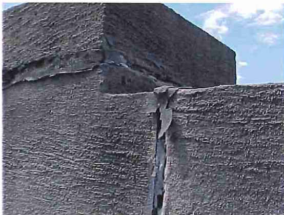
Photo #21: Brittle sealant at roof coping
