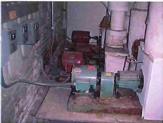
Photo #47: Heated and chilled water circulating pumps
