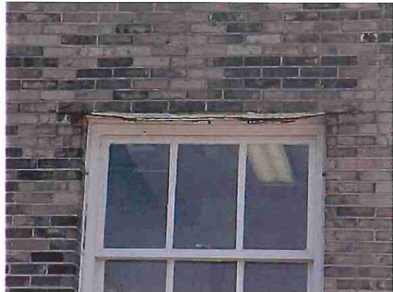
Photo #26: Deteriorating steel lintel at window opening
