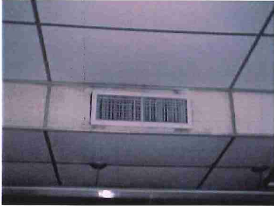
Photo #49: Ceiling conditioned air supply vents
