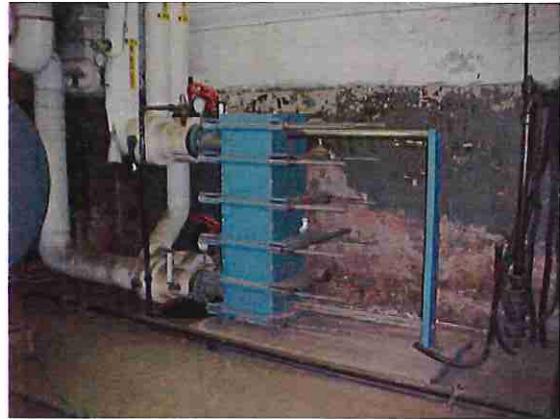
Photo #50: Heating water loop heat exchanger
