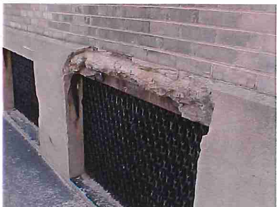
Photo #28: Damaged stone veneer
