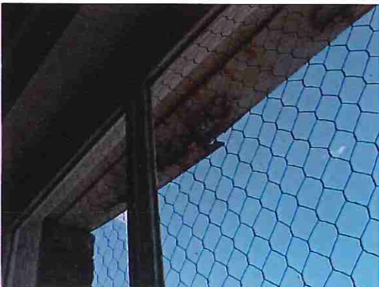
Photo #27: Deteriorating steel lintel
