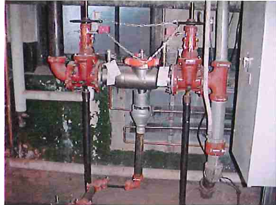
Photo #62: Fire water back flow preventer
