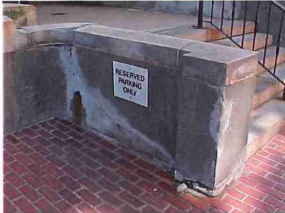
Photo #13: Damaged concrete retaining wall
