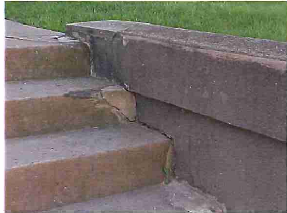
Photo #8: Damaged concrete steps
