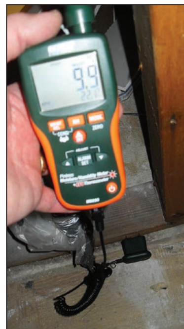
Figure 5: Use of a penetrating (pin-type) moisture meter to verify that wood frame has a water content of less than 15 percent
