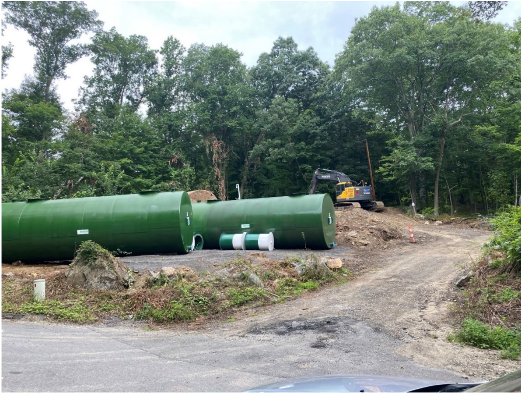
Fig. 3 New water storage tanks which were installed at the Candlewood Knolls Water Authority small public water system to replace aging infrastructure. The project was funded by the DWSRF.
