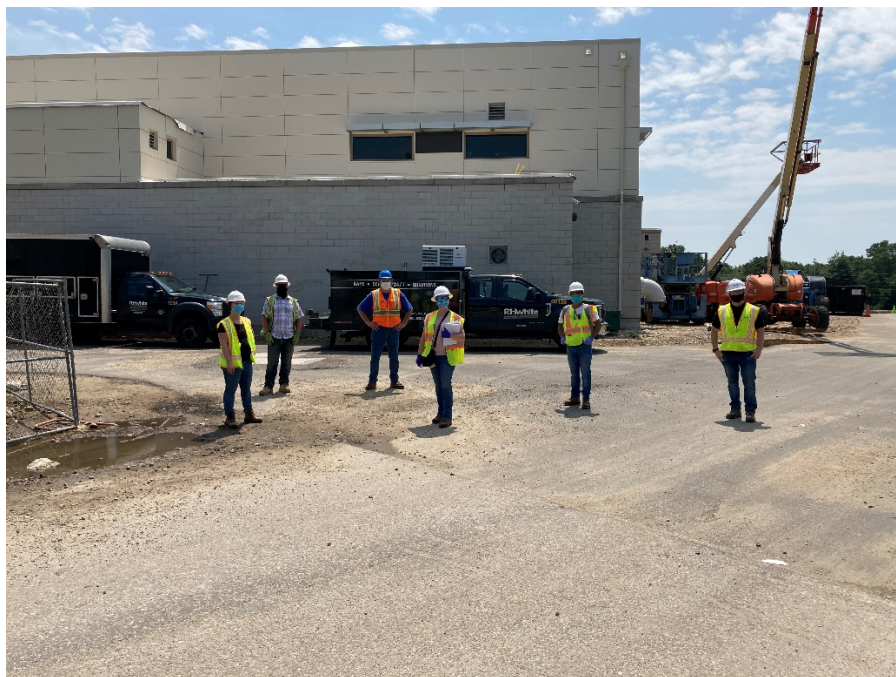
Fig. 2 Multi-year DWSRF Regionalization/Interconnection Project at Groton Utilities WTP site visit during Covid-19 pandemic to put new plant processes online
