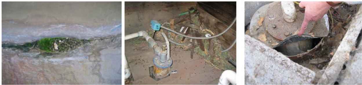
Cracks on a storage tank Rat droppings around the wellhead Seal on wellhead not watertight
