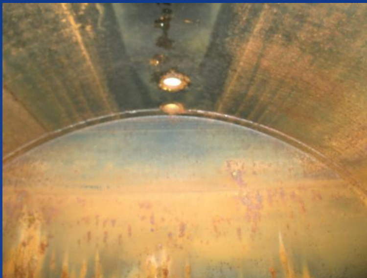
Holes in the roof
