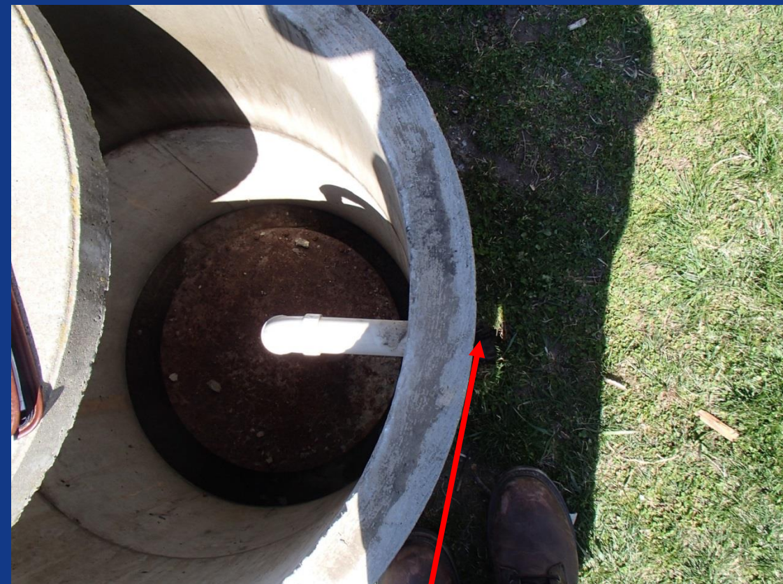
Vent/Overflow Pipe Broken
