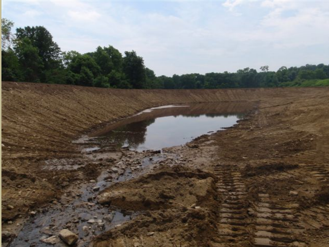
Stormwater and Leachate Collection
