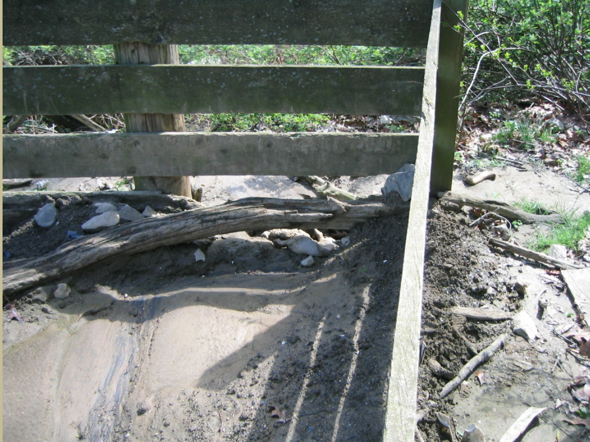
Erosion- Soil Loss
