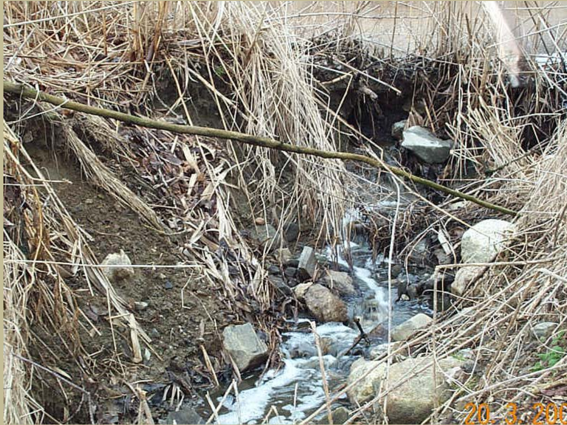
FAILED BERM ON WASTEWATER LAGOON
