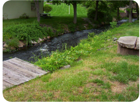
Dug well with cracked cover too close to stream. Photo by DPH.
