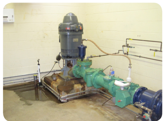
Well pump and meter. Photo by MMI.
