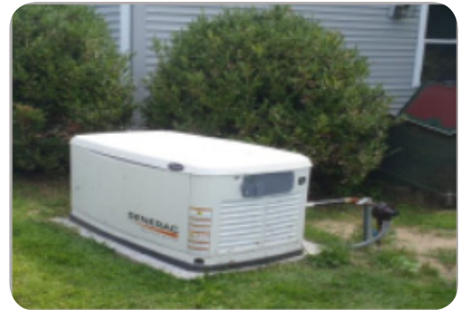
Backup generator. Photo by DPH.
