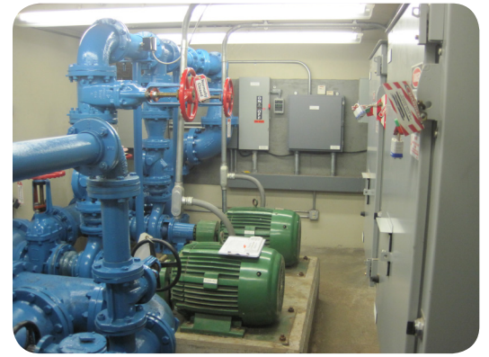
Pump station. Photo by MMI.
