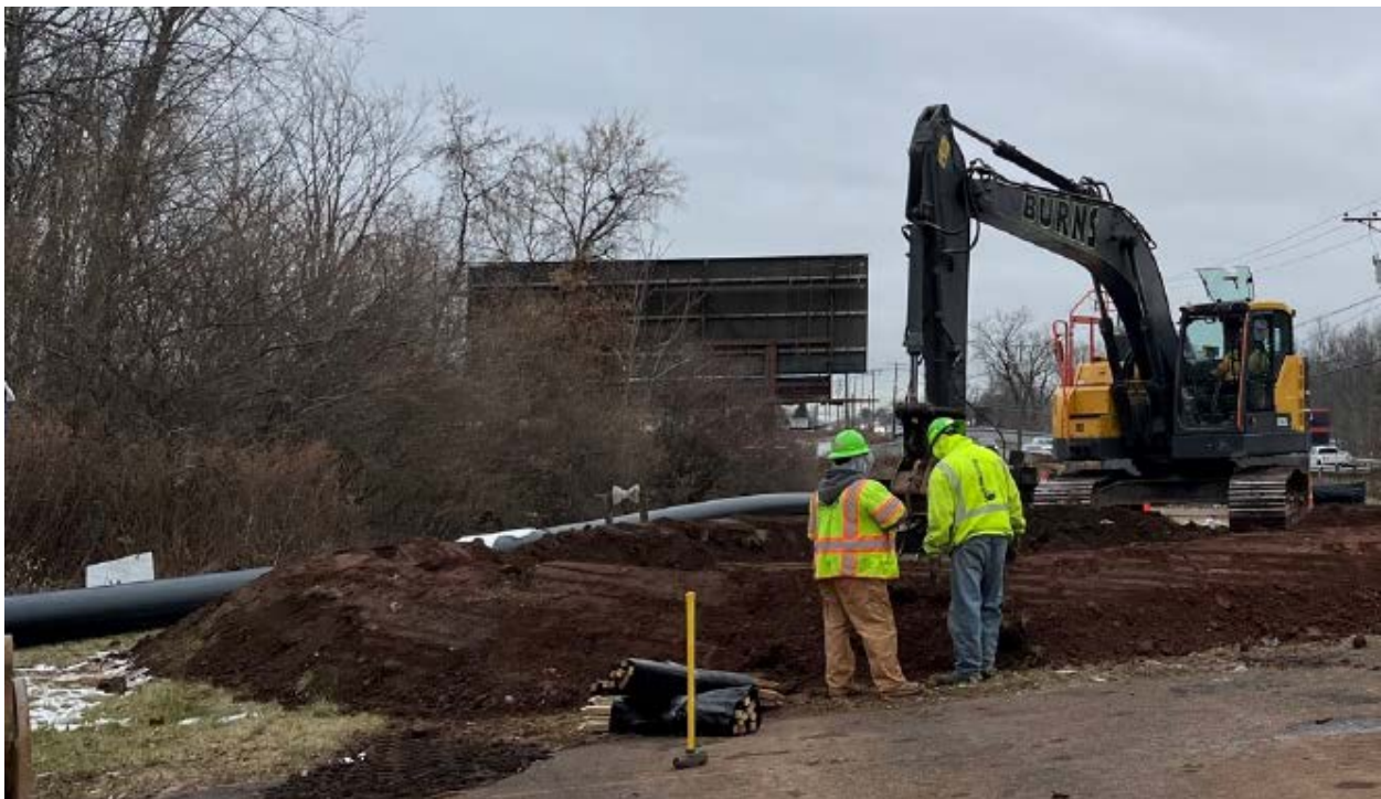
Fig. 6 Water transmission main was installed in the Berlin Water Control Commission small water system to replace aging infrastructure. The project was funded by the DWSRF.
