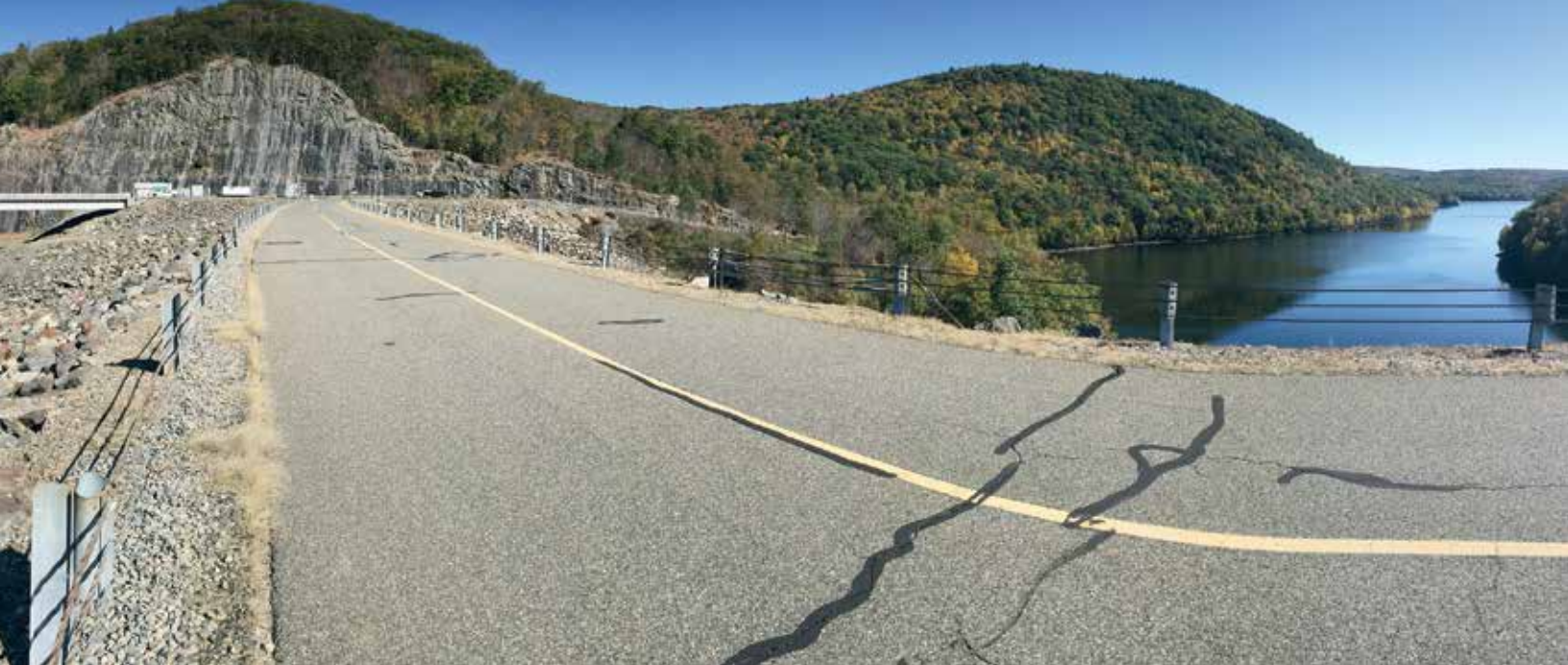
A 180-degree view from the middle of the Army Corps of Engineers Dam (est. 1969) at Colebrook River Lake, Colebrook. Looking left (pg. 18) and to the North is Colebrook River Lake and its gate house. To the right (pg. 19) and south is the West Branch Reservoir. The management of these two waterbodies is complex, balancing legal requirements of minimum flows, water rights (riparian) for downstream entities established in the early 1800s, hydropower, protecting life and property from floods, and managing fish habitat. In addition, these two waterbodies provide the public with recreational boating and fishing opportunities.
