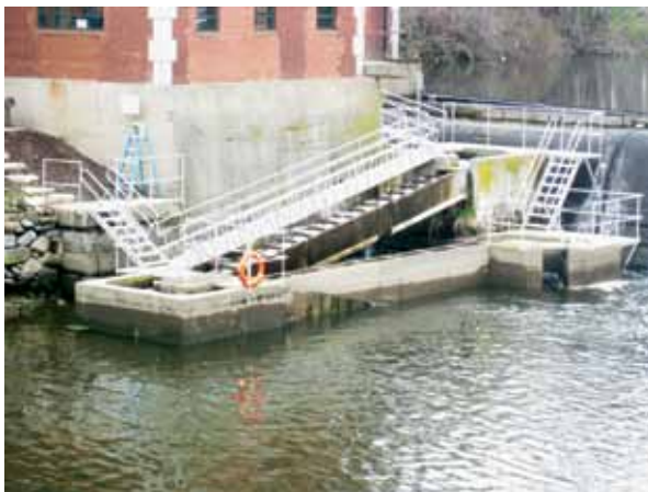
The Mianus Pond Fishway on the Mianus River in Greenwich is a steppass fishway with two resting pools. It has annually passed 90,000 herring in recent years.
