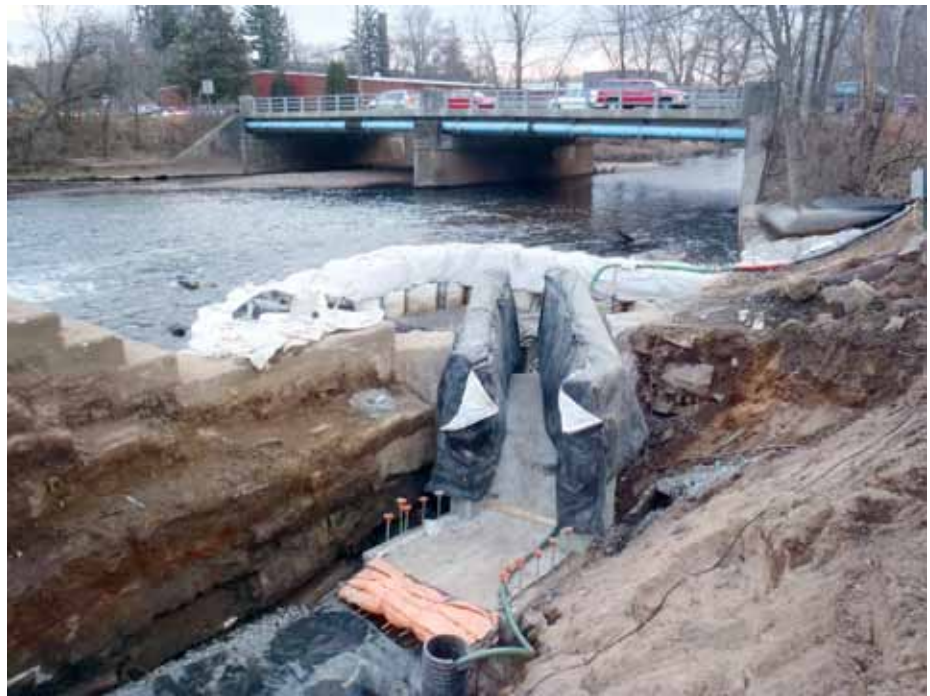
The Wallace Dam Fishway on the Quinnipiac River in Wallingford is currently under construction. The dam is to the left of the photo.
