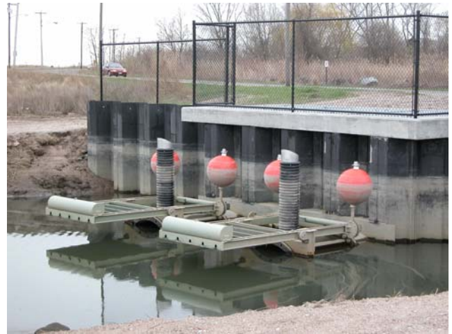
Self-regulating tide gates (SRTs) increase tidal flow without causing upstream flooding. Photo courtesy of Roger Wolfe.
