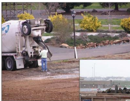
Figure 1. Chute washwater being dumped on the ground
