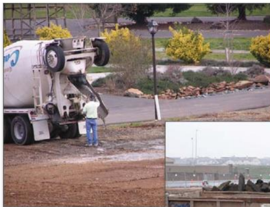
Figure 1. Chute washwater being dumped on the ground
