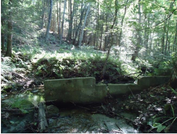
Photo 71: Abandoned diversion structure and dam
