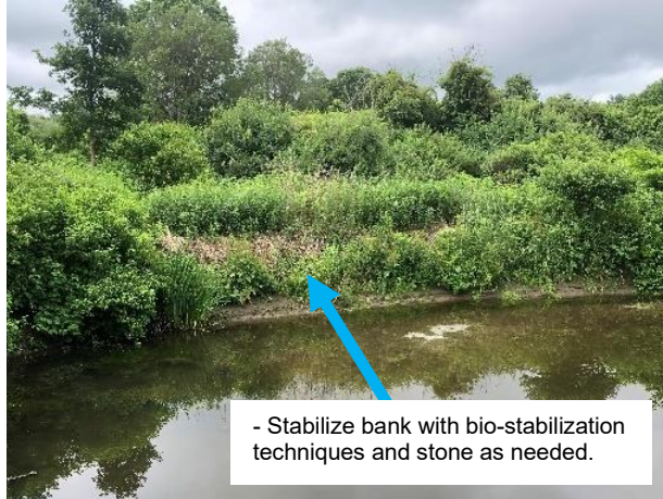
Photo 4-10: Eroding banks at LLC5.
