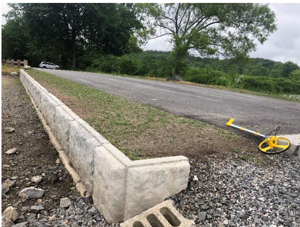
Photo 7-4: Grass strip and concrete blocks along the road to the boat launch.
