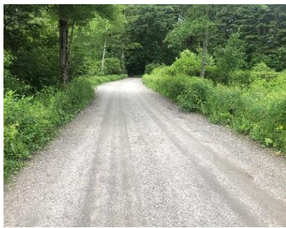
Photo 1-1: Section of Whitehall Road that floods multiple times per year.
