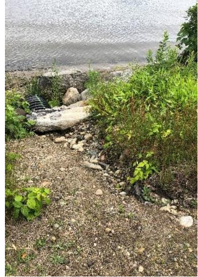
Photo 8-3: Erosion around top of outfall on North Shore Road.
