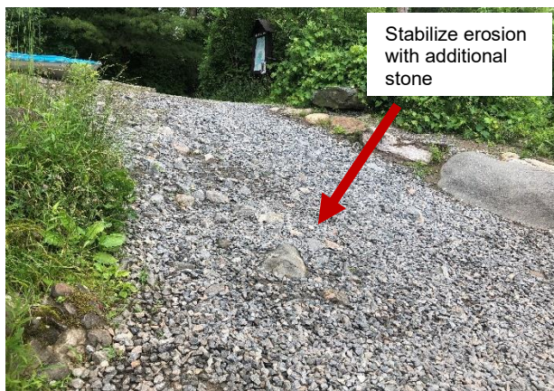
Photo 3-1: Erosion of gravel on east side of boat launch
