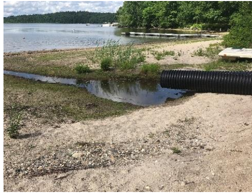
Photo 13-2: Sandy Beach with perched outlet pipes discharging to the lake via an eroded gully.
