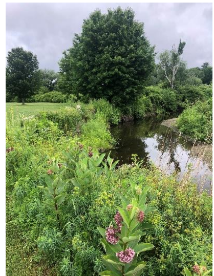
Photo 4-14: Bank beginning to undercut at LCC6.
