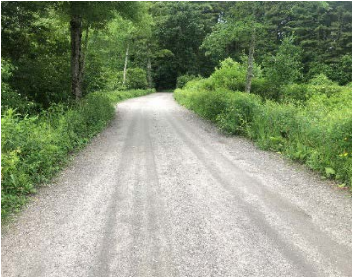
Photo 1-1: Section of Whitehall Road that floods multiple times per year.
