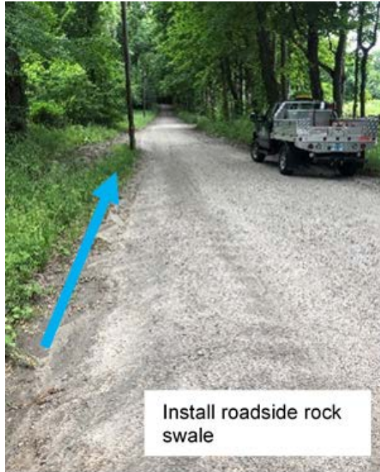
Photo 6-1: Roadside erosion from Town Hill Road.
