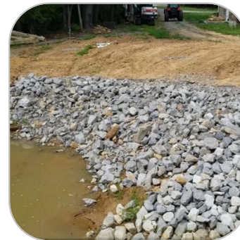
Stone Slope Protection
