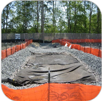
Pumping Settling Basin
