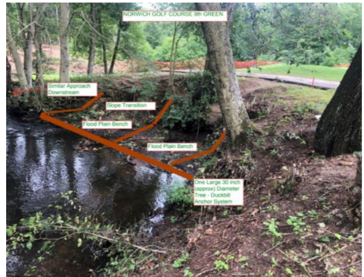
Figure 19: Image of streambank erosion from site visit at Norwich Golf Course. Image courtesy of ECCD.
