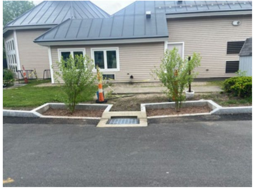
Figure 10: Tree filter installed in school parking lot. Image courtesy of FRWA.
