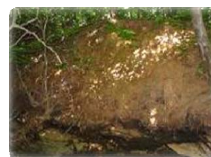
Severe slope failure, Miner Brook, Middletown, CT
