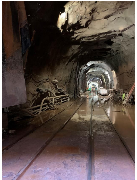
Inside the South Hartford Conveyance and Storage Tunnel
