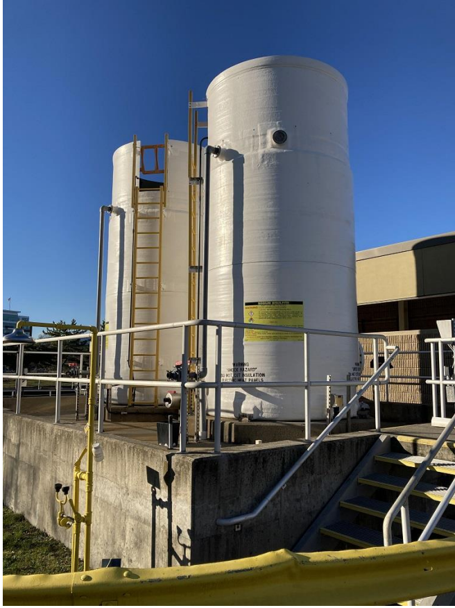
Sodium Bisulfite Tanks
