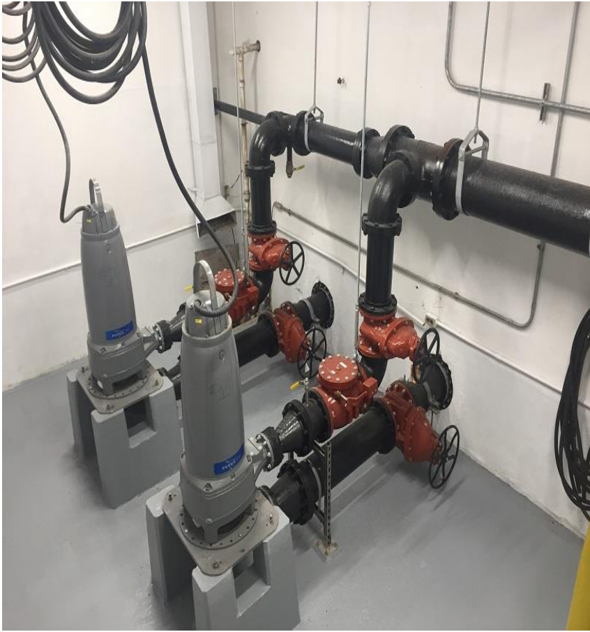
New Flygt Dry Pit Pumps and Piping
