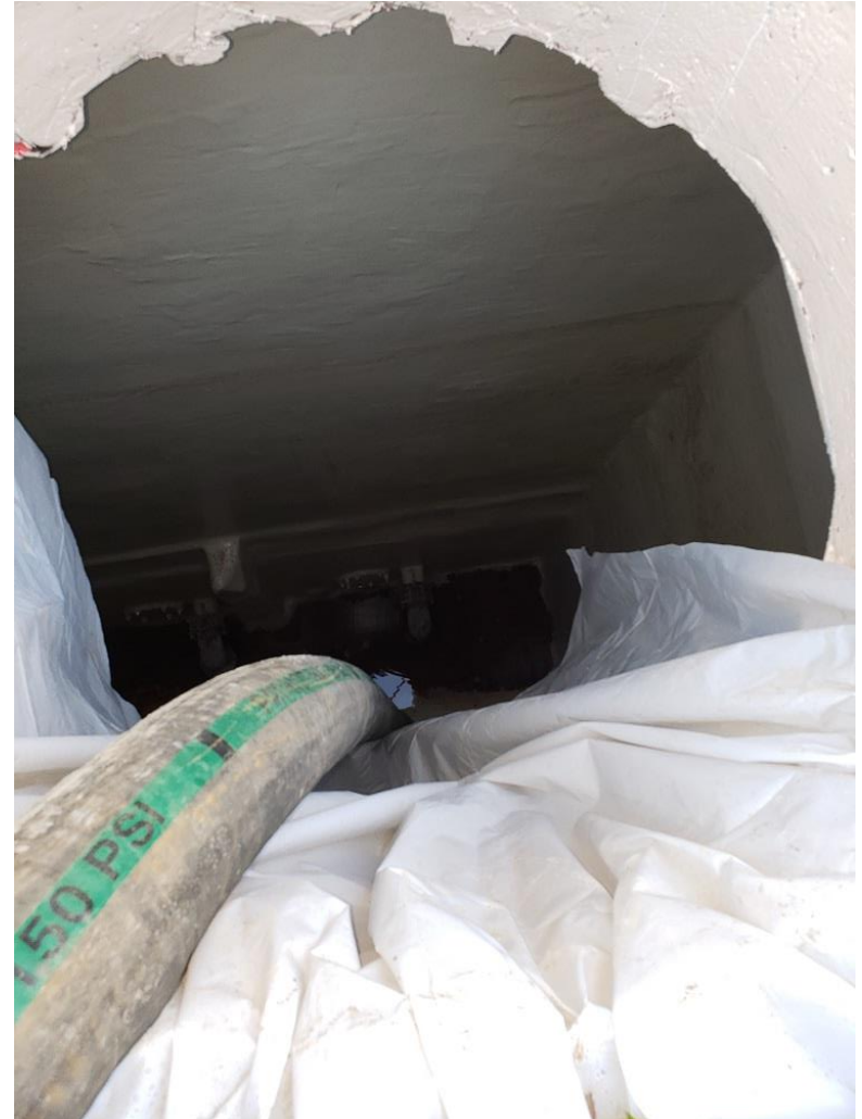
Marvin Beach PS Wet Well Coating
