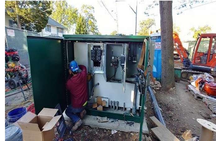
New Electrical and Pump Controls
