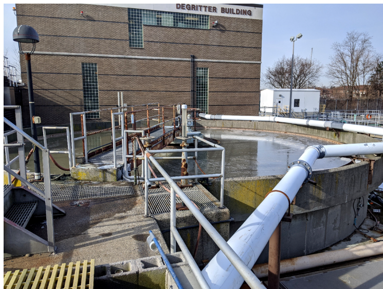
Figure 4.2-7 Gravity Thickener Tank #2 and Mixed Sludge Gravity Line
