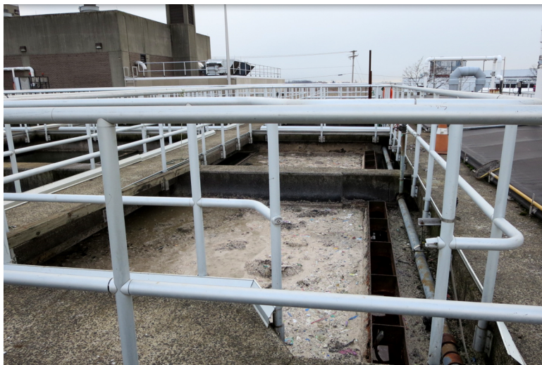
Figure 4.3-3 Inoperable Primary Scum Collection Troughs and Accumulated Scum
