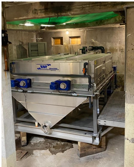
Figure 4.2-8 Rotary Drum Thickener Skid
