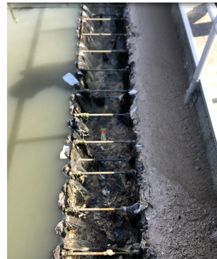
Figure 4.2-4 Scum Accumulation on Primary Clarifier Weirs
