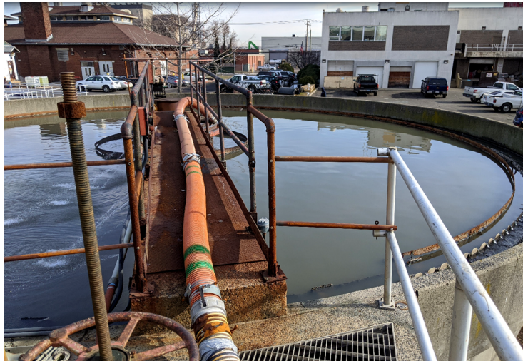
Figure 4.2-6 Gravity Thickener Tank #1 (temporary WAS pipe on walkway)
