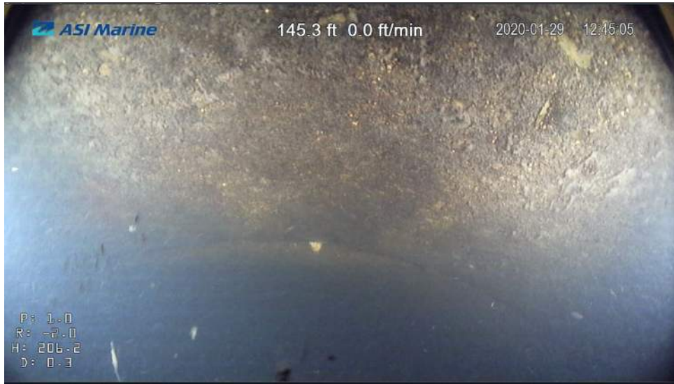
Image 4.1.1B-6: Image of crown and joint ahead 145 feet downstream of Manhole 3.
