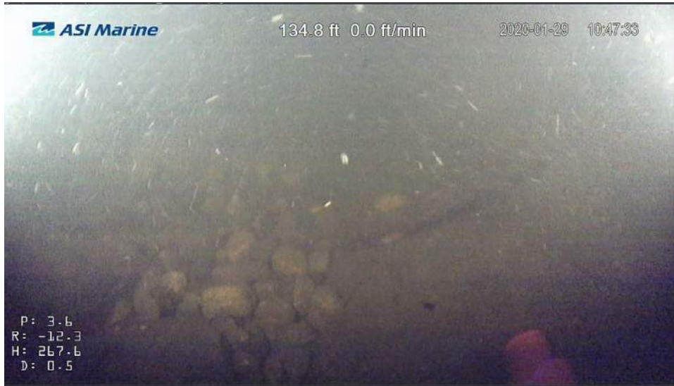
Image 4.1.1A-3: Debris on invert at 135 feet downstream of Manhole 1.
