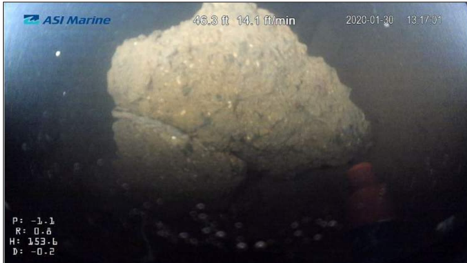
Image 4.2.1-1: Debris on invert 46 feet downstream of Access Point 1.
