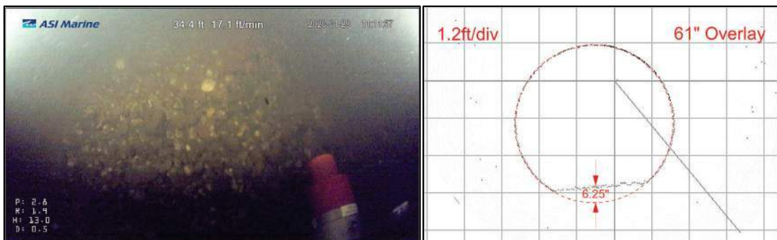
Figure 10: Image of debris on invert at 34 feet upstream of Manhole 1 (left); Profile of rock debris at 116 feet upstream of Manhole 1 (right)
