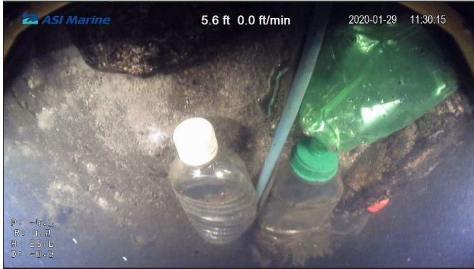
Image 4.1.1A-5: Floating debris and line at crown 5 feet upstream of Manhole 1.
