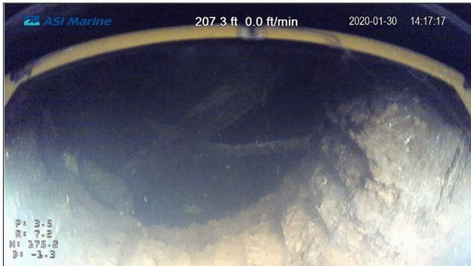
Image 4.2.1-14: Opening in crown 207 feet downstream of Access Point 1.
