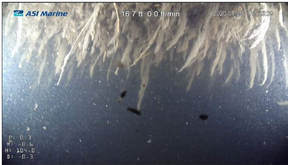
Image 4.1.1A-8: Biofouling on crown in plant bypass conduit 17 feet east of Manhole 1 in plant bypass.
