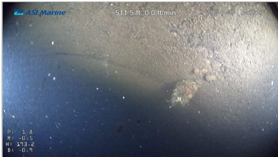
Image 4.2.1-20: Protrusion at crown 511 feet downstream of Access Point 1.
