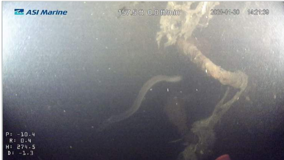
Image 4.2.1-9: Ladder rungs at manhole access 157 feet downstream of Access Point 1.
