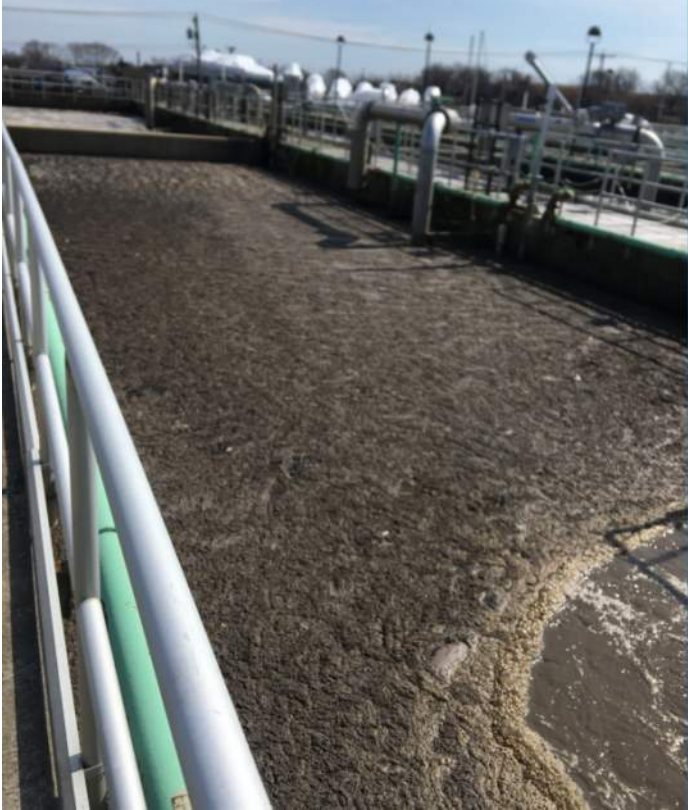
Figure 10. Floating Scum in West Side WWTP's BNR Basins
