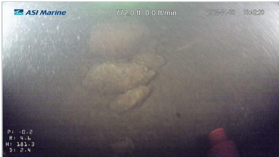
Image 4.2.1-28: Debris on invert 772 feet downstream of Access Point 1.
