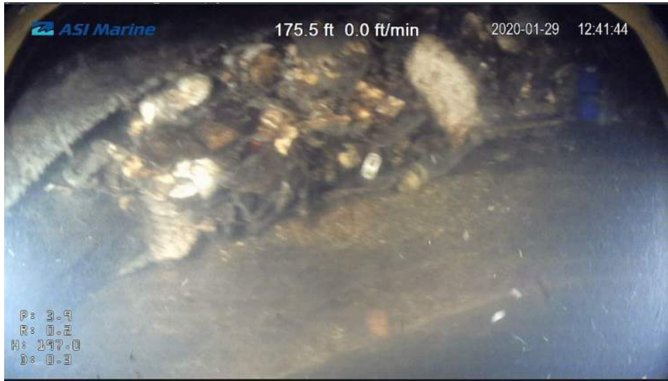
Image 4.1.1B-8: Floating debris at crown 176 feet downstream of Manhole 3.
