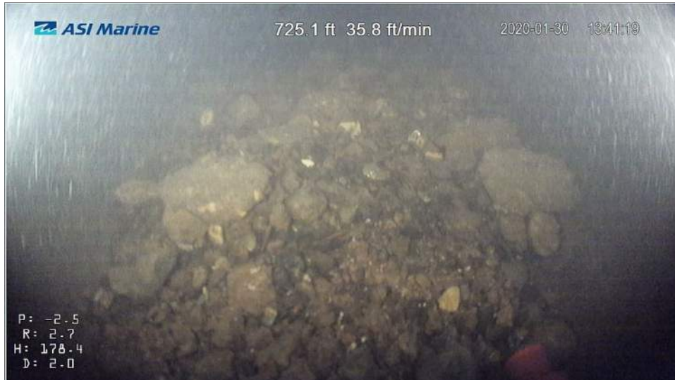
Image 4.2.1-27: Rock debris on invert 725 feet downstream of Access Point 1.
