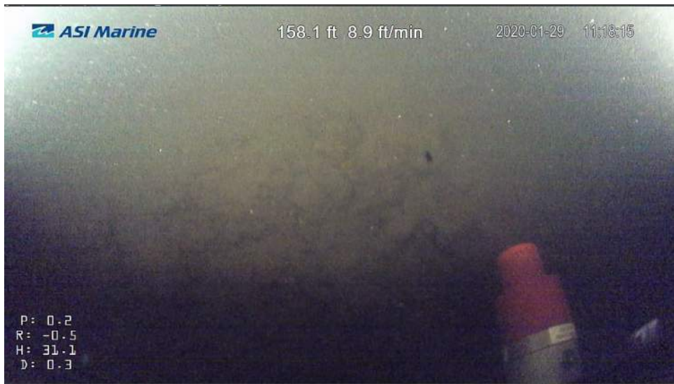
Image 4.1.1A.16: Sediment on invert 158 feet upstream of Manhole 1.
