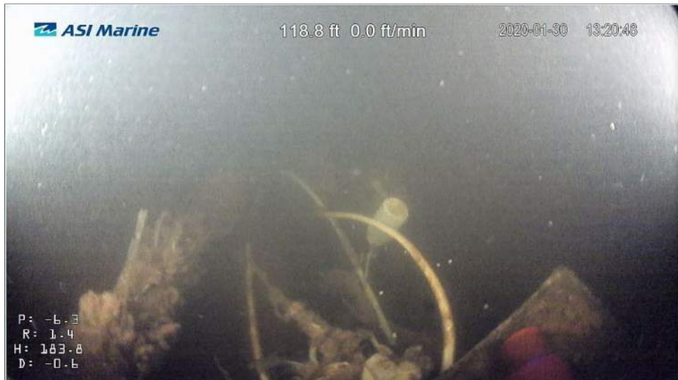
Image 4.2.1-6: Debris and possibly instrumentation on invert 121 feet downstream of Access Point 1.
