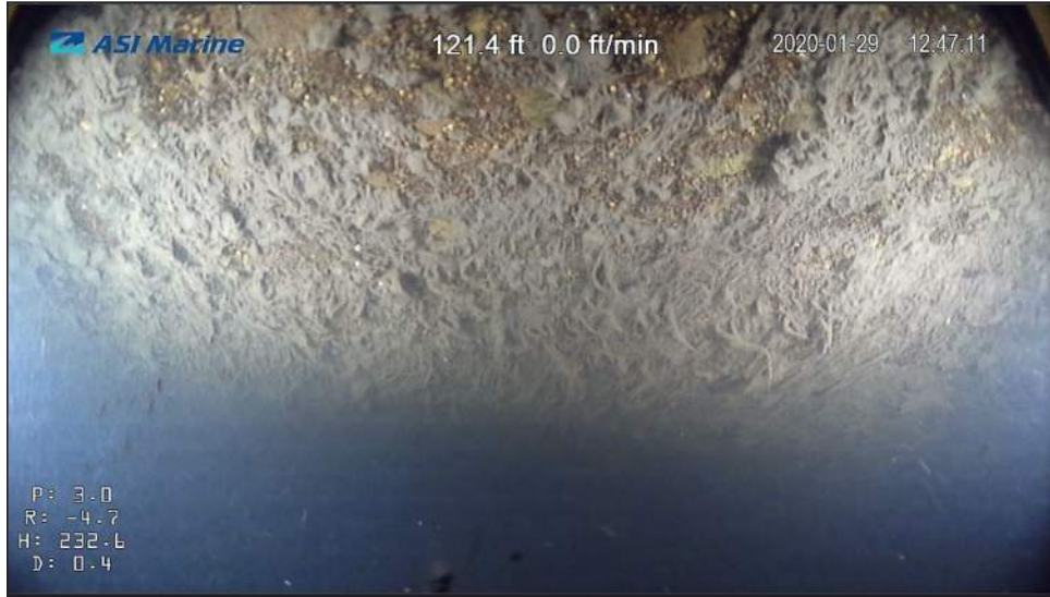
Image 4.1.1B-5: Image of crown 121 feet downstream of Manhole 3.
