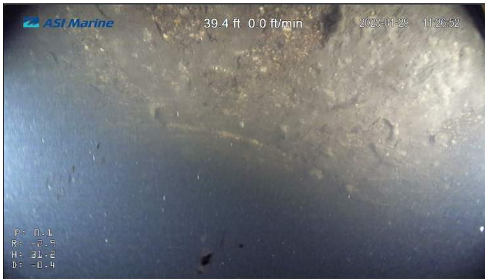
Image 4.1.1A-10: Image of joint at crown 39 feet upstream of Manhole 1.
