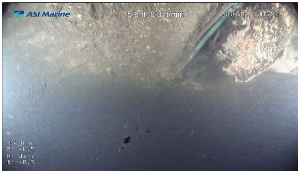
Image 4.1.1A-4: Exposed aggregate and line at crown 5 feet upstream of Manhole 1.
