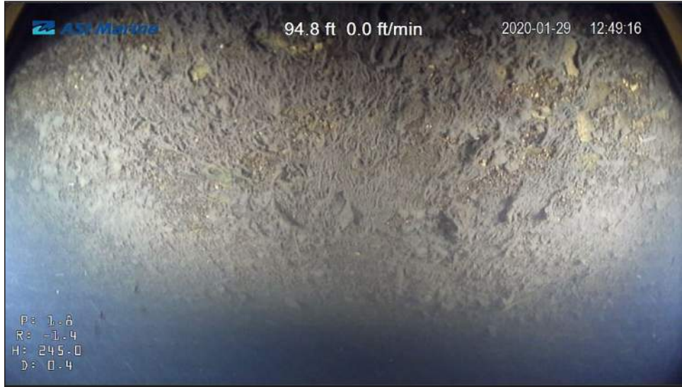
Image 4.1.1B-3: Image of crown 95 feet downstream of Manhole 3.
