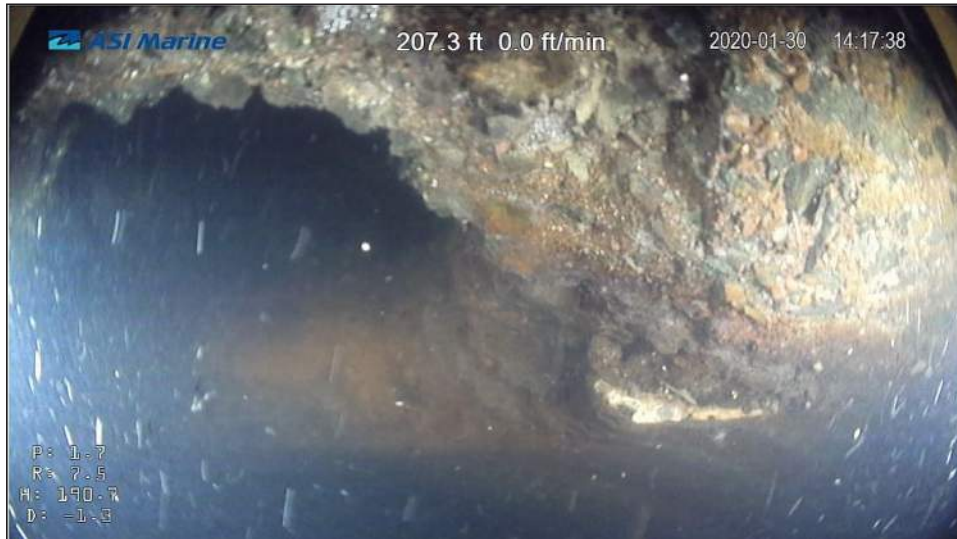
Image 4.2.1-13: Opening in crown 207 feet downstream of Access Point 1.
