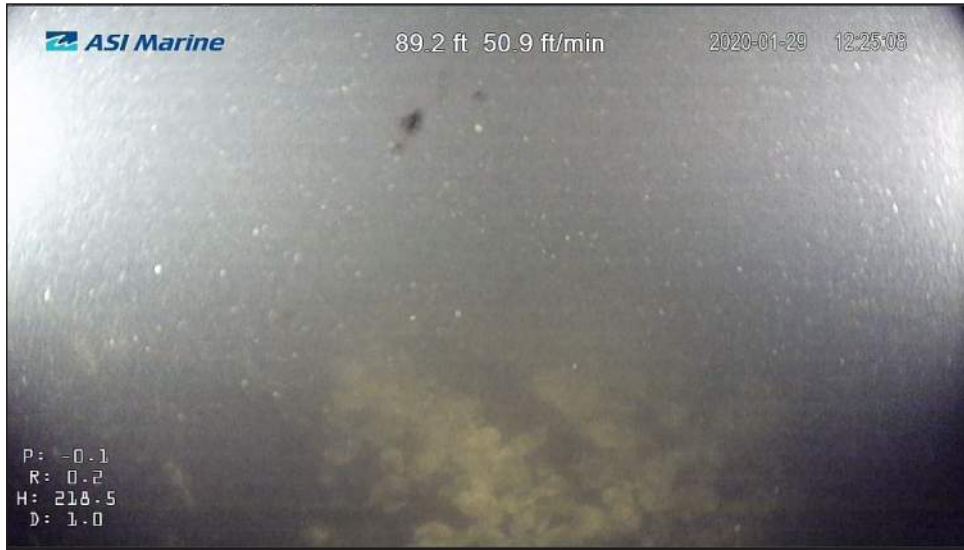
Image 4.1.1B-2: Debris on invert 89 feet downstream of Manhole 3.
