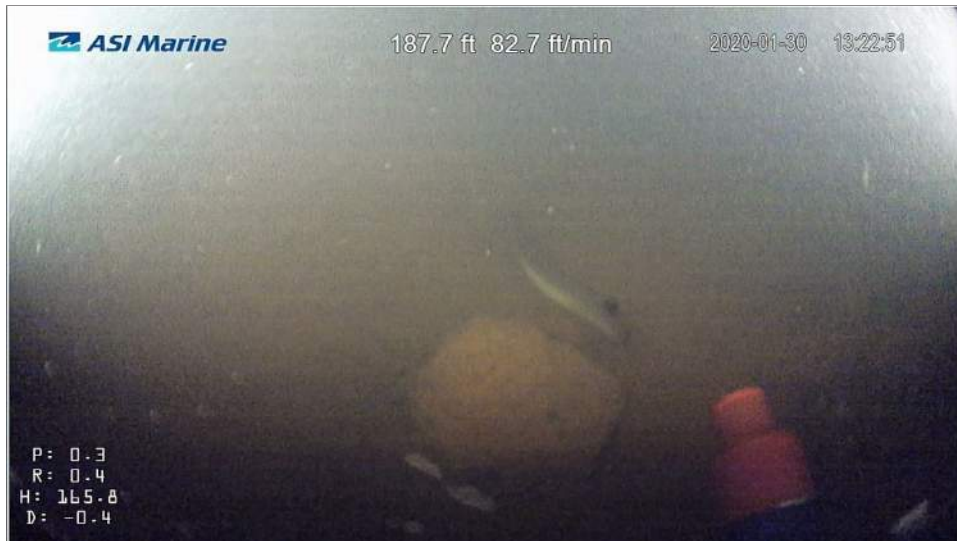
Image 4.2.1-12: Debris on invert 188 feet downstream of Access Point 1. Debris on invert.
