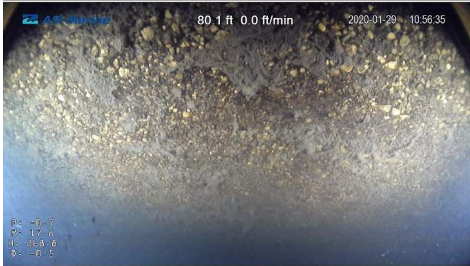
Image 4.1.1A-1: Image of crown 80 feet downstream of Manhole 1.
