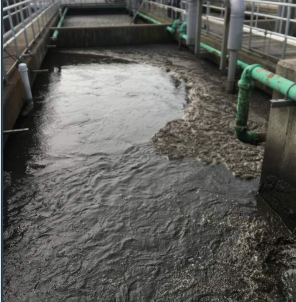
Figure 10. Floating Scum in Aeration Tanks at the East Side WWTP
