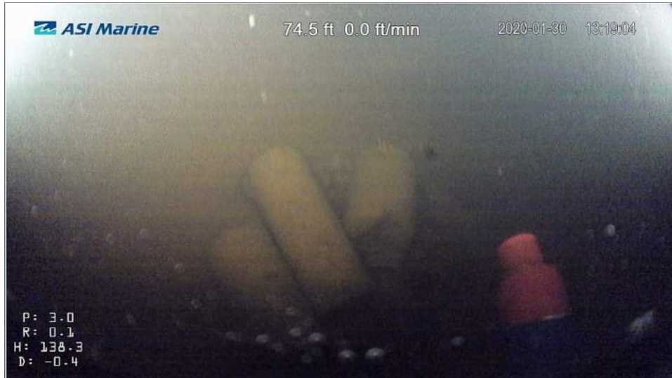
Image 4.2.1-3: Debris on invert 74 feet downstream of Access Point 1.
