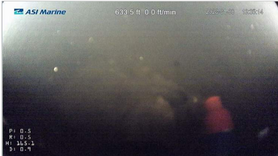
Image 4.2.1-23: Debris on invert 634 feet downstream of Access Point 1.
