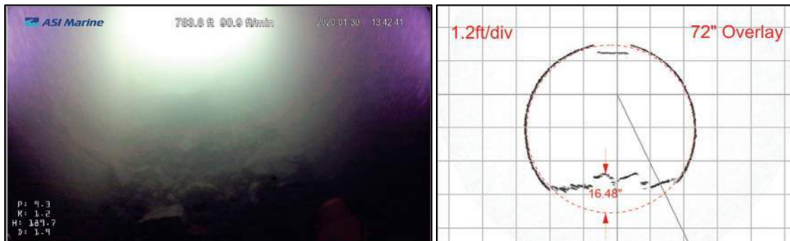
Figure 22: Image of outlet at 784 feet (left); Profile image of debris at 786 feet (right)
