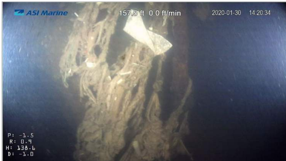
Image 4.2.1-10: Biofouling on ladder 157 feet downstream of Access Point 1.
