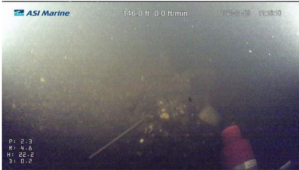
Image 4.1.1A.15: Debris on invert 146 feet upstream of Manhole 1.
