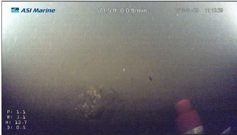
Image 4.1.1A-12: Debris on invert 71 feet upstream of Manhole 1.
