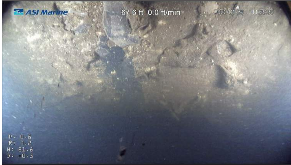
Image 4.1.1A-11: Image of crown 68 feet upstream of Manhole 1.
