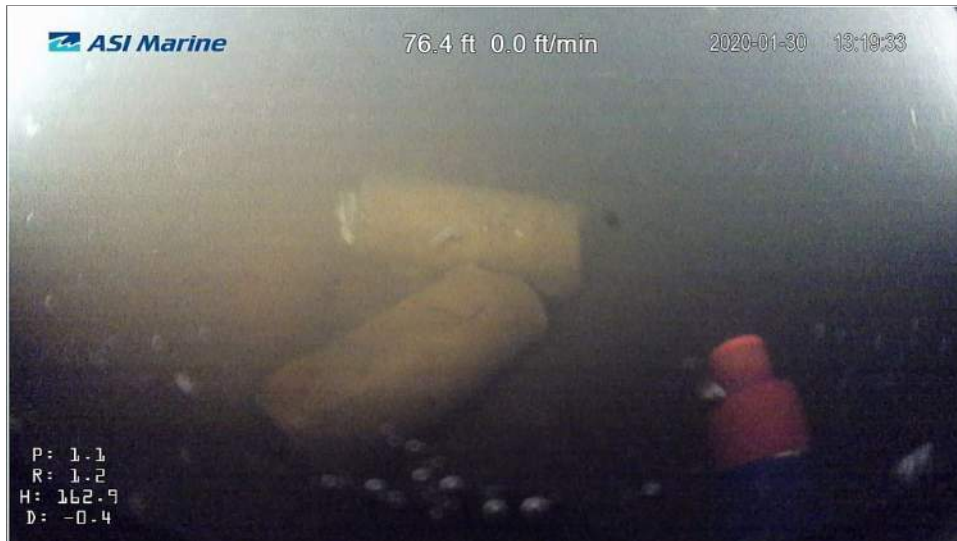
Image 4.2.1-4: Debris on invert 76 feet downstream of Access Point 1.
