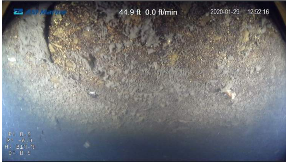
Image 4.1.1B-1: Image of crown 45 feet downstream of Manhole 3.
