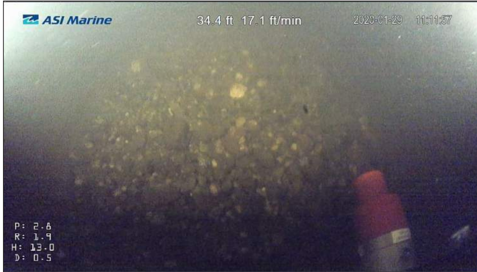
Image 4.1.1A-9: Debris on invert 35 feet upstream of Manhole 1.
