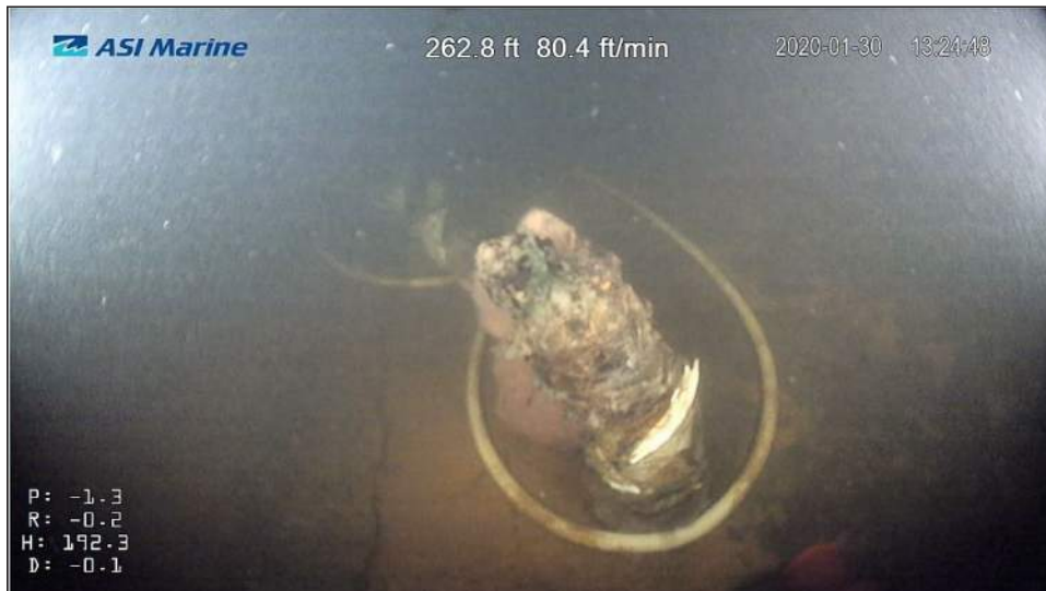
Image 4.2.1-16: Protrusion at invert 262 feet downstream of Access Point 1.
