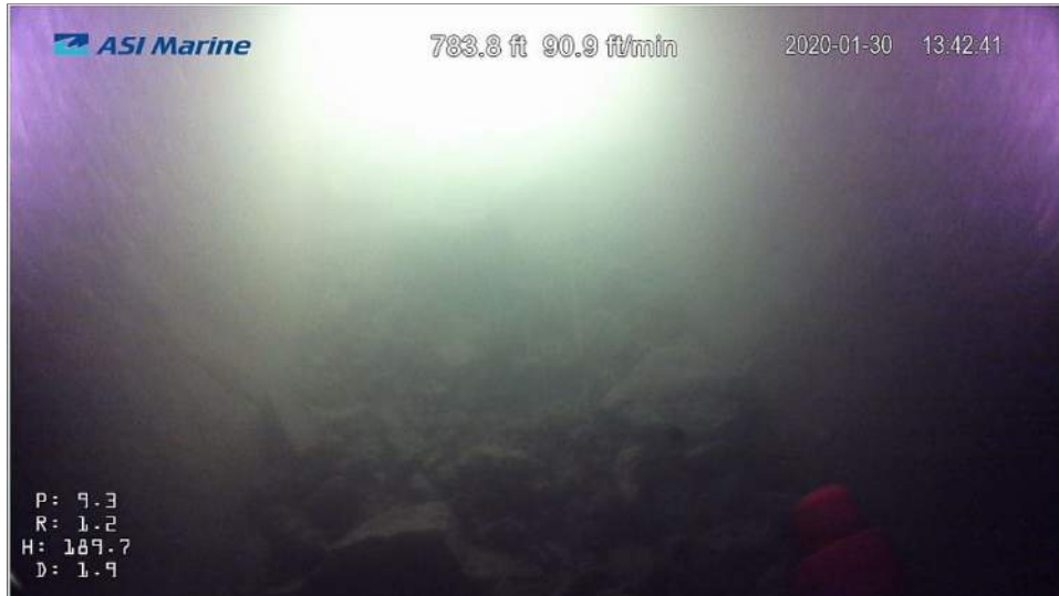
Image 4.2.1-29: Debris on invert at outfall 784 feet downstream of Access Point 1.
