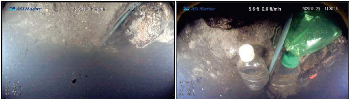
Figure 11: Exposed aggregate and line 5ft upstream (left); Exposed line at crown 5ft upstream (right)
