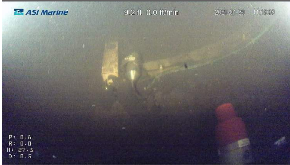
Image 4.1.1A-7: Sensor on invert 9 feet upstream of Manhole 1.
