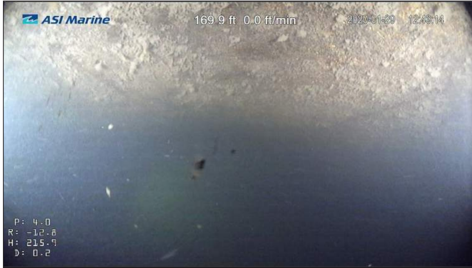
Image 4.1.1B-7: Image of crown 170 feet downstream of Manhole 3.
