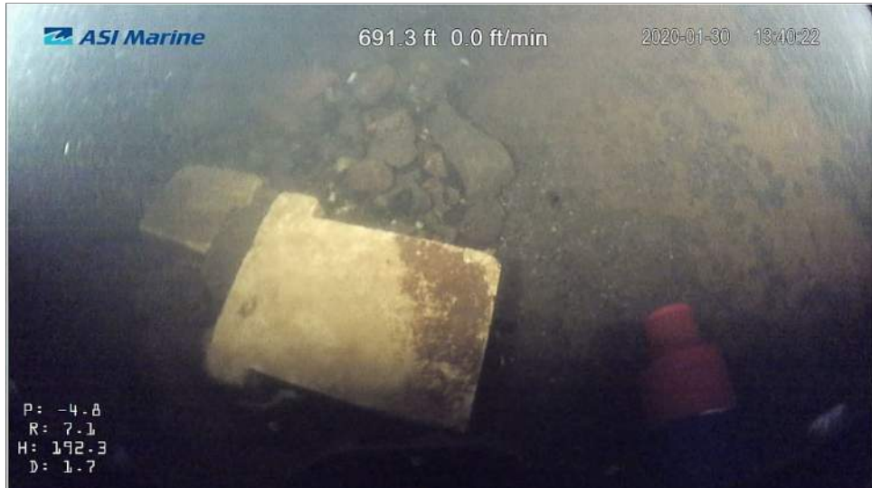
Image 4.2.1-25: Debris on invert 691 feet downstream of Access Point 1.
