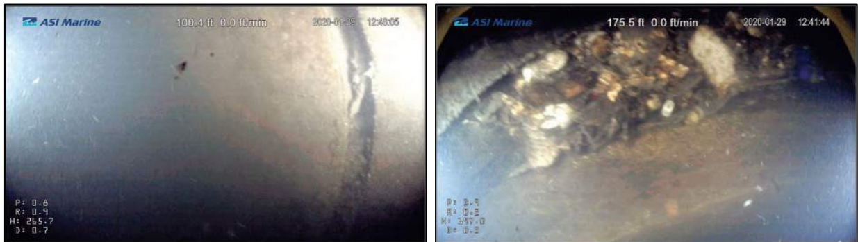
Figure 15: Image of joint at 100.4 feet (left); Image of joint at 175.5 feet (right)
