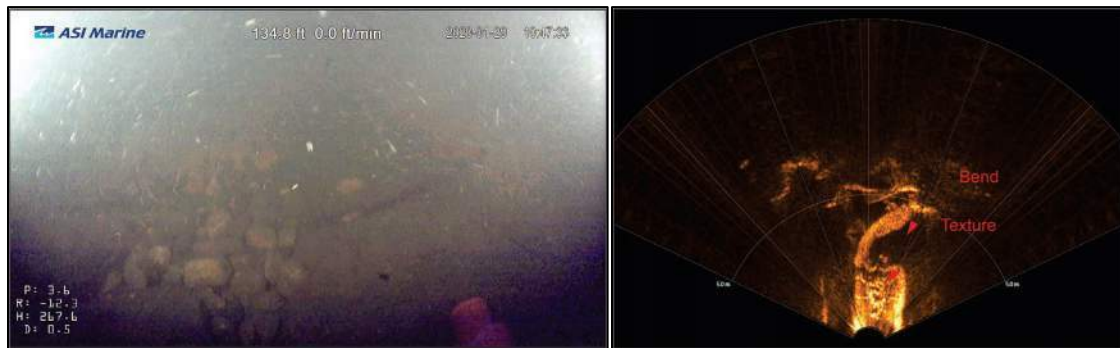
Figure 9: Image of debris on invert at 135 feet (left); Sonar image of bend at 141 feet (right)
