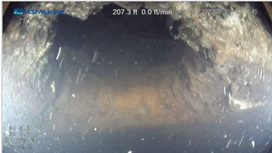
Image 4.2.1-15: Opening in crown 207 feet downstream of Access Point 1.
