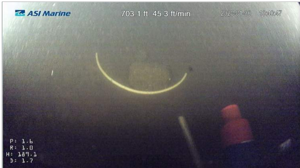
Image 4.2.1-26: Debris on invert 704 feet downstream of Access Point 1.
