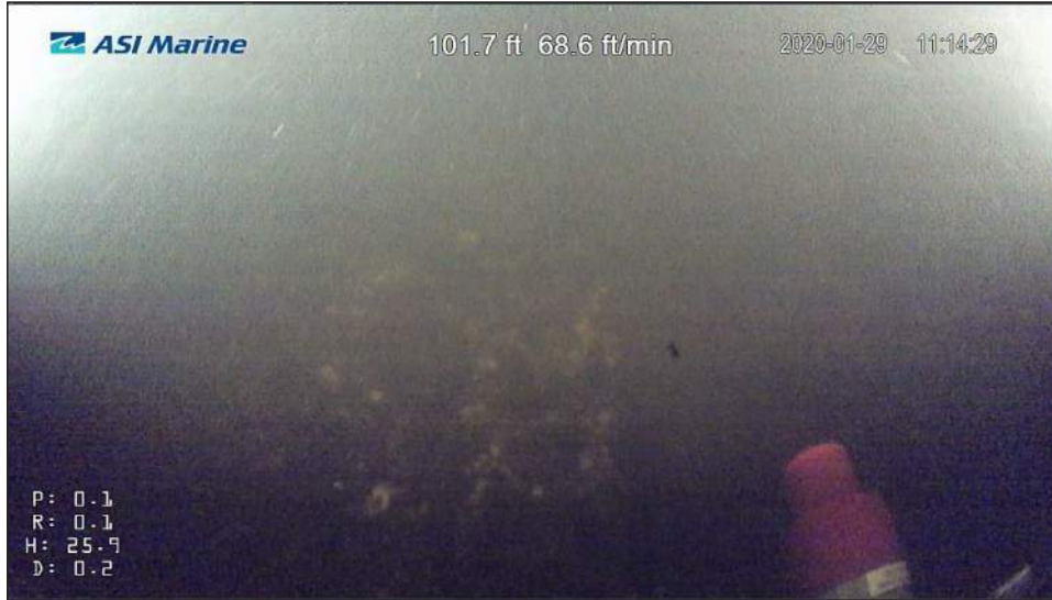
Image 4.1.1A-13: Debris on invert 103 feet upstream of Manhole 1.
