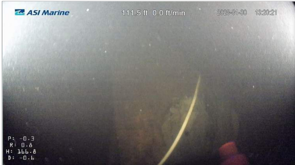
Image 4.2.1-5: Debris on invert 112 feet downstream of Access Point 1.
