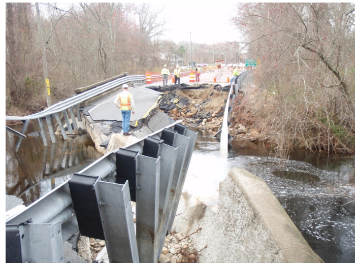
Damage to Route 184, Stonington
