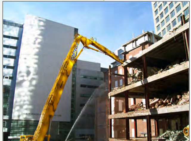
Costello Dismantling Company, Inc. provides state of the art demolition services as well as equipment removal and salvage.
