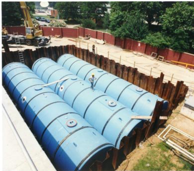
3 Underground Storage Tanks
