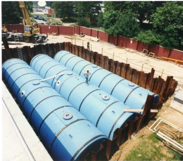
3 Underground Storage Tanks
