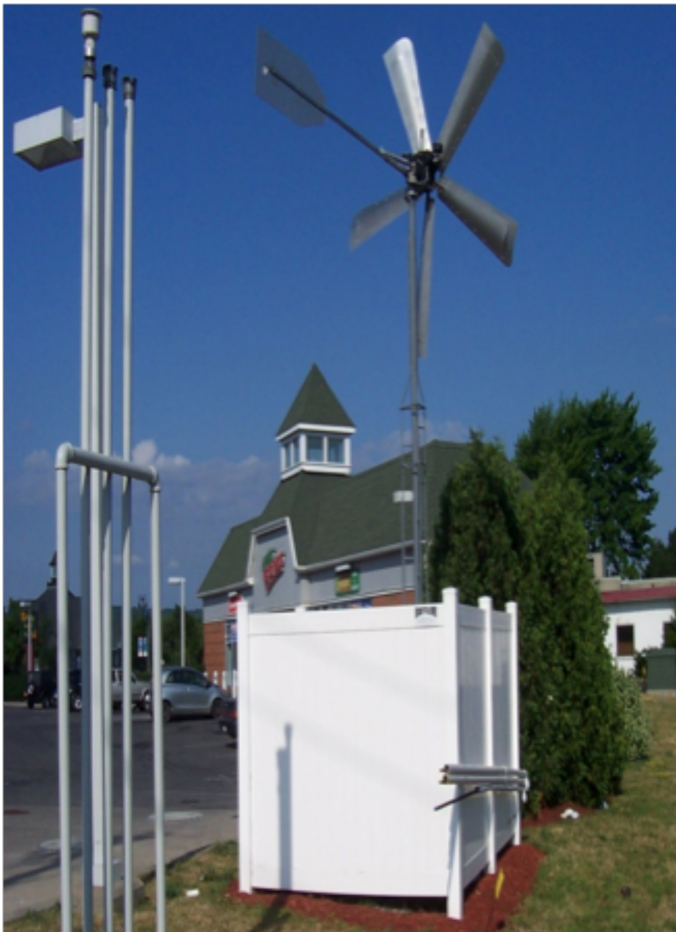
Figure 3. A wind-driven compressor operating a biosparge system to increase dissolved oxygen.
