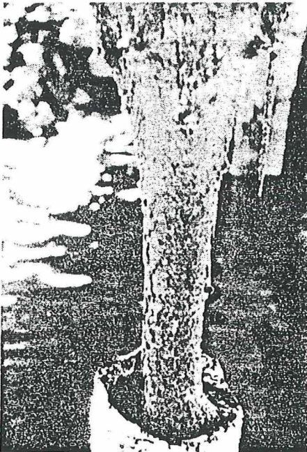
Figure 11 Crustacean borer damage - severely weakened marine piling.
