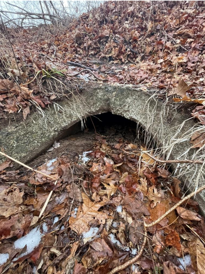
Views of clogged pipe at DEEP property to be removed by owner of 730 Forest Road.
