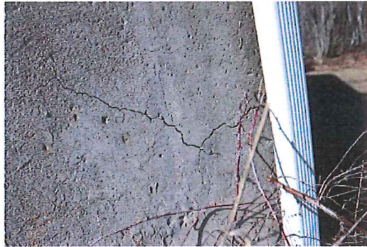
(c) map cracking
