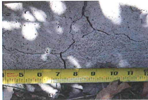
(c) wide crack opening
