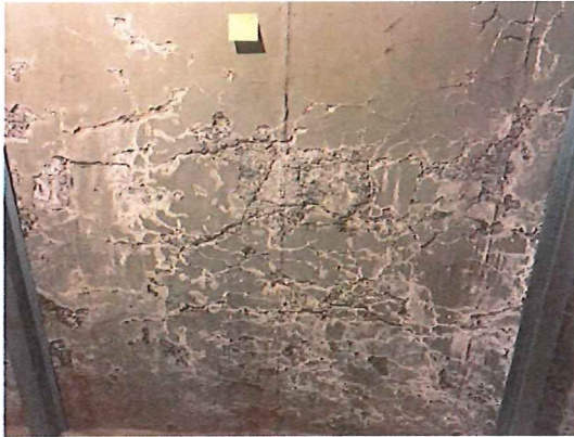
a) map cracking
