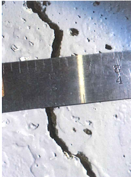
(c) wide crack opening
