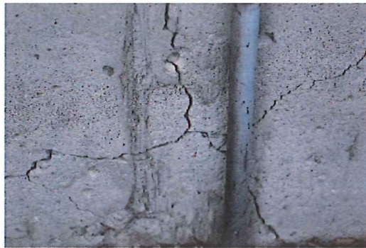
(b) map cracking
