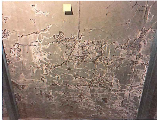
(c) map cracking
