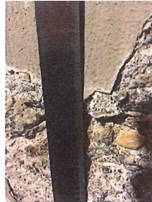
d) crack opening (>4mm)
