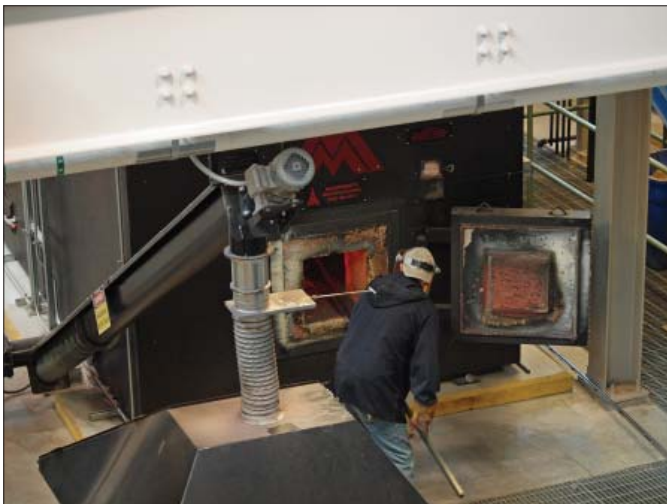
The firebox does need tending as wood chips are being burned. Here, one of the operators at the Hotchkiss School moves ash in the bottom of the firebox over towards where it can be aggregated and then removed through the use of a screw auger (left of the picture). The ash will be used as a soil amendment.
