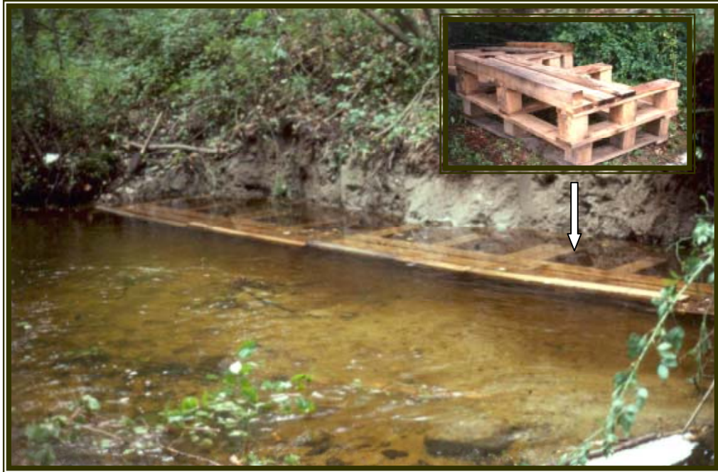
Installation of pre-fabricated LUNKER structures designed to create undercut streambank cover for fish.
