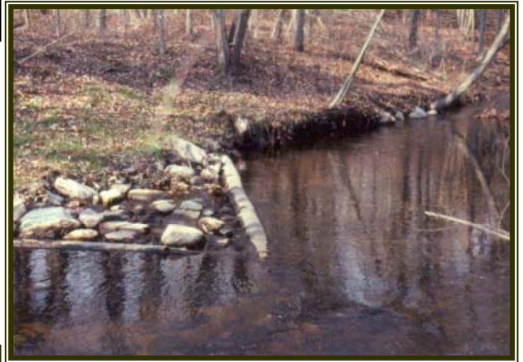
Log/rock wing deflector after completion. This habitat structure is designed to create a narrow and sinuous channel.
