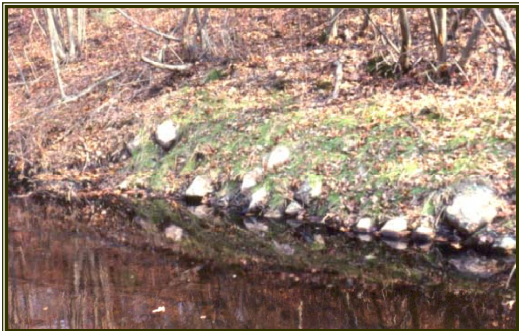
View of LUNKERS after installation. Structures have been incorporated into the streambank underneath the water surface.
