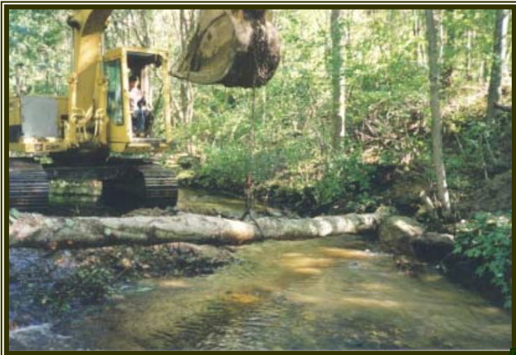
Installation of cross-log habitat structure designed to create pool habitats above and below the structure.
