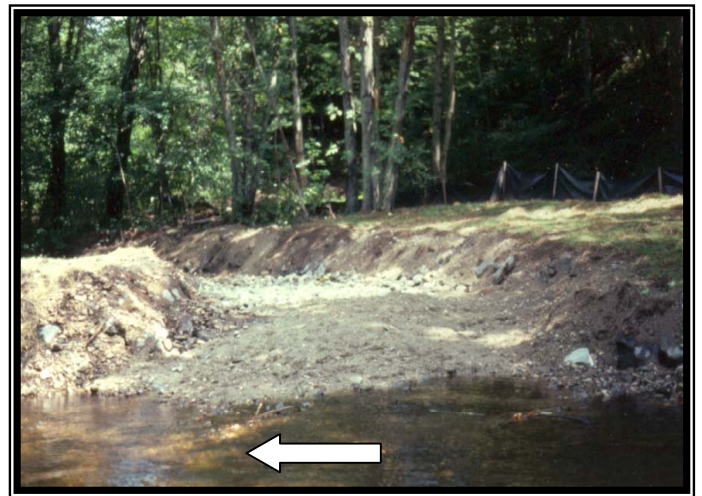
Completed channel block. The structure with its raised elevation redirects flow back to the main channel of the Moosup River.
