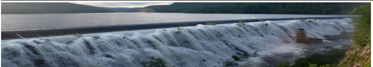
Occasionally, during periods of sustained high precipitation, water spills over the Goodwin Dam. A key function of the Colebrook River Dam (far background in photo) is to mitigate against flooding in the watershed. Photo by the Farmington River Watershed Association.
