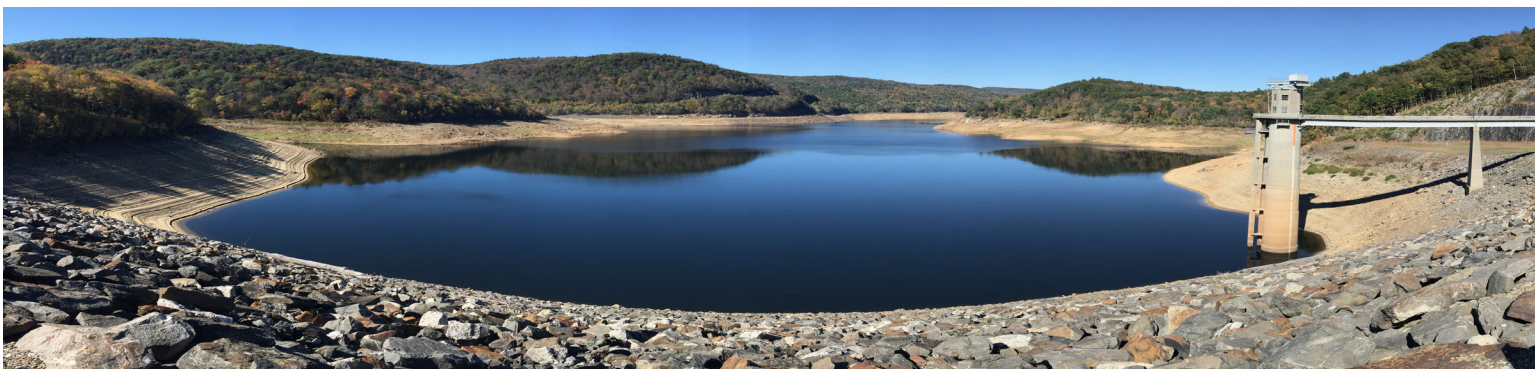
Colebrook River Lake and the control tower on October 17, 2017 when the surface elevation was 641.1 feet. Photo by the DEEP Fisheries Division
